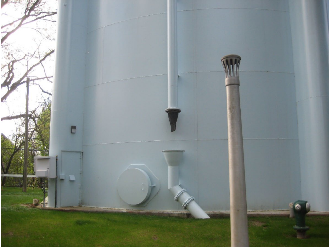
Photo 1 – SUEZ Spring Valley Standpipe – April 30, 2021
