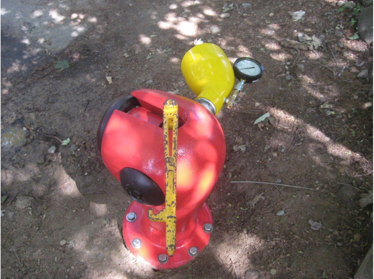
Hydrant 1-119 – Hydrant with diffuser – June 10, 2021
