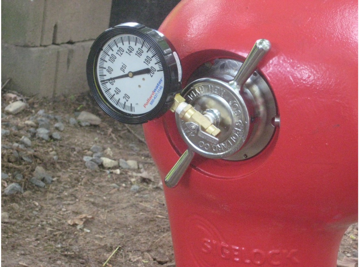
Hydrant 1-119 Installed on April 30, 2022 – Pressure Gauge Detail – June 10, 2021
