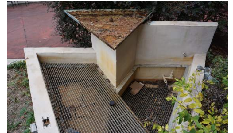
Generally the fountains are in fair to poor condition.
