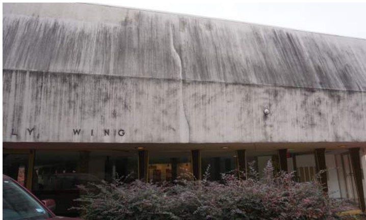
Concrete at the education wing addition is heavily soiled and cracked.
