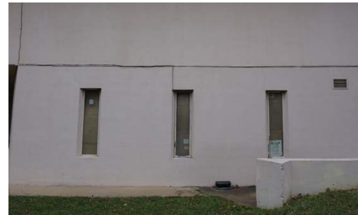
Steel frame windows at the added basement offices are in good to fair condition.
