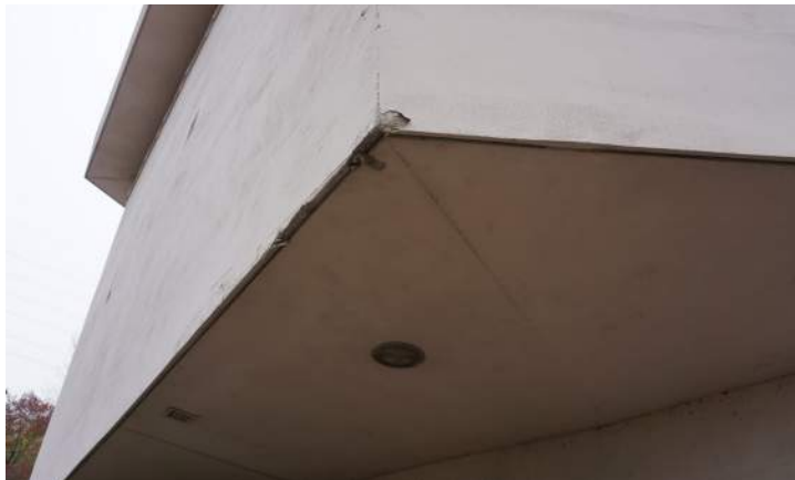
Delaminated coatings and deteriorated concrete is typical at overhang edges. Exterior lighting and mechanical vents in soffits in fair condition.
