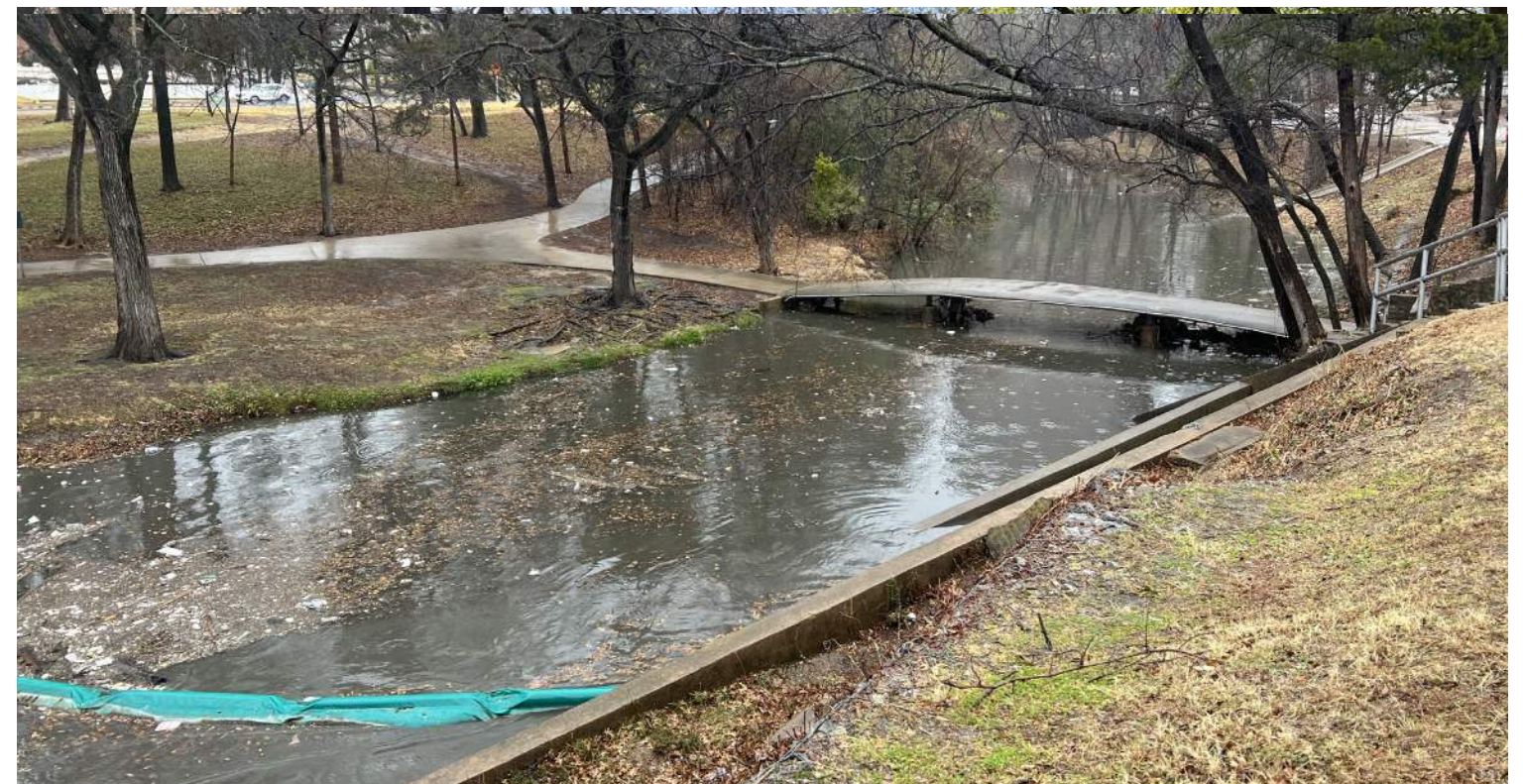
A floating silt fence installed just below the large outflow structure on site collects trash and debris from Turtle Creek. Trash flow into the creek is compounded during storm events.
