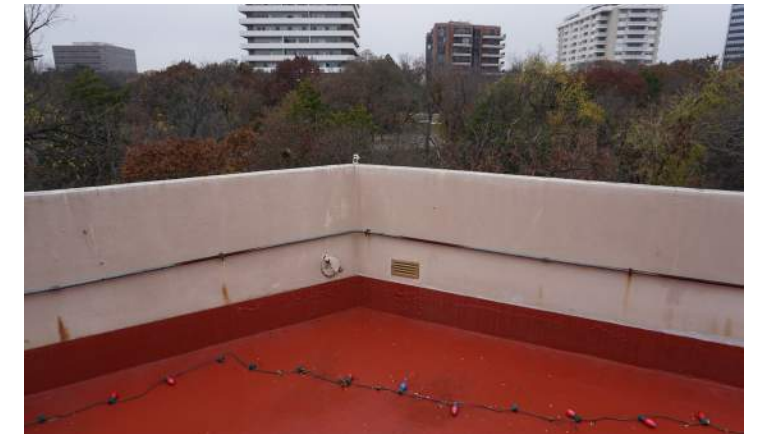
Built up roofing on terraces in fair to poor condition.
