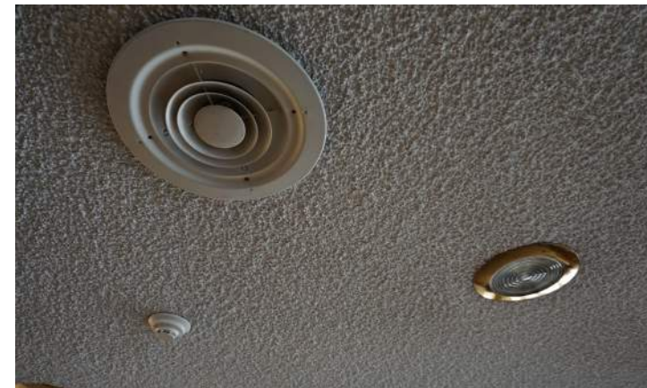
Circular flush-mount lense lighting typical of the building seen at right. MEP and life safety devices are randomly placed across lobby ceiling.
