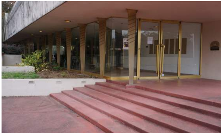
Exterior red-stained concrete steps are in poor condition.
