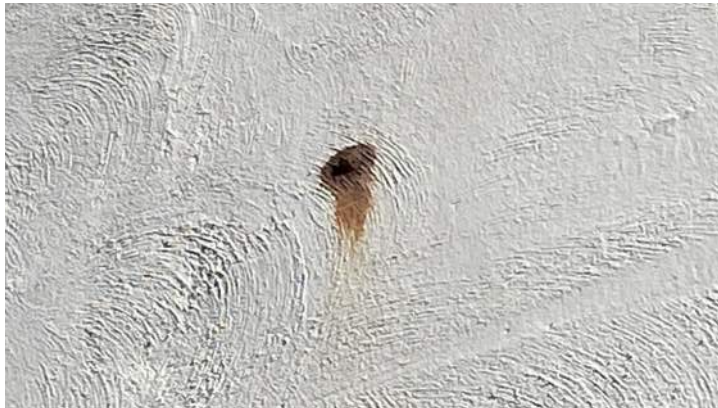
Image 7 Ferrous staining at drum exterior, viewed from roof
