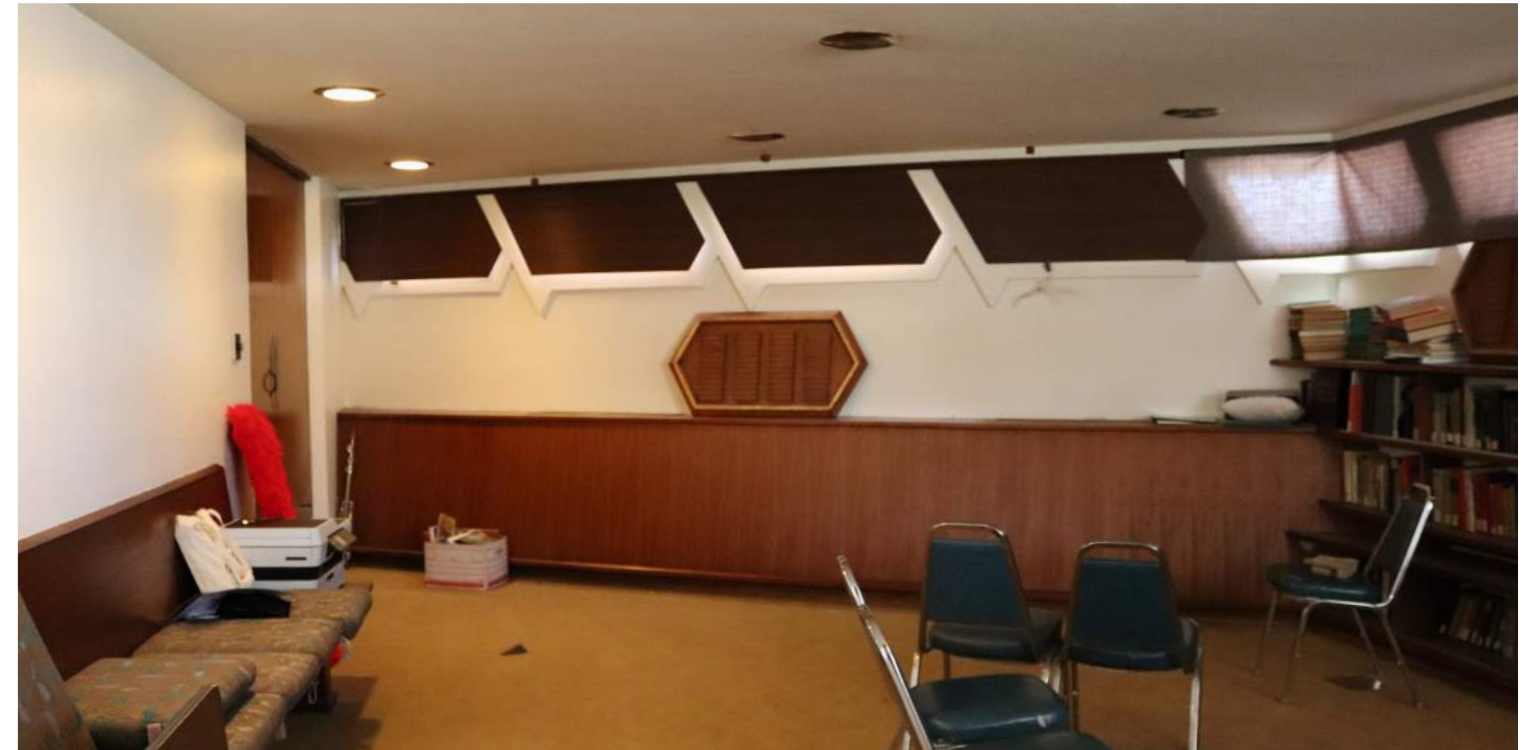
West wall of committee room lined with mechanical enclosure with typical clerestory windows above.
