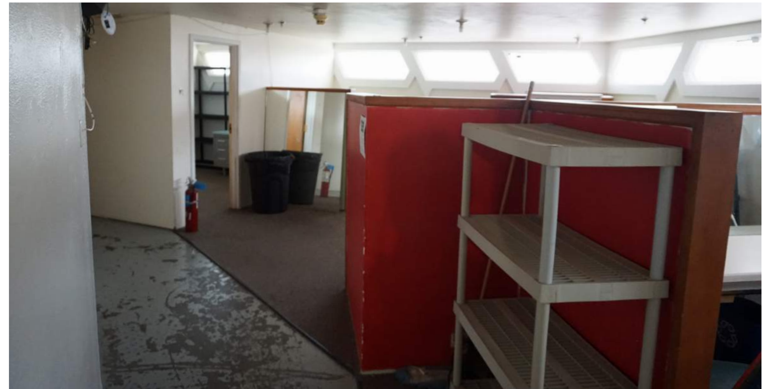
View of open dressing room at the plenum level.
