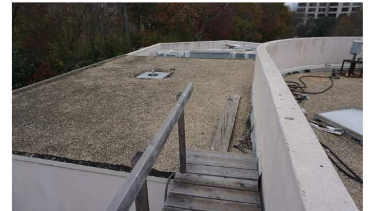
Flat roofing is at the end of its serviceable life.
