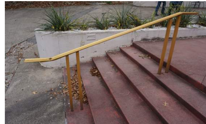
The non-original handrails are unstable.
