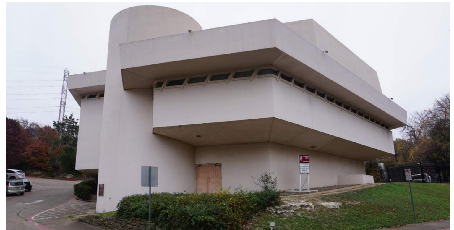
Typical existing conditions of coated concrete facades, soffits, clerestory windows, and exterior doors are visible on the northwest facade.
