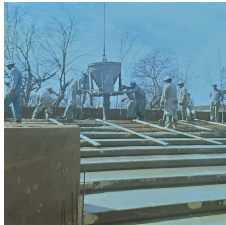
Images 16, 17 Construction photos of the house floor showing reinforcement in the slab and initial slab pour. Courtesy of Avery Library.
