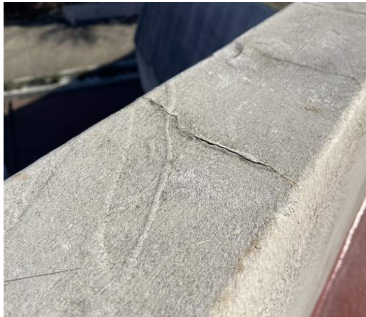
Image 8 Cracking in exterior parapet
