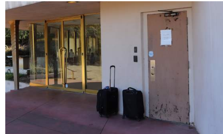
Exterior hollow metal doors are in fair condition with failed paint.
