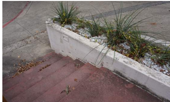
Concrete retaining walls are in fair condition with failing paint and areas of delaminated concrete.
