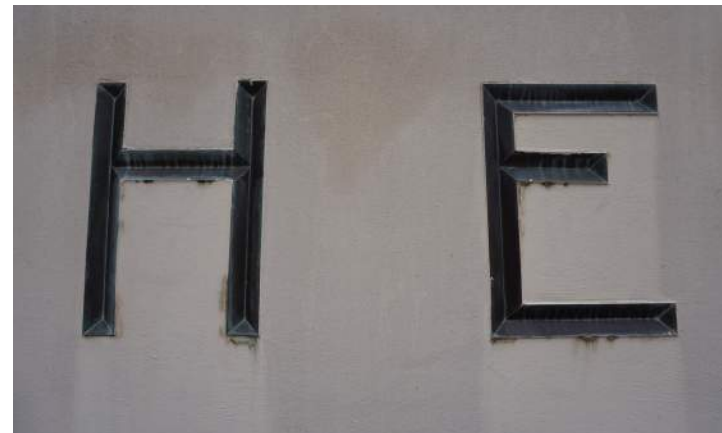
Bronze lettering on the building sign is in good condition, though is causing some soiling to the surrounding concrete.
