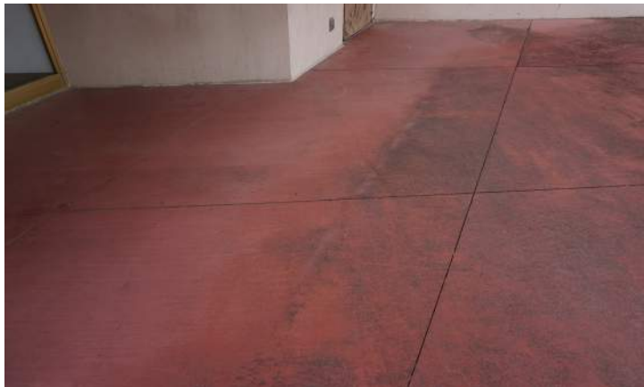
Exterior red-stained concrete pavers are soiled, cracked, and previously repaired.
