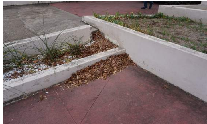
Generally exterior entry elements are soiled.
