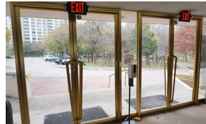
New glass doors at south entry are replicated from the original doors.
