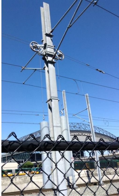
Figure 4. Auto-tension Weights for Overhead Catenary Systems. The self-adjusting cylindrical weights are hanging on either side of the support pole. Photo source: Sound Transit.
