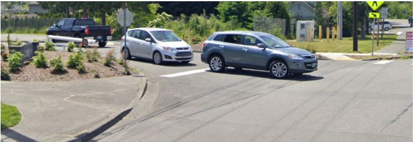
Paving joint – either the driveway crossing or the Lundeen Parkway crossing was affected, only one ramp replaced
