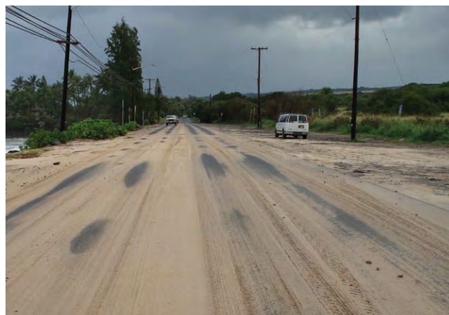
While it provides access to 13,000 cars per day (Hawai'i Department of Transportation-Highways Division), Kamehameha Highway at Laniākea is threatened by chronic erosion and frequently floods during large swell events. Photo: Dolan Eversole
