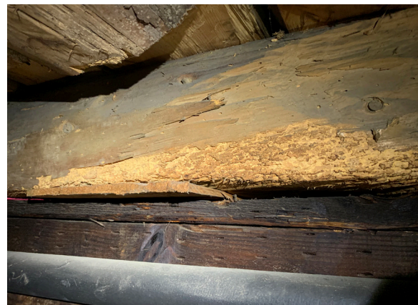
Figure 1-357. Insect damage visible on a first floor dropped log beam (CBB, 08/26/2021)
