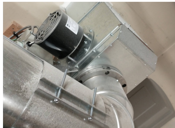
Figure 1-372. Boiler Flue Draft Inducer (JSW 8/24/2021)
