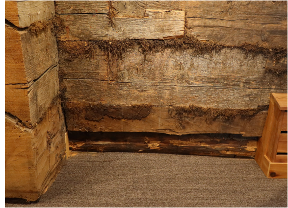
Figure 1-289. Previously replaced log at north wall of Museum II 104. (EAV, 08/24/2021)
