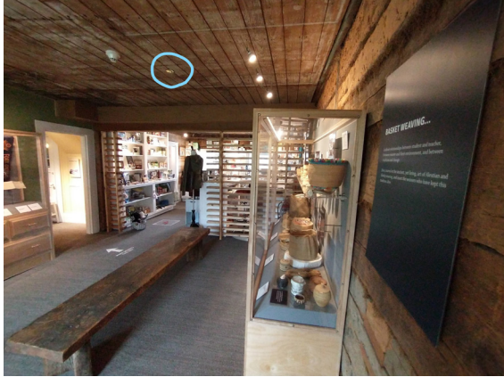
Figure 1-397. Exhibit Area Fire Sprinkler Heads (JSW 8/24/2021)
