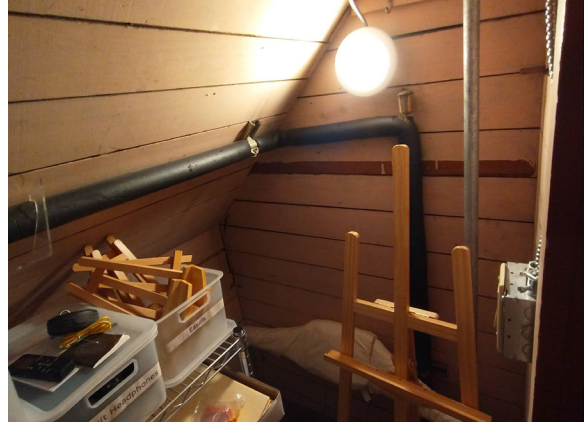
Figure 1-400. Second Level Exposed Fire Sprinkler Head and Pipe (JSW 8/24/2021)
