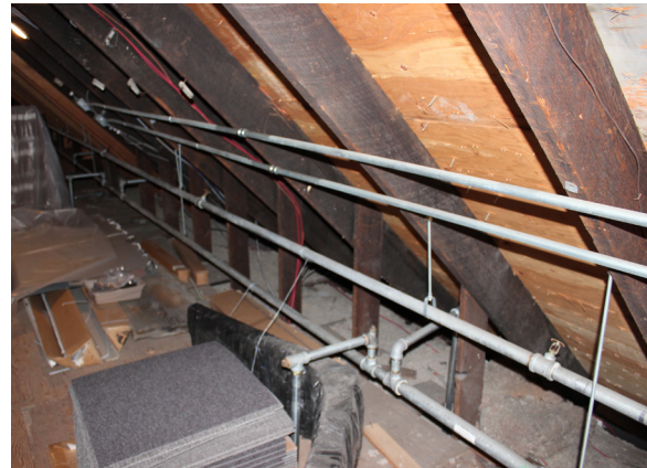
Figure 1-364. Verticals hanging the attic floor joists from the rafters (as seen behind the piping). (CBB, 08/26/2021)
