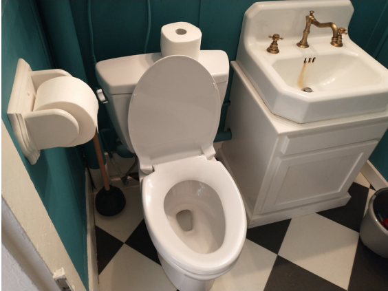
Figure 1-391. First Level Restroom Fixtures (JSW 8/24/2021)
