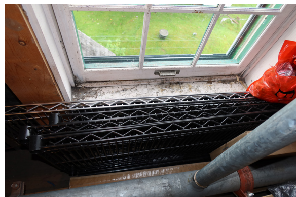
Figure 1-197. Debris and water damage at sill of Window 34. (EAV, 08/24/2021)
