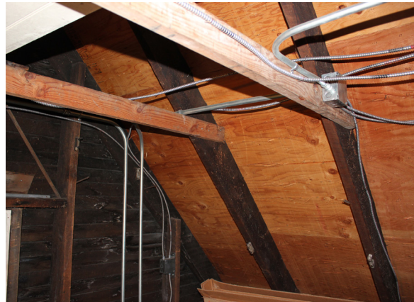
Figure 1-362. Roof framing of the Magazin. Note the rafters, collar ties, and plywood sheathing (CBB, 08/26/2021)
