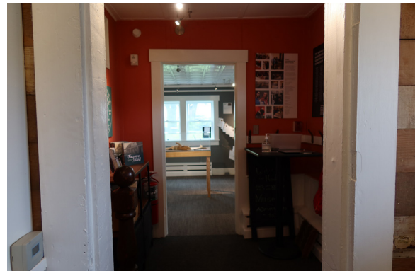
Figure 1-241. Gouged and painted trim at CO 101. Note also mark at right from previous door hinge, painted over. (EAV, 08/24/2021)
