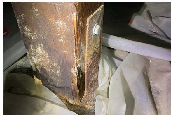
Figure 1-360. Deteriorating base of first floor post in the crawlspace. Note the corrosion of the steel angle that was intended to connect the post to the foundation (CBB, 08/25/2021)
