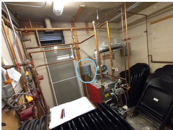
Figure 1-373. Poorly Supported Expansion Tank (JSW 8/24/2021)
