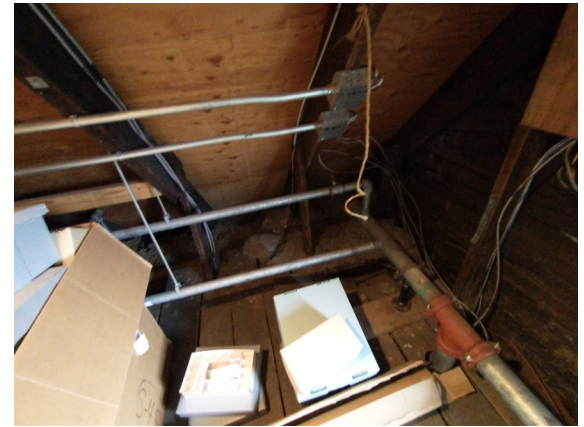
Figure 1-401. Attic Fire Sprinkler Heads and Piping (JSW 8/24/2021)
