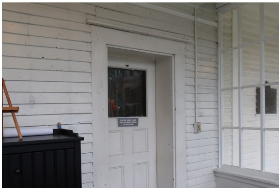
Figure 1-291. Scratched paint at north wall of Sun Porch 103. (EAV, 08/24/2021)
