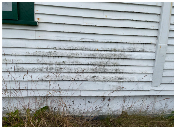
Figure 1-158. Deteriorated siding on the north facade, below the missing downspout. (KAC, 08/24/2021)
