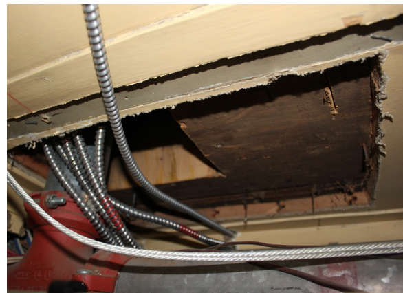
Figure 1-352. Second floor beam of the Magazin on the east half of the structure. Note the large hole cut in the beam to allow the piping to pass up to the second floor (CBB, 08/26/2021)
