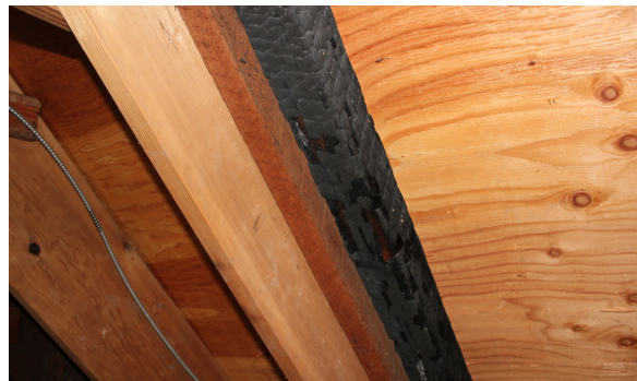
Figure 1-363. Charred 4x4 rafter with sisters (CBB, 08/26/2021)
