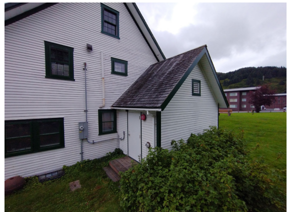
Figure 1-382. First Level Restroom Exhaust and Vent Out Of Building (JSW 8/24/2021)
