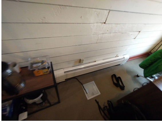
Figure 1-377. Second Level Baseboard Radiator (JSW 8/24/2021)
