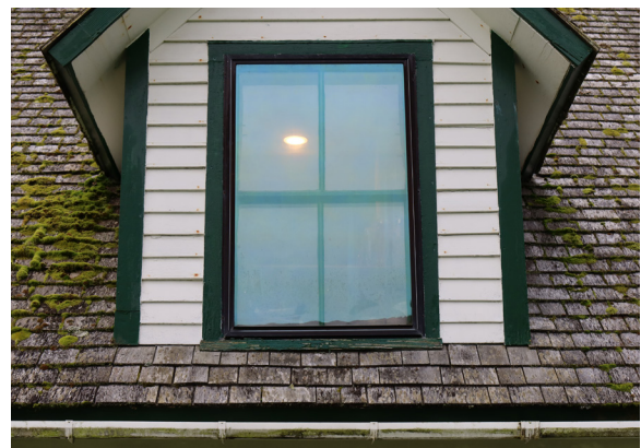
Figure 1-163. Deteriorated sill at Window 30, Type C. (EAV, 08/24/2021)
