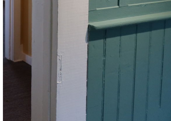
Figure 1-293. Scratched finishes with thickly applied paint in Kitchen 108. (EAV, 08/24/2021)
