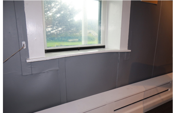
Figure 1-296. Warped sill and finishes at Window 01 in Museum IV 112. (EAV, 08/24/2021)
