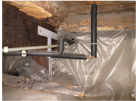
Figure 1-376. Hydronic Piping In The Crawlspace (JSW 8/24/2021)
