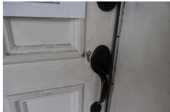
Figure 1-205. Worn and missing paint near hardware of Door 100, exterior. (EAV, 08/24/2021)
