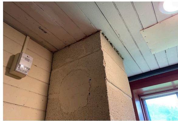
Figure 1-328. Patched ceiling and abandoned chimney in Stair Hall 200. (KAC, 08/24/2021)
