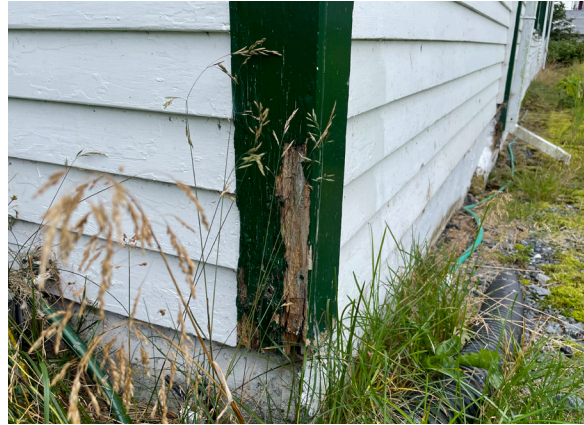
Figure 1-159. Deteriorated edge trim at northeast corner of the building. (KAC, 08/24/2021)
