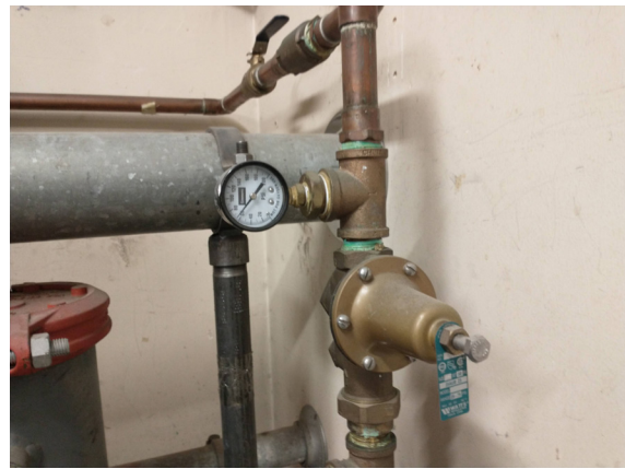
Figure 1-384. Domestic Water PRV (JSW 8/24/2021)
