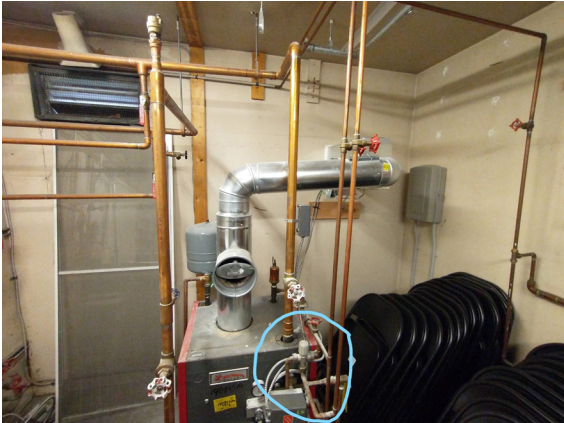
Figure 1-389. Domestic Hot Water Mixing Valve (JSW 8/24/2021)
