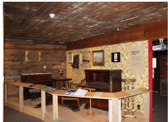
Figure 1-350. Dropped beam supporting the second floor visible at the dividing wall in Museum I (102) (CBB, 08/25/2021)
