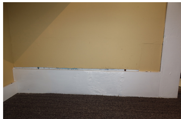
Figure 1-295. Worn plywood and wall base at north wall of Museum III 111. (EAV, 08/24/2021)
