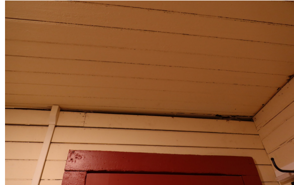
Figure 1-335. Gap at the top of the south wall of Staff Restroom 207. (EAV, 08/24/2021)
