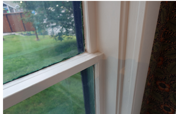
Figure 1-193. Window 15, interior. Note visible paint on glazing and sashes painted shut. (EAV, 08/24/2021)
