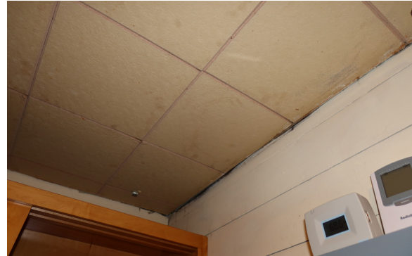
Figure 1-330. Ceiling tiles and wall boards at northeast corner of Collections II 202. (EAV, 08/24/2021)
