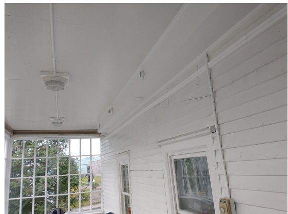
Figure 1-396. Fire Sprinkler Heads in Porch (JSW 8/24/2021)
