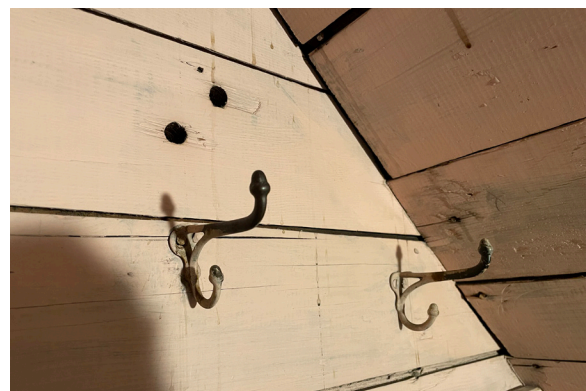
Figure 1-332. Scratched paint and holes from previous attachments in Storage 205A. (EAV, 08/24/2021)
