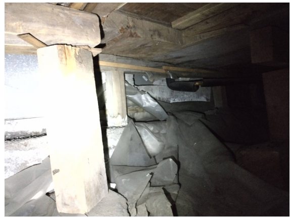
Figure 1-387. Damaged Cast-Iron Waste Pipe (JSW 8/24/2021)
