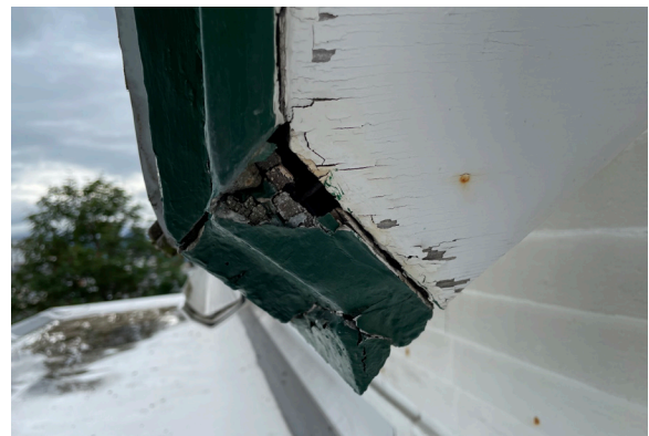
Figure 1-142. Deterioration at the end of wood fascia and trim. (KAC, 08/24/2021)
