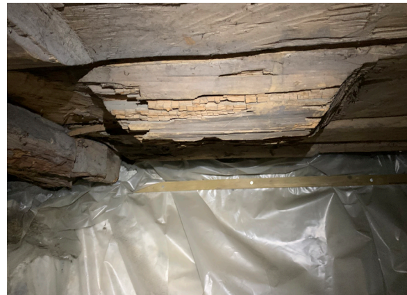
Figure 1-356. Deterioration visible on a first floor deck board (CBB, 08/25/2021)
