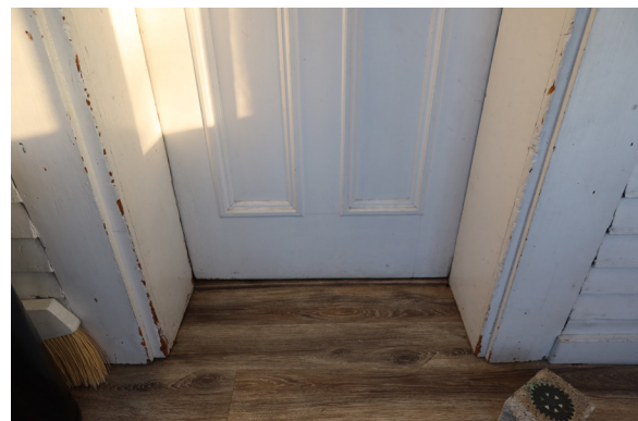
Figure 1-242. Missing paint at trim on Sun Porch 103 side of Door 103A. (EAV, 08/24/2021)
