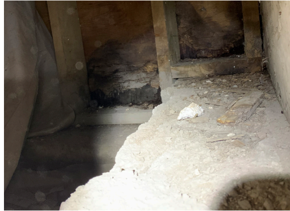
Figure 1-346. Interior face of the north wood stud foundation wall of the Alcove. Note the water staining and deterioration at the base of the wall (CBB, 08/25/2021)
