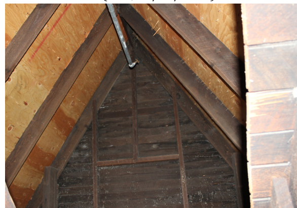
Figure 1-366. Roof framing of the gable dormer on the south facet of the roof. (CBB, 08/26/2021)
