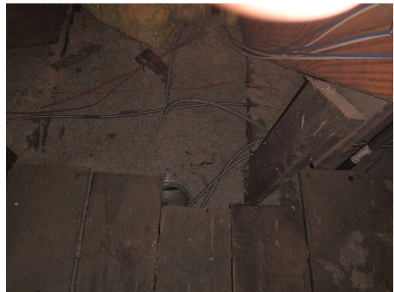
Figure 1-381. Second Level Restroom Exhaust Into Attic (JSW 8/24/2021)
