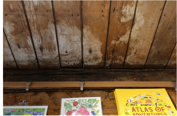
Figure 1-288. Stained ceiling boards in Gift Shop 101. (EAV, 08/24/2021)
