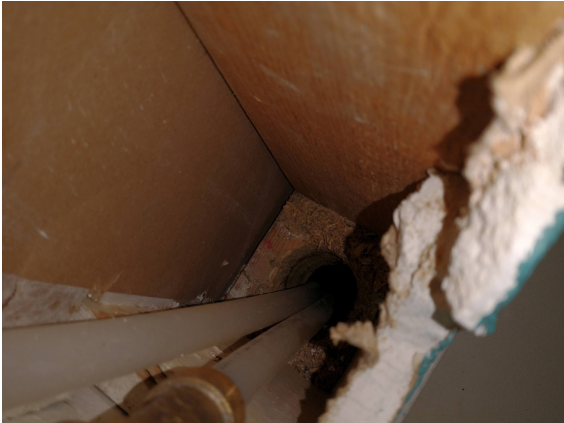
Figure 1-390. PEX Piping Down in Restroom Wall to Crawlspace (JSW 8/24/2021)
