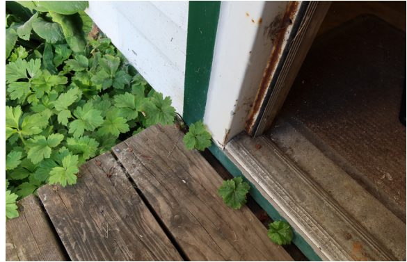
Figure 1-207. Rust at frame of Door 110. (EAV, 08/24/2021)
