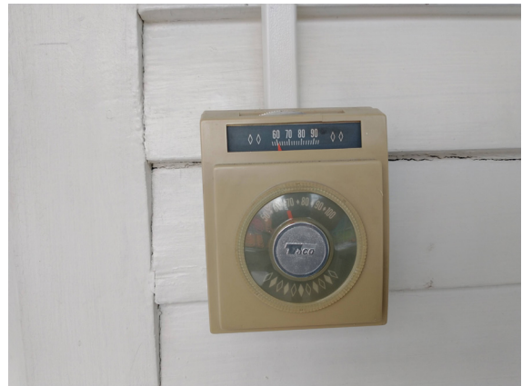
Figure 1-375. Hydronic Thermostat (JSW 8/24/2021)
