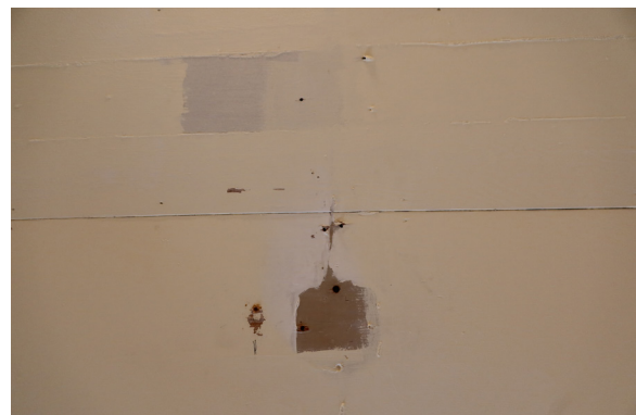
Figure 1-334. Missing paint at ceiling of Office II 206. (EAV, 08/24/2021)
