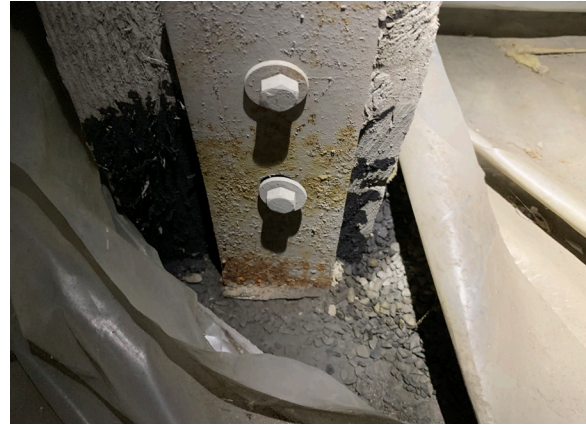
Figure 1-348. Deteriorating and disintegrating concrete at the interior isolated concrete footings (CBB, 08/25/2021)
