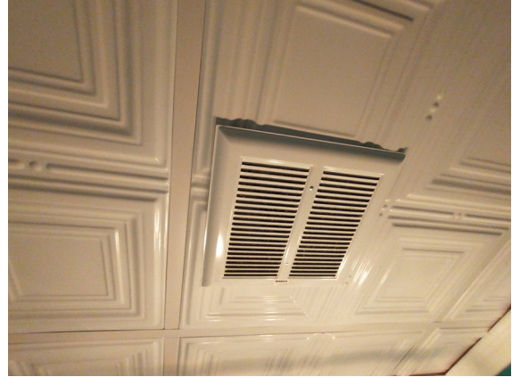
Figure 1-380. Exhaust Fan in First Floor Restroom (JSW 8/24/2021)
