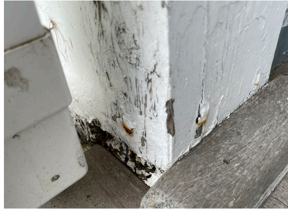
Figure 1-150. Deteriorated column base. (KAC, 08/24/2021)
