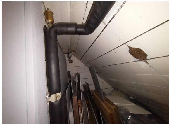
Figure 1-378. Hydronic Piping on The Second Level (JSW 8/24/2021)
