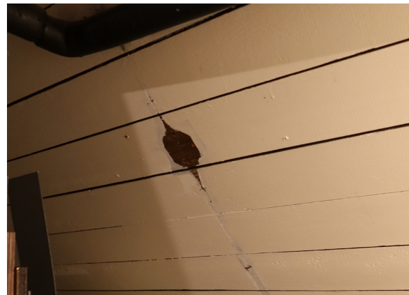
Figure 1-329. Missing paint from previous attachments in Eunice 201A. (EAV, 08/24/2021)
