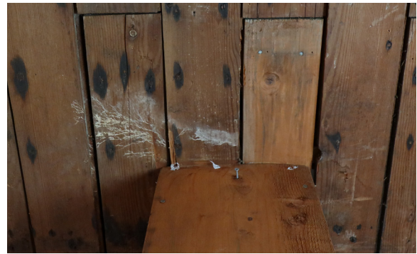
Figure 1-286. Growth on ceiling boards near the plumbing chase in Museum I 102. (EAV, 08/24/2021)
