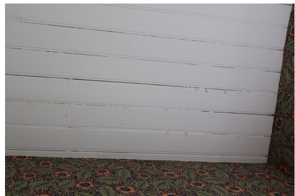
Figure 1-287. Water staining at alcove ceiling in Museum I 102. (EAV, 08/24/2021)
