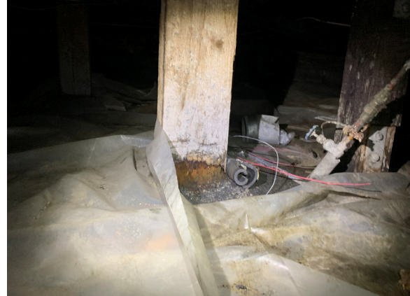
Figure 1-355. Deteriorating base of a post supporting the first floor of the Magazin (CBB, 08/25/2021)
