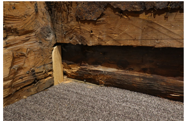
Figure 1-292. Previously replaced log at north wall of Museum II 104. (EAV, 08/24/2021)
