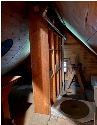
Figure 1-306. Facing east in Mechanical Attic 201B. (EAV, 08/24/2021)
