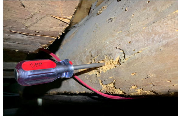
Figure 1-358. Insect damage visible on a first floor dropped log beam as exhibited by the penetration of the awl into the member (CBB, 08/26/2021)
