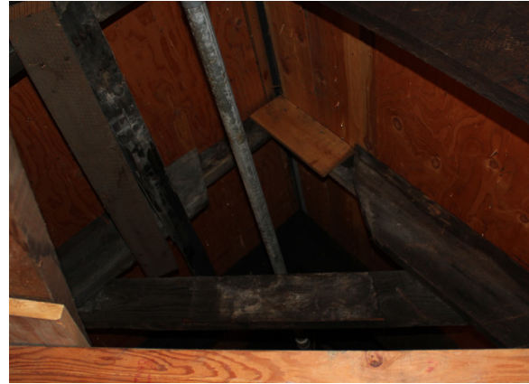
Figure 1-367. In one location, the rafters have been cutback from the peak of the roof and sistered (CBB, 08/26/2021)
