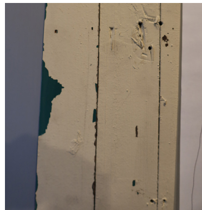
Figure 1-336. Thickly applied and missing paint at wall boards in Director's Office 208. (EAV, 08/24/2021)
