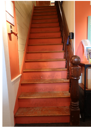
Figure 1-282. Facing north at the bottom of the stairs to the second floor. (EAV, 08/24/2021)
