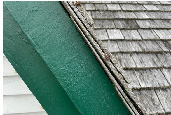
Figure 1-136. Lapped cedar shingles viewed at gable end of dormer. Visible here is the historic fascia profile. (KAC, 08/24/2021)
