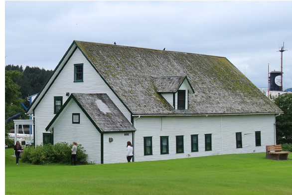
Figure 1-138. Magazin viewed from northeast. Note the small dormer, center, and the patch of replaced shingles at the addition roof, image left. (EAV, 08/24/2021)
