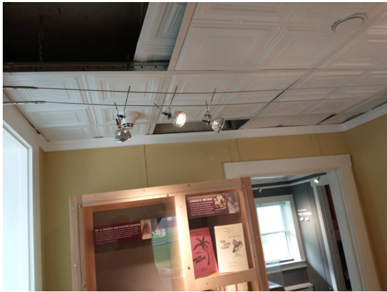
Figure 1-398. Tin Ceiling Fire Sprinkler Heads (JSW 8/24/2021)
