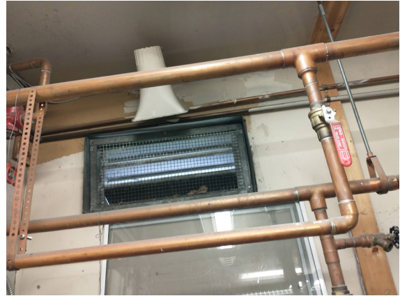
Figure 1-374. Combustion Air Louver (JSW 8/24/2021)
