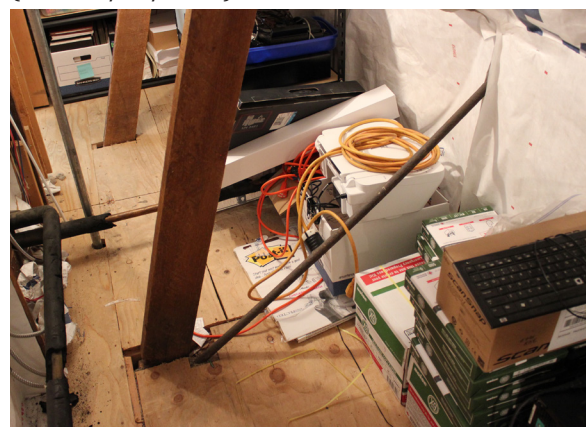
Figure 1-365. Dimensional lumber and steel rod diagonals of the roof framing visible in the storage areas along the eaves of the north and south elevations (CBB, 08/26/2021)
