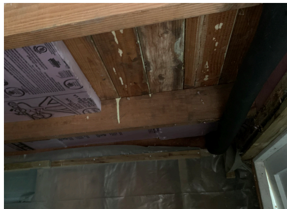
Figure 1-347. Interior face of the south wood stud foundation wall of the Sun Porch as seen through the plastic sheeting (CBB, 08/24/2021)
