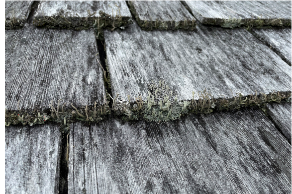
Figure 1-141. Significant bio-growth at cedar shingles. (KAC, 08/24/2021)
