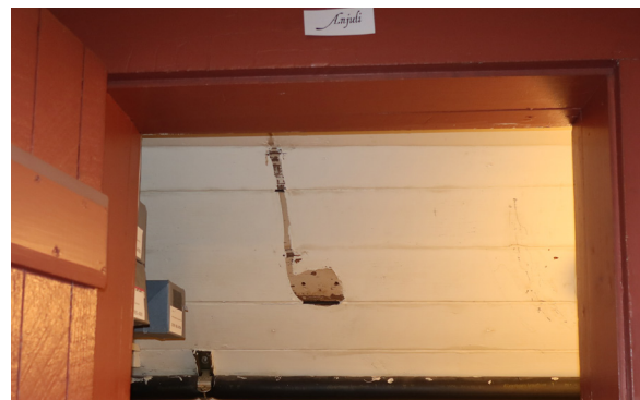
Figure 1-331. Missing paint from previous attachments in Anjuli 202A. (EAV, 08/24/2021)
