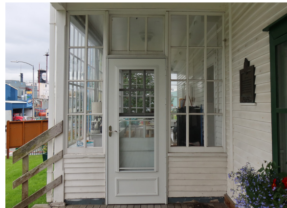
Figure 1-170. Window 07 at right and Window 08 at left, Type F. Door 103B at center. (EAV, 08/24/2021)
