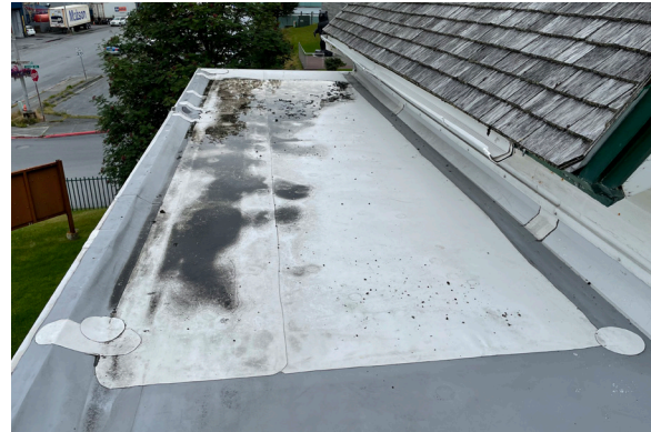
Figure 1-144. Ponding water at the west end of the porch roof. Recent patches visible in white. (KAC, 08/24/2021)
