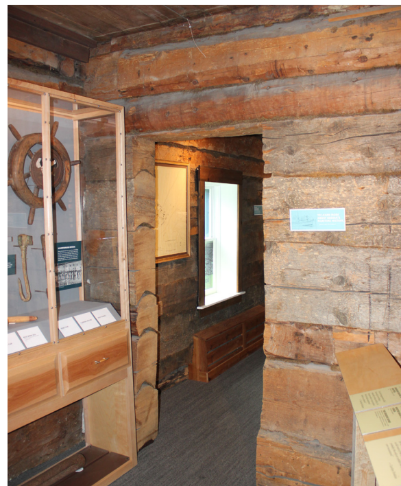
Figure 1-369. Opening created in the interior log wall after the original construction (CBB, 08/25/2021)
