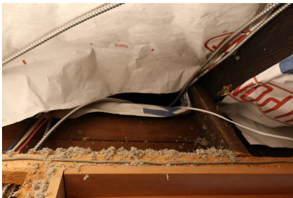
Figure 1-333. Insulation from above falling into Storage 205B. (EAV, 08/24/2021)
