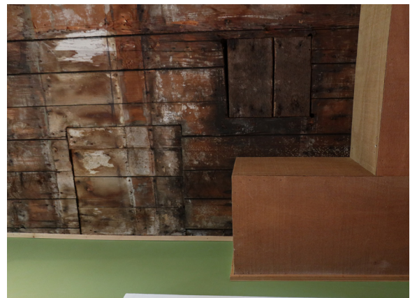
Figure 1-290. Patched and stained ceiling boards in Museum II 104. (EAV, 08/24/2021)
