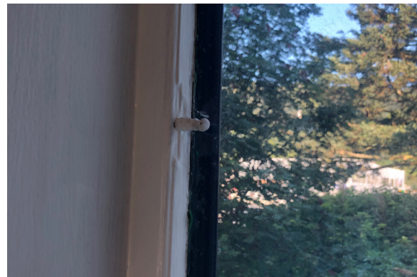
Figure 1-63. Windows are painted shut. (BM, 08/24/2021)
