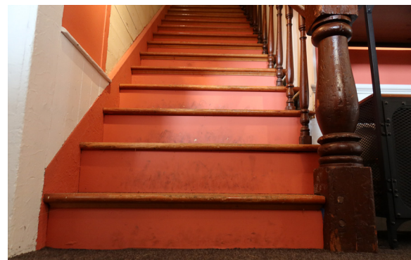
Figure 1-284. Facing north at the bottom of the stairs to the second floor. Note missing trim at replaced risers. (EAV, 08/24/2021)
