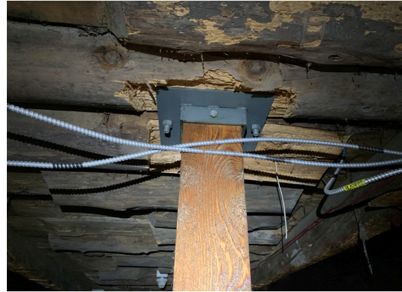
Figure 1-351. Timber post supporting dropped second floor glulam beam added in the 1980s as seen from the crawlspace (CBB, 08/24/2021)
