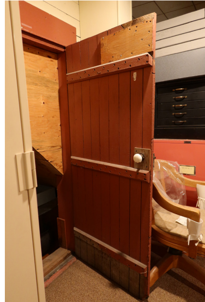
Figure 1-243. Mechanical Attic 201B side of Door 201B. (EAV, 08/24/2021)
