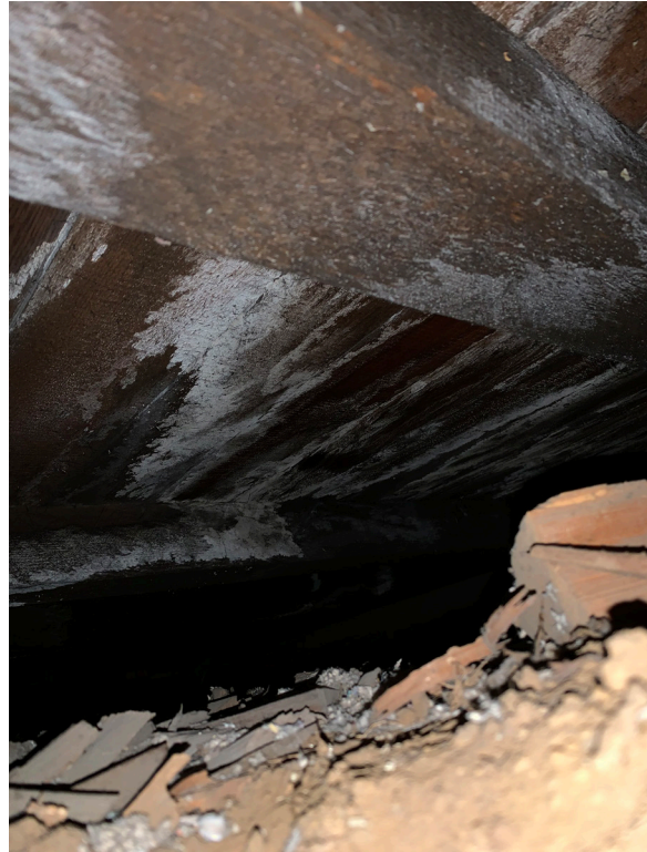
Figure 1-353. Second floor framing cavity of the Magazin on the east half of the structure. Note the 4x4 joists at the top of the cavity and the mold or water staining visible on the wood members (CBB, 08/25/2021)
