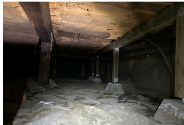
Figure 1-359. Added dropped beam, posts, and footings to support the previously unsupported floor framing at the south elevation of the structure near the front door (CBB, 08/24/2021)
