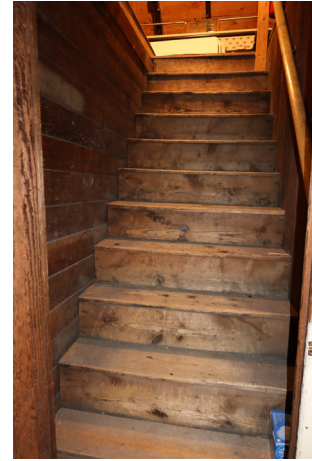
Figure 1-327. Facing north at the bottom of the stairs to the attic. (EAV, 08/24/2021)
