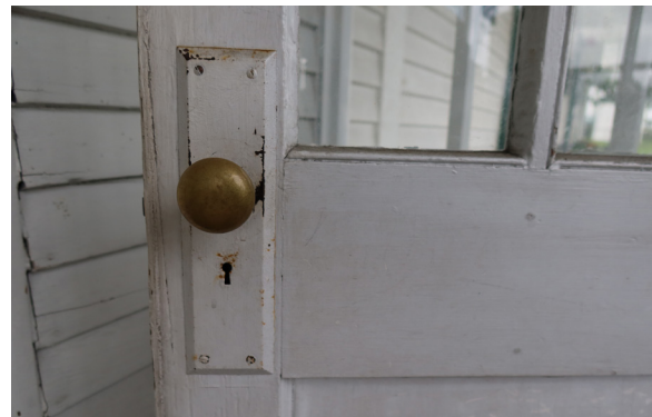
Figure 1-206. Missing and worn paint on and near hardware of Door 103B, exterior. (EAV, 08/24/2021)
