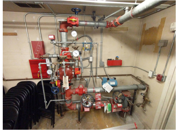
Figure 1-394. Fire Suppression Equipment and Water Entry (JSW 8/24/2021)
