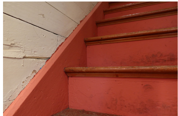
Figure 1-297. Scuffed risers and thick paint at the stairs. (EAV, 08/24/2021)
