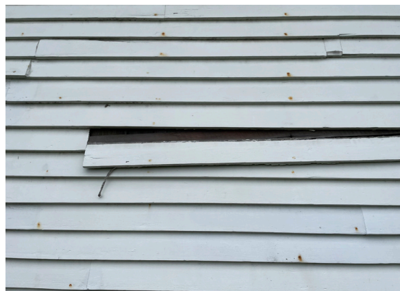
Figure 1-157. Loose siding board on the north facade. (KAC, 08/24/2021)
