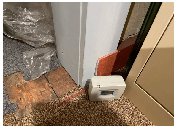
Figure 1-305. Missing carpet reveals wood floor boards at CO 201A. (KAC, 08/24/2021)
