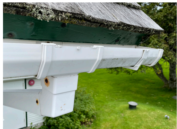
Figure 1-143. Shingles overhang the undersized gutters. (KAC, 08/24/2021)
