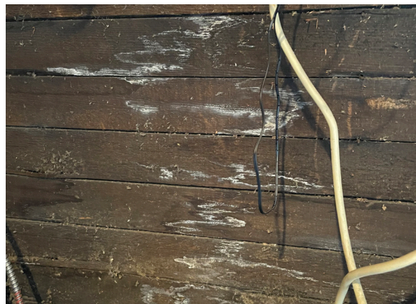
Figure 1-343. Smoke stain and efflorescence on exposed sheathing at the east wall of Attic I 300. (EAV, 08/24/2021)
