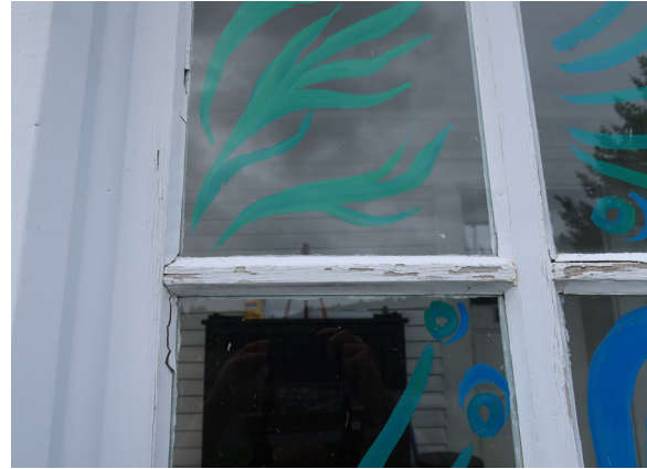
Figure 1-192. Missing paint and cracked glazing putty at Window 09. (EAV, 08/24/2021)
