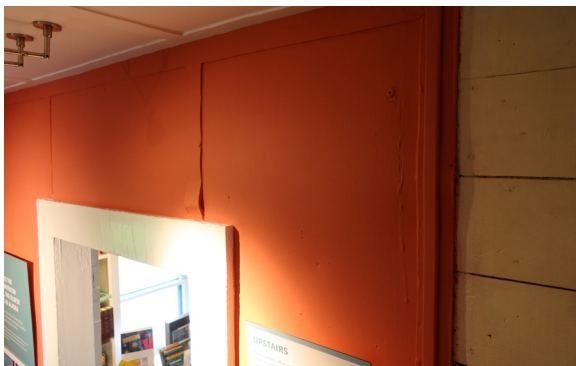
Figure 1-285. Warped gypsum wall board and battens in Entry 100. (EAV, 08/24/2021)
