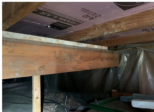
Figure 1-354. Joists and dropped beams of the first floor of the Sun Porch (CBB, 08/24/2021)
