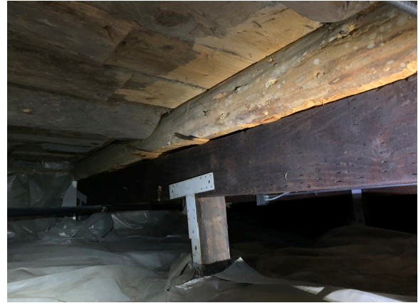
Figure 1-349. First floor framing of the Magazin west of the interior log wall. Note the deck boards framing to a dropped log beam that is now supported by a continuous dropped creosote treated member (CBB, 08/25/2021)
