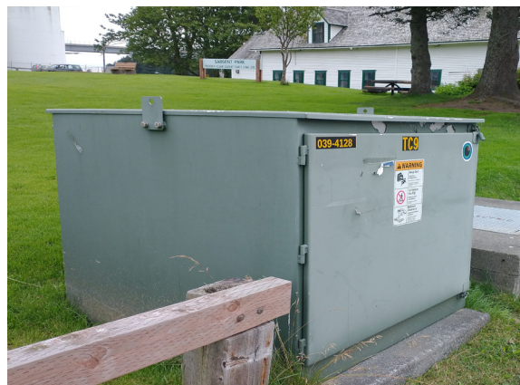
Figure 1-402. Utility Transformer (JSW, 8/25/2021)
