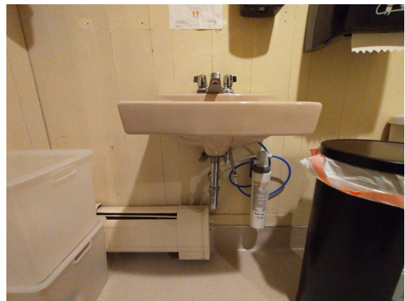
Figure 1-388. Second Level Lavatory Filter (JSW 8/24/2021)
