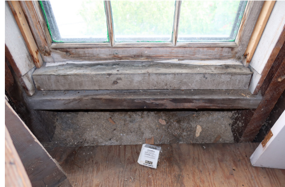
Figure 1-344. Water-stained wood around the sill of Window 33. (EAV, 08/24/2021)
