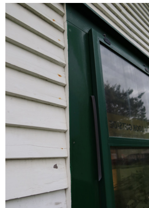
Figure 1-194. Loose sealant strip at storm of Window 22. (EAV, 08/24/2021)
