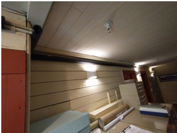
Figure 1-399. Second Level Fire Sprinkler Heads (JSW 8/24/2021)
