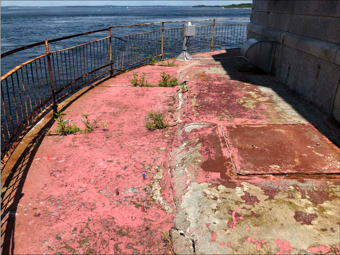
Photo 9. General view of the Drum deck and perimeter railing, both of which are currently in an unsafe condition. Bulkheads to the right provide access to the cellar and stores; in their deteriorated state, and without being safely cordoned, they harbor potential for a serious fall to nearly one story below.
