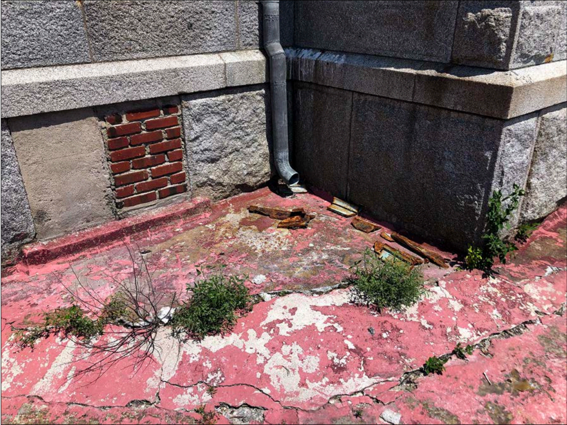
Photo 8. The Drum's deck surface is a crucial first line of defense, protecting the foundation and stores below. Cracks and breaching allow infiltration of vegetation and other organic matter, exacerbating the condition. Rainwater, left to spill adjacent to foundation walls, compounds deterioration. Note shards of cast iron that have fallen from the Lantern above.
