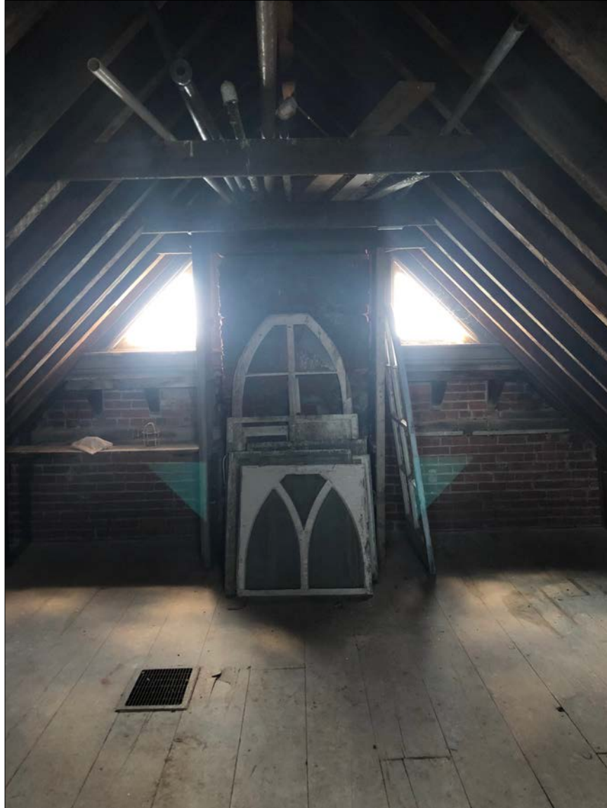
Photo 20. The attic space is clear and pristine, with few issues of concern relating to condition, structural integrity or usefulness. Remarkably, many of the original wood windows – swapped for utilitarian versions by USGC – have been stored for safekeeping; these should be re-integrated during the Lighthouse restoration, where they can exceed new energy standards.
