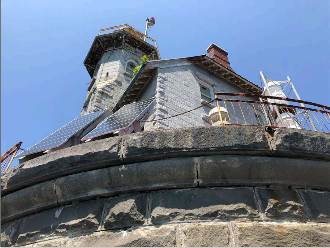
Photo 6. Missing rails, open masonry joints, gutters filled with organic matter, and similar myriad but addressable issues combine to undermine stability, even of structures built to last hundreds of years or more.
