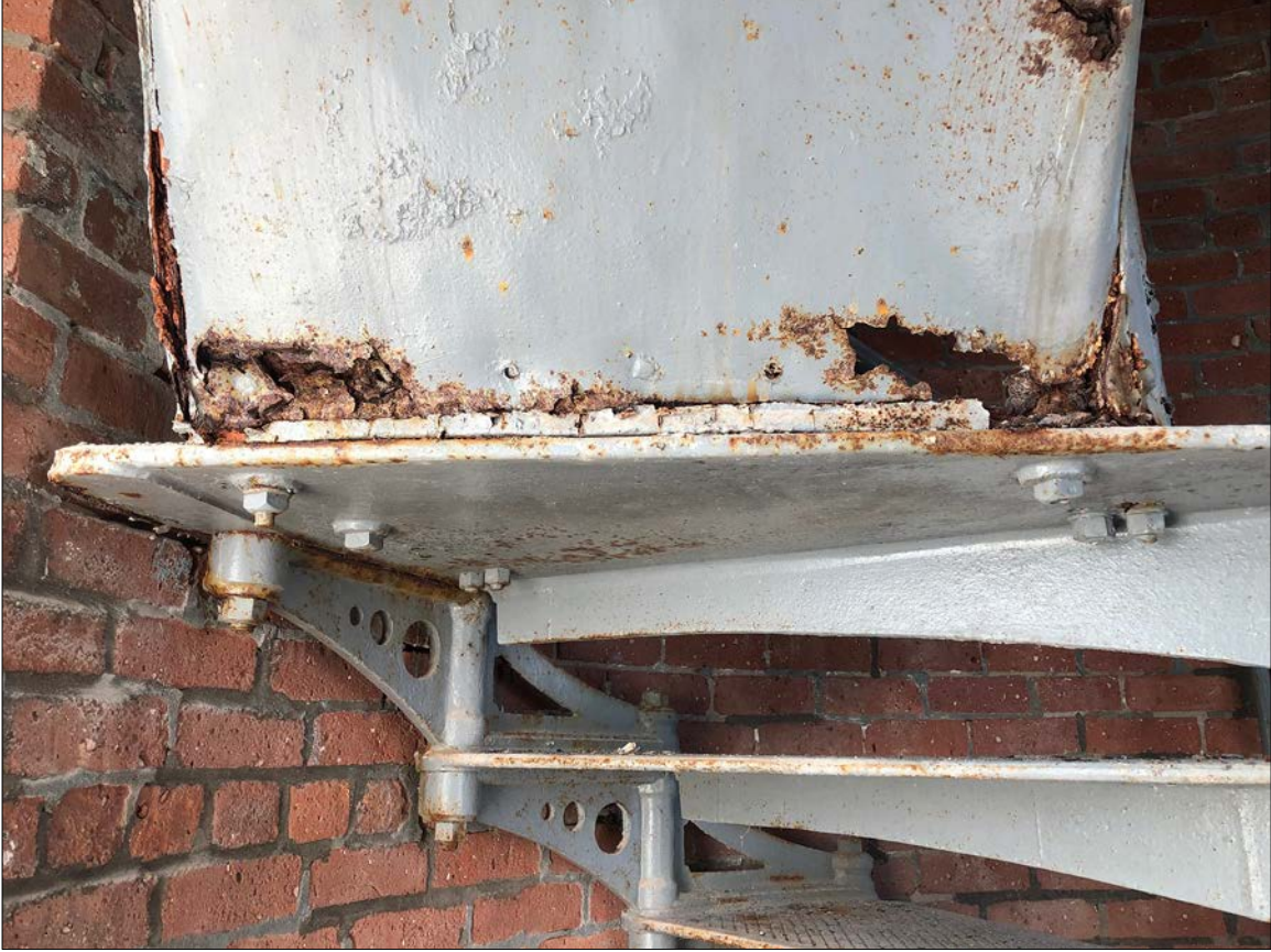
Photo 23. Just beneath the Lantern Level, the final stair run is permeated with rust resulting from water ingress above as well as deposition of condensation from being closed for long periods. Despite its appearance, damage such as this remains very restorable.
