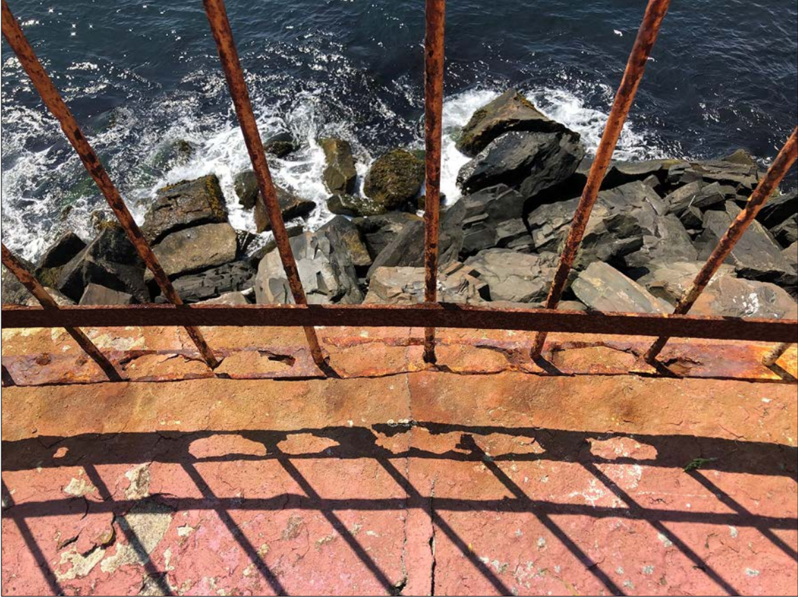
Photo 10. Perimeter iron railing, embedded into concrete Drum deck, is strong but corroded. It also is discontinuous. Despite these conditions, this early railing remains restorable and may be refined to meet current building safety standards.
