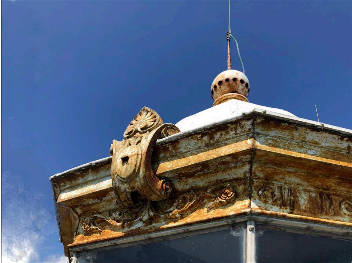
Photo 14. A cast iron cartouche, as well as embellishments of the lower fasciae, demonstrate the celebratory nature of Lighthouse design; these were the technological marvels of their time, expressed in architectural details such as these, as well as in literature and visual arts. Their allure is undiminished.
