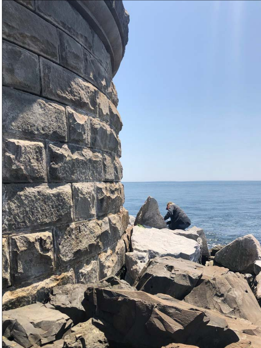
Photo 5. Years in the making, the granite sheathed concrete drum is an inherently rugged core, yet there are locations of distress rendered from lack of continual maintenance that would have occurred with a Keeper.
