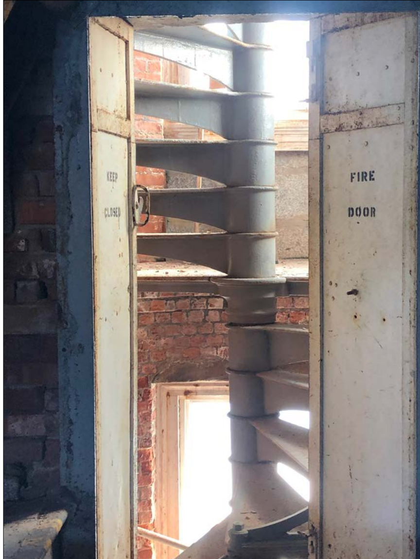
Photo 22. Cast iron spiral stairs continue directly to the Lantern, via the attic and Service Level of the Lighthouse. Water seeping through the Lantern's cast iron elements is evident throughout.
