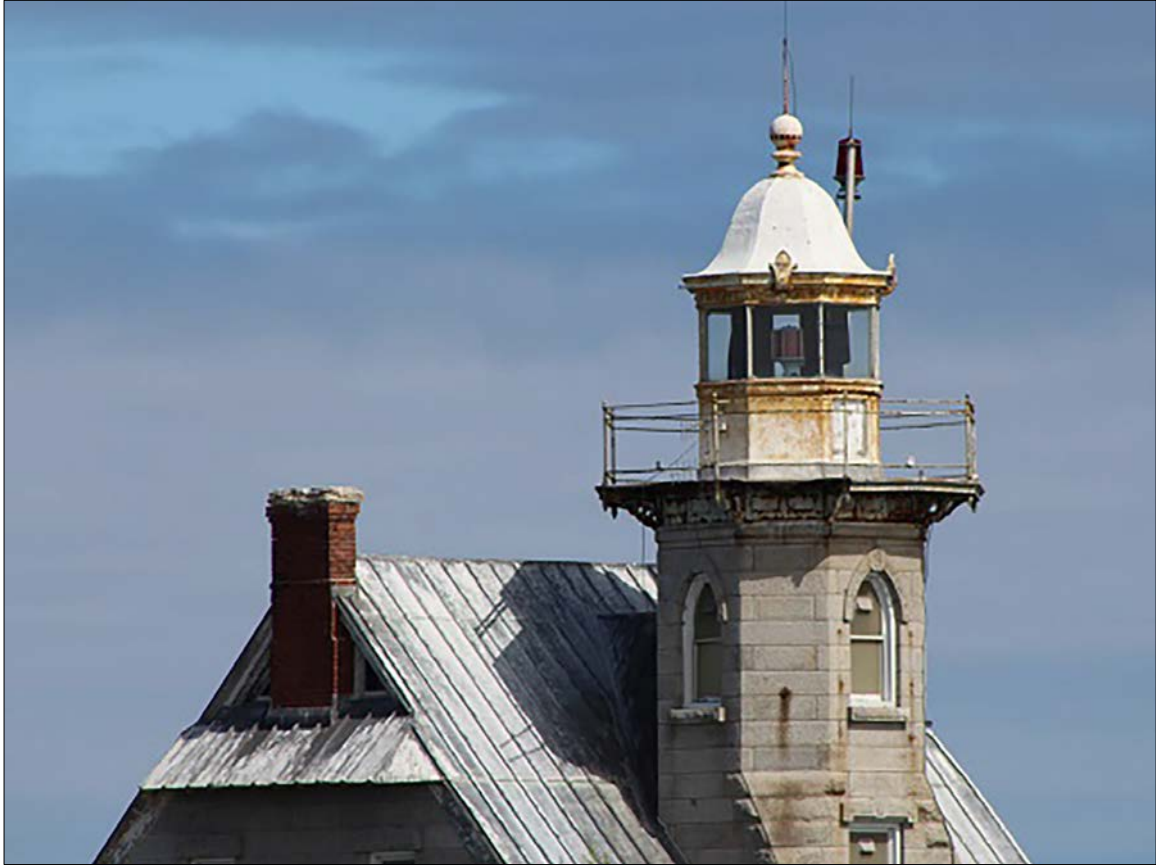
Photo 12. Drone view of Lantern, upper tower, chimney and south roof slope. Photo credit: Jim Tracy US Beacons.
