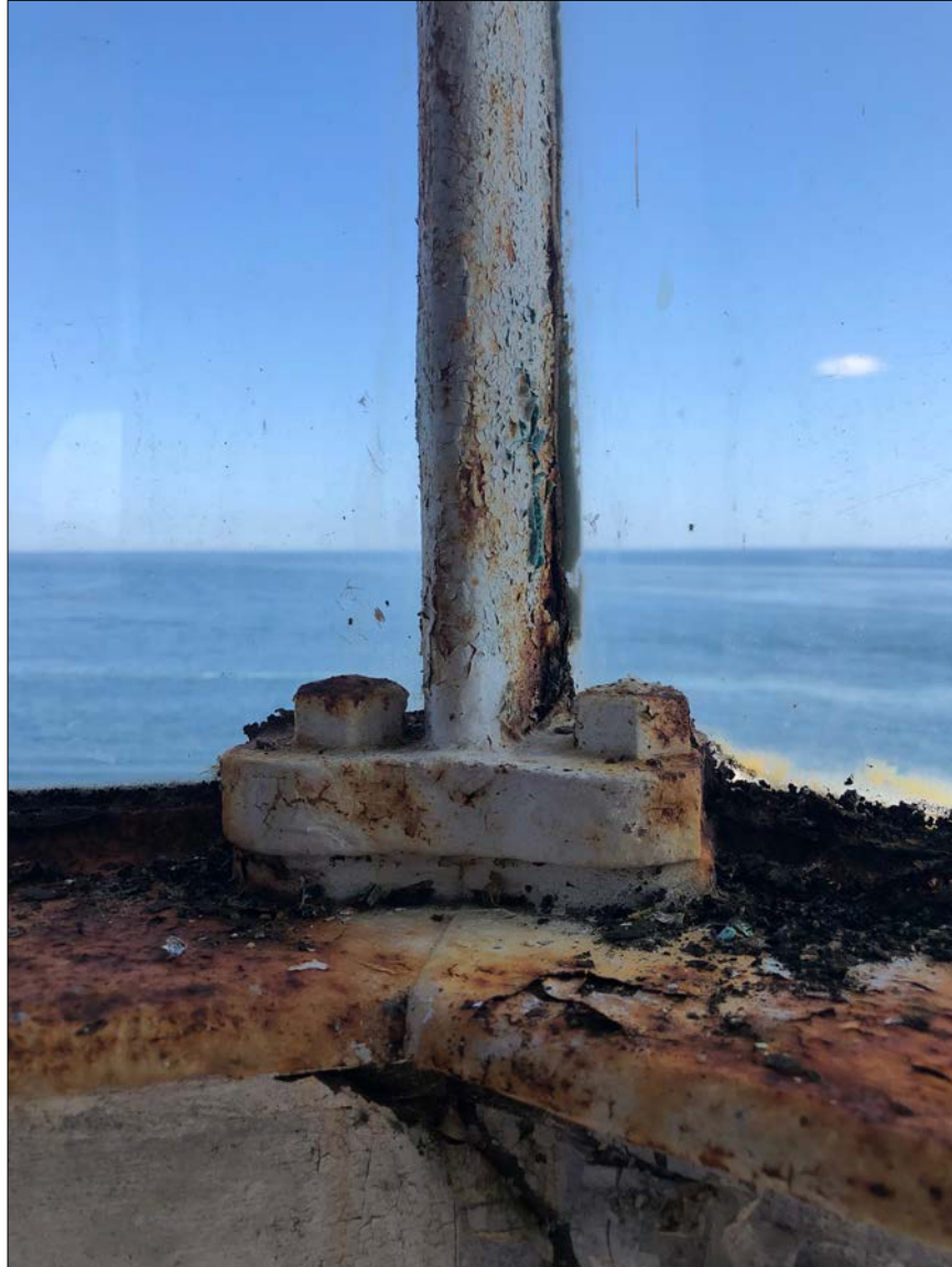
Photo 24. Within the Lantern, the vertical bars, sills, vents, spider frame and various related elements all suffer from lack of a Keeper who could attend to small coating & repair issues before they became large. Most elements are intact, which speaks well for the success of the planned restoration.
