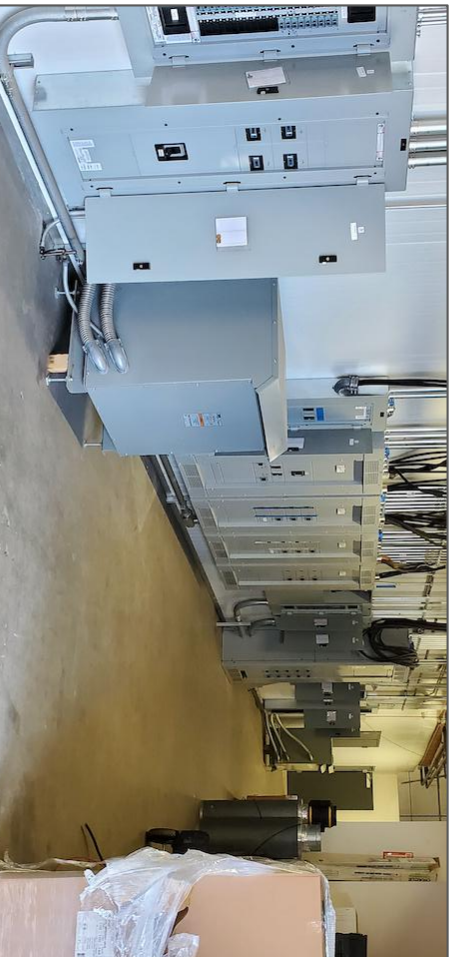
Electrical panels at 5733 San Leandro (serving RNK)
