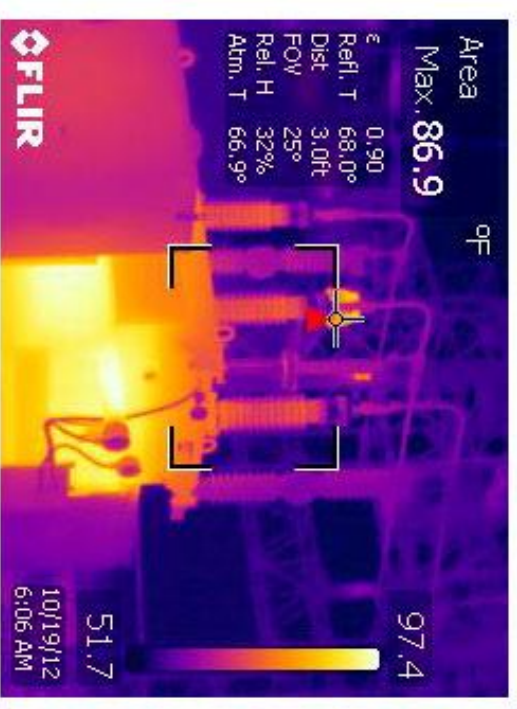
An overloaded (and overheated) utility transformer
