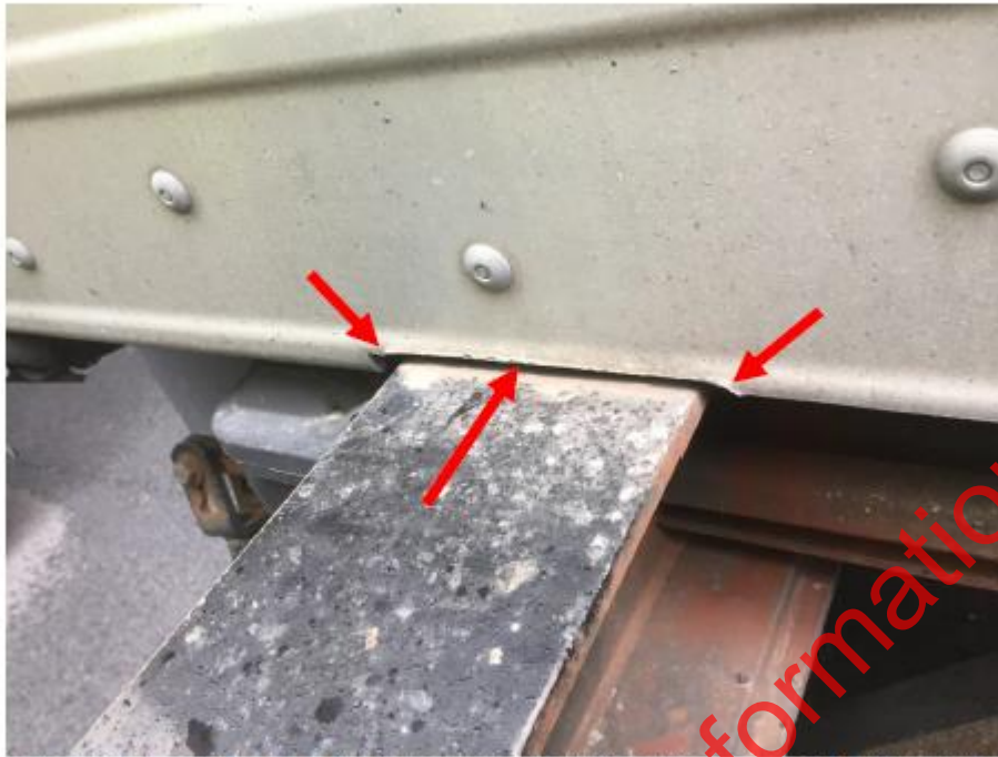
Failed welds on the floor front cross members lead to movement between the chassis and the front of the body and with experience this can provide an indication of broken welds.
