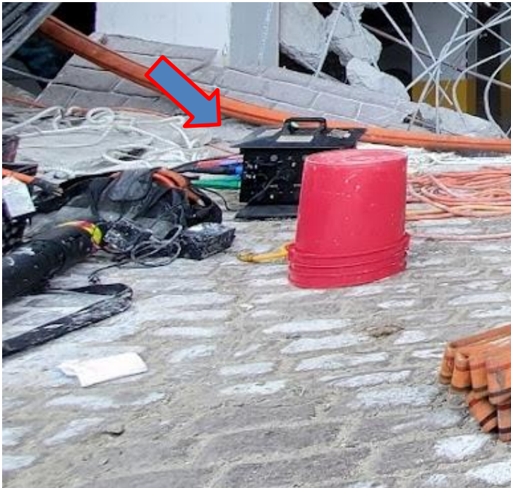
Image 3: Portable distribution box
