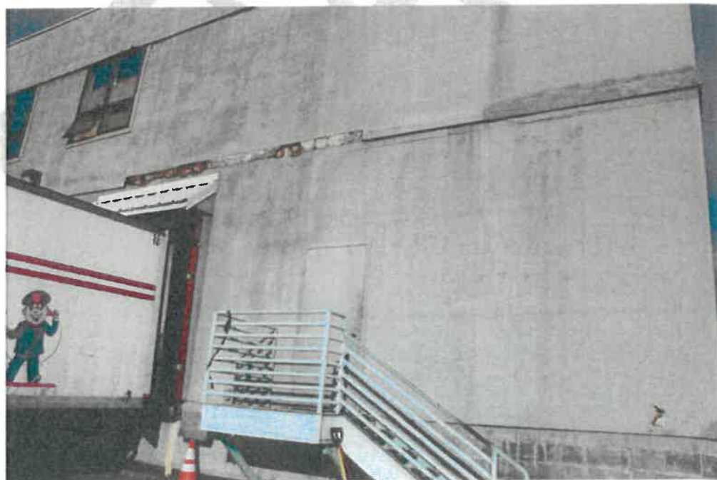
Photograph 10.1-3 – Deteriorated / missing wood trim at stucco, impact damage at southeast building corner
