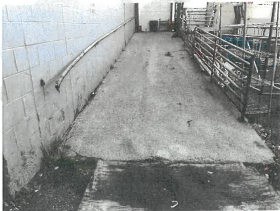
Photograph 5.2-3 – Service ramp: broken handrail, subsiding asphalt at bottom of ramp
