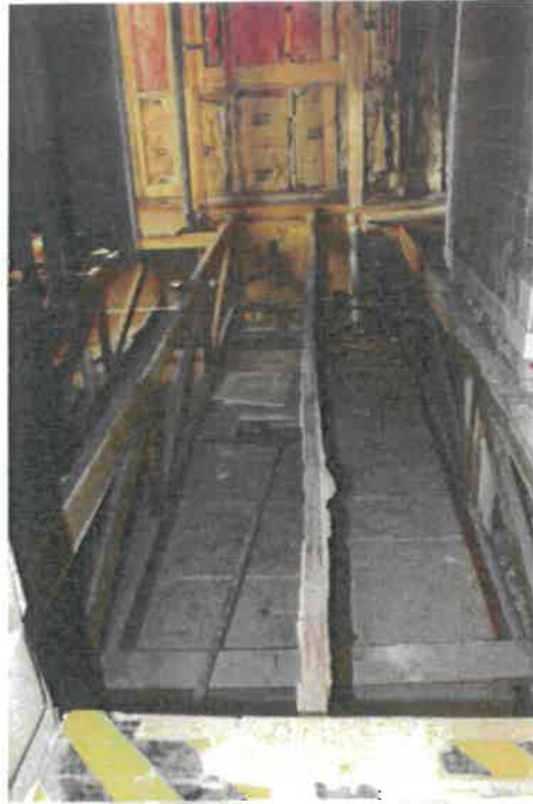
Photograph 9.0-1: Structural Damage, Residential Wing 2 nd Floor
