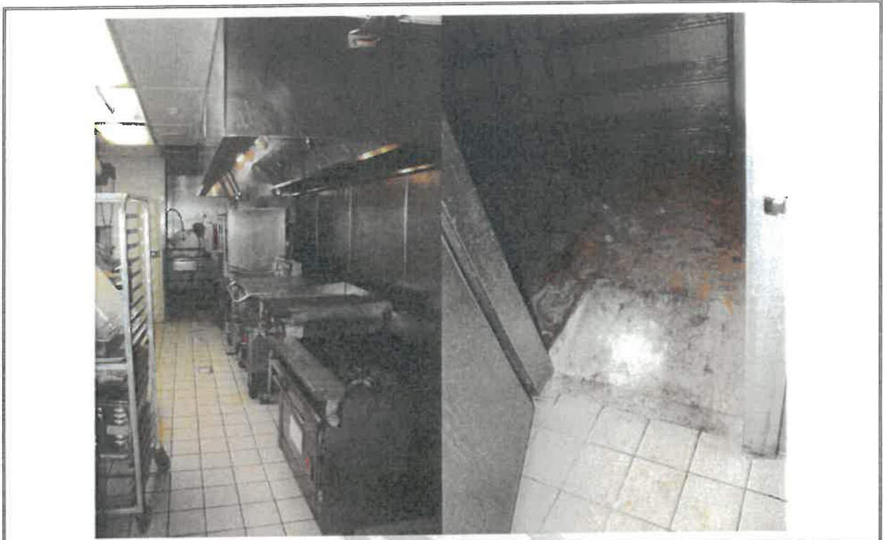
Photograph 17.7-1 – Kitchen: cook line and hood (left), walk-in floor rusted and missing (right)
