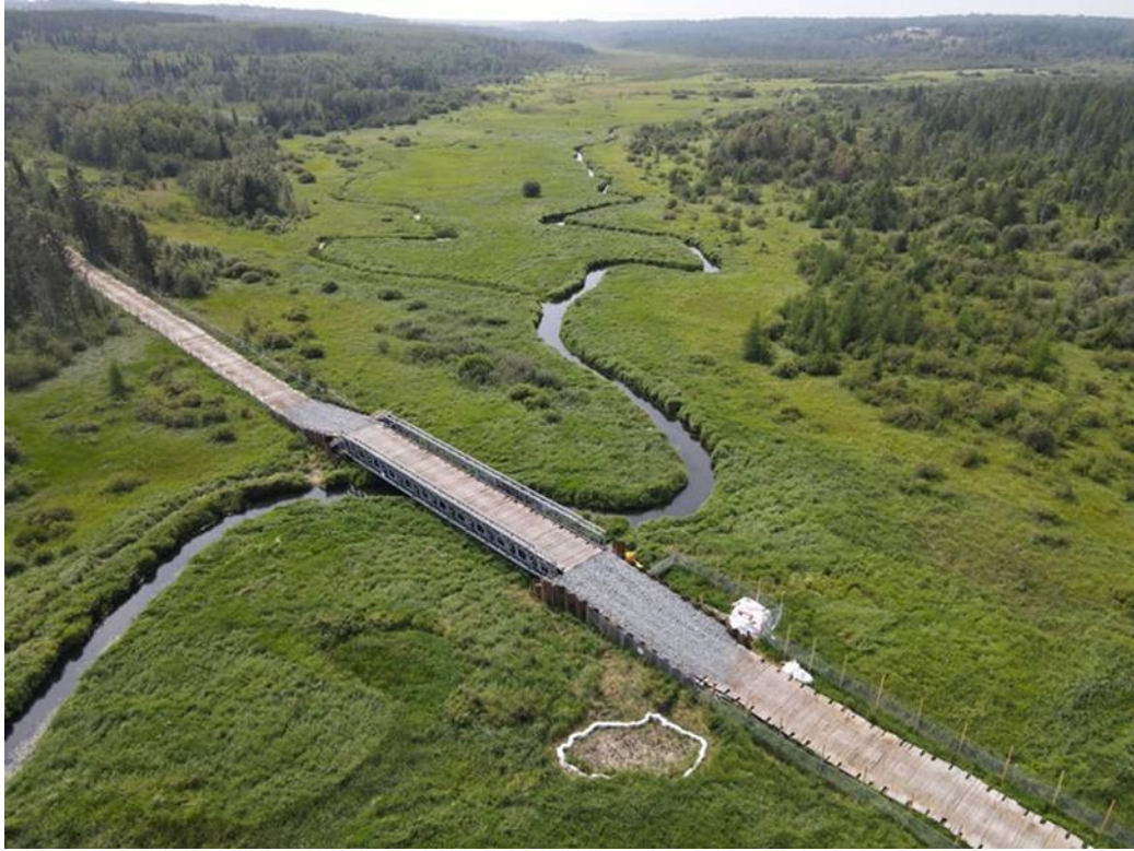
Figure 1. Mississippi River Crossing Fracouts during construction July 2021. Image by Indigenous Environmental Network
