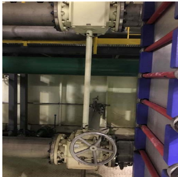
Figure 10. TLO cooler 6-way transfer valve. 37
