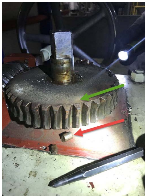
Figure 11. Stop pin (red arrow) found under gear (green arrow). 40
