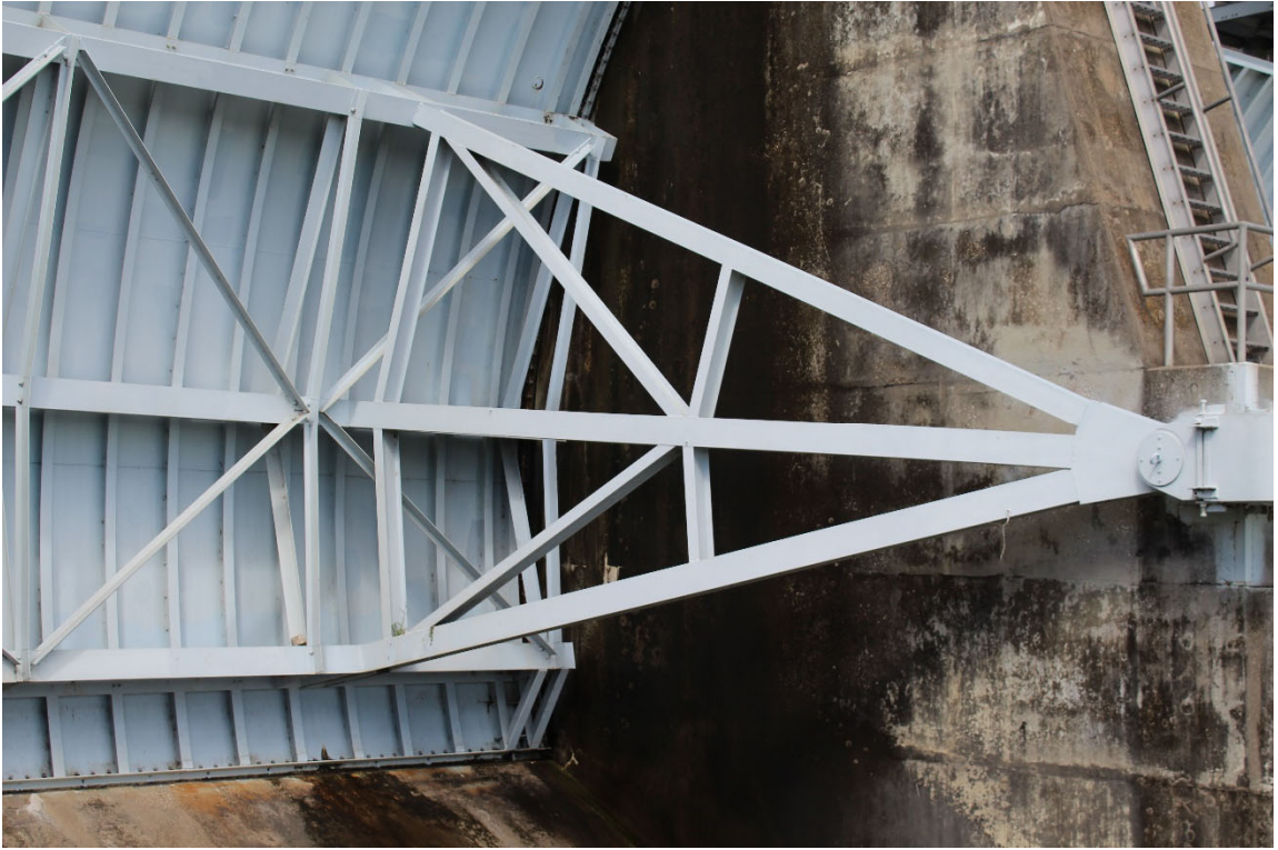
Photo 3-2: Left strut arm, Forney Dam (typical).
