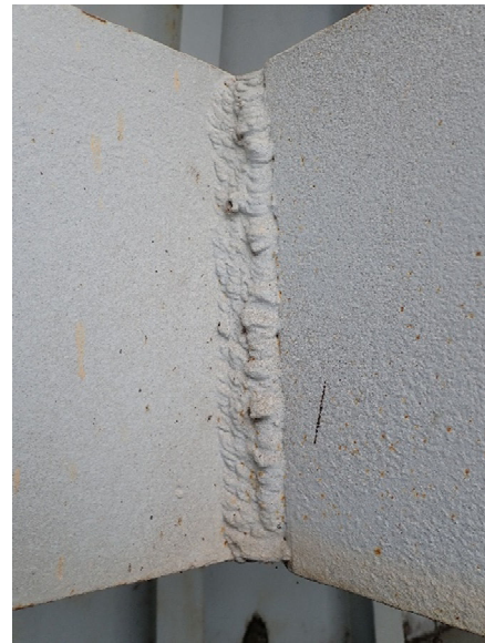
Photo 5-4: Example of a poor quality weld.
