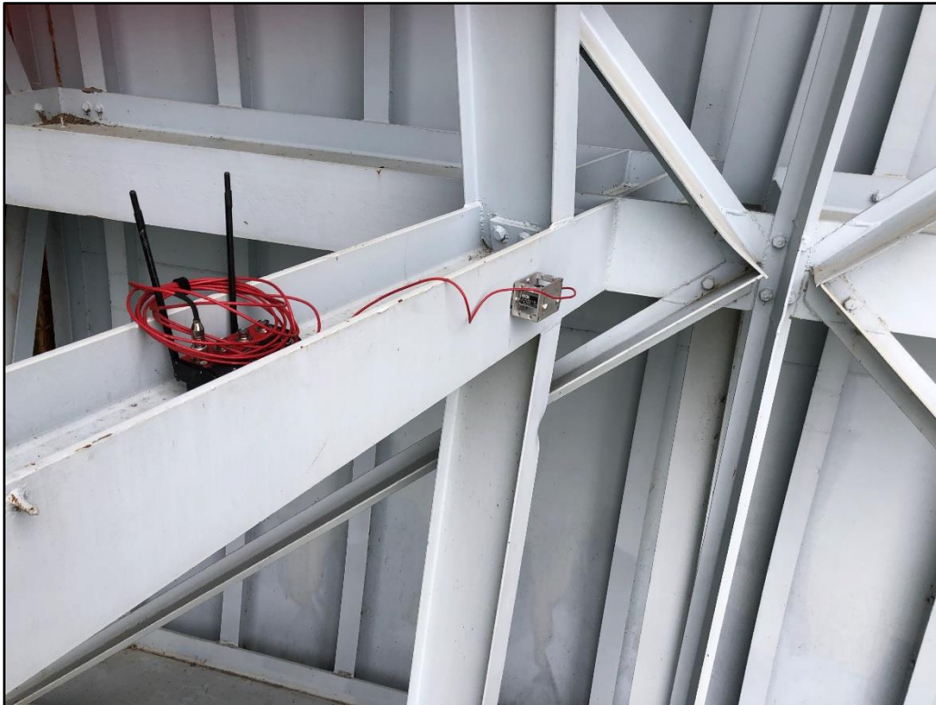
Figure 2 – BDI tiltmeter rotation sensor installed near skin plate (Typical)
