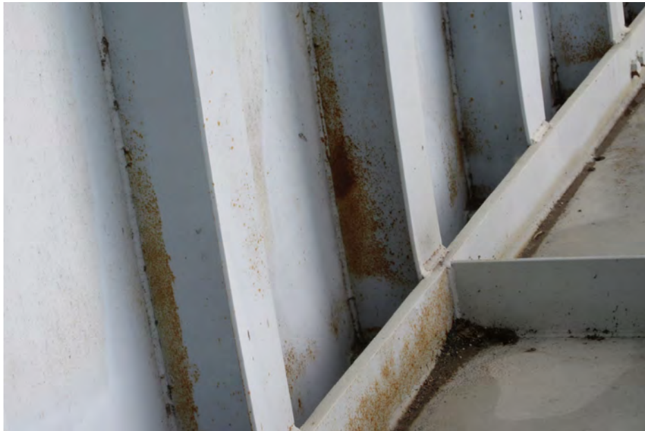
PHOTOGRAPH No.: 10 GATE: Gate 5 Photo Taken: 3/31/2020 File: DK-34.jpg
