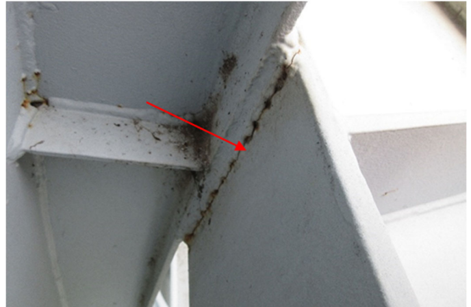
Photo 5-3: Fractured weld between the vertical rib and horizontal girder.
