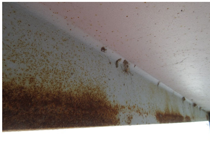
Photo 5-1: Local coating failure.
