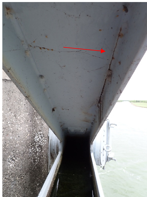
Photo 5-10: Bottom of member LS-1 (Gate 6) showing fracture between flange and web.
