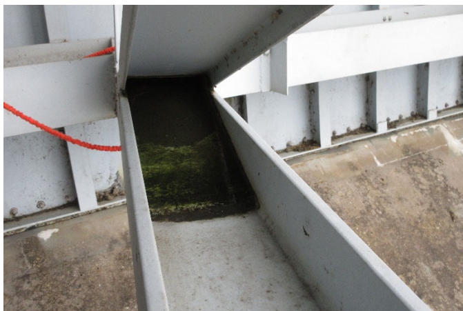
Photo 5-2: Water trapped in between the flanges of a primary strut arm due to clogged drainage hole.
