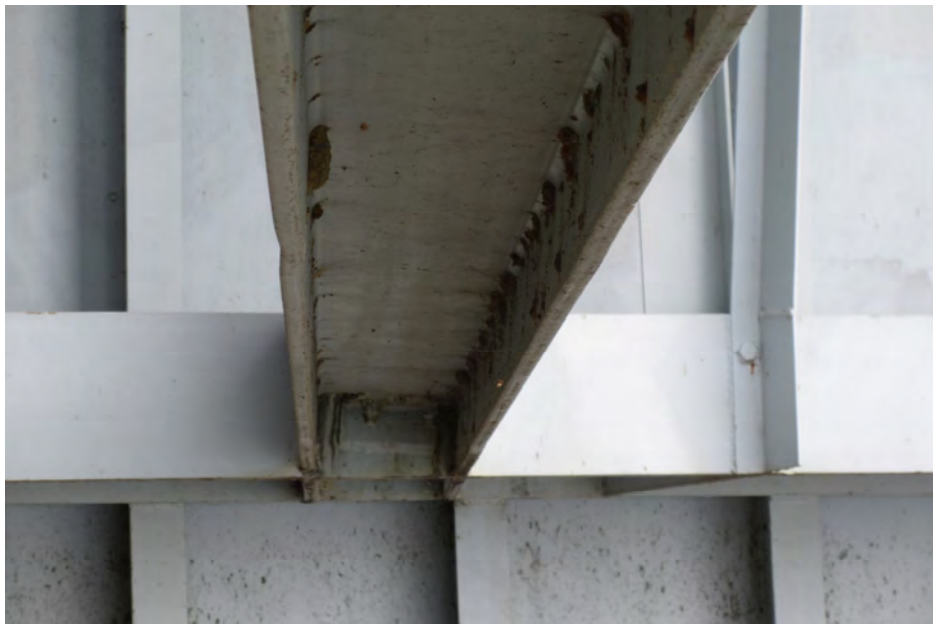
PHOTOGRAPH No.: 2 GATE: Gate 3 Photo Taken: 3/30/2020 File: DK-2.jpg
