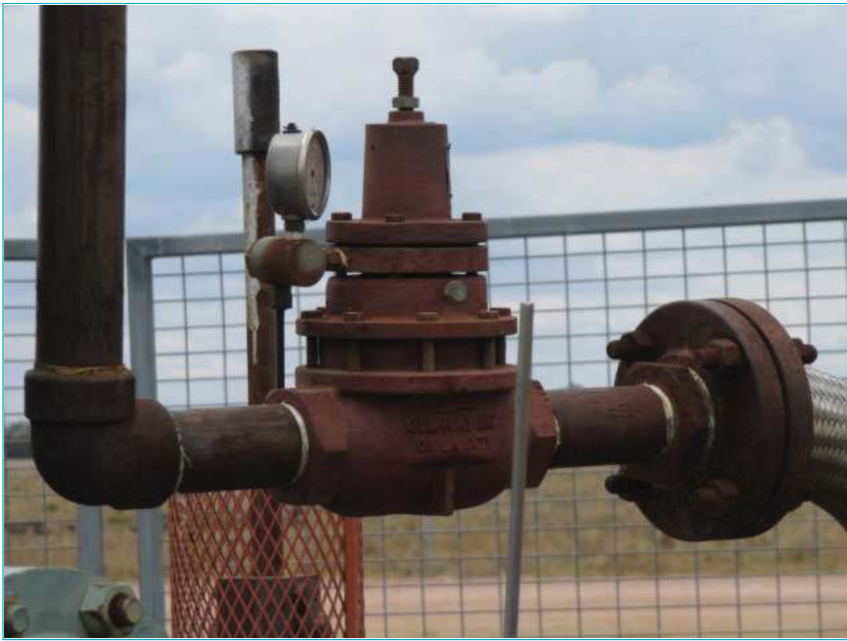
Figure 5.2. Pressure regular that was a common source of CH 4 leakage.
