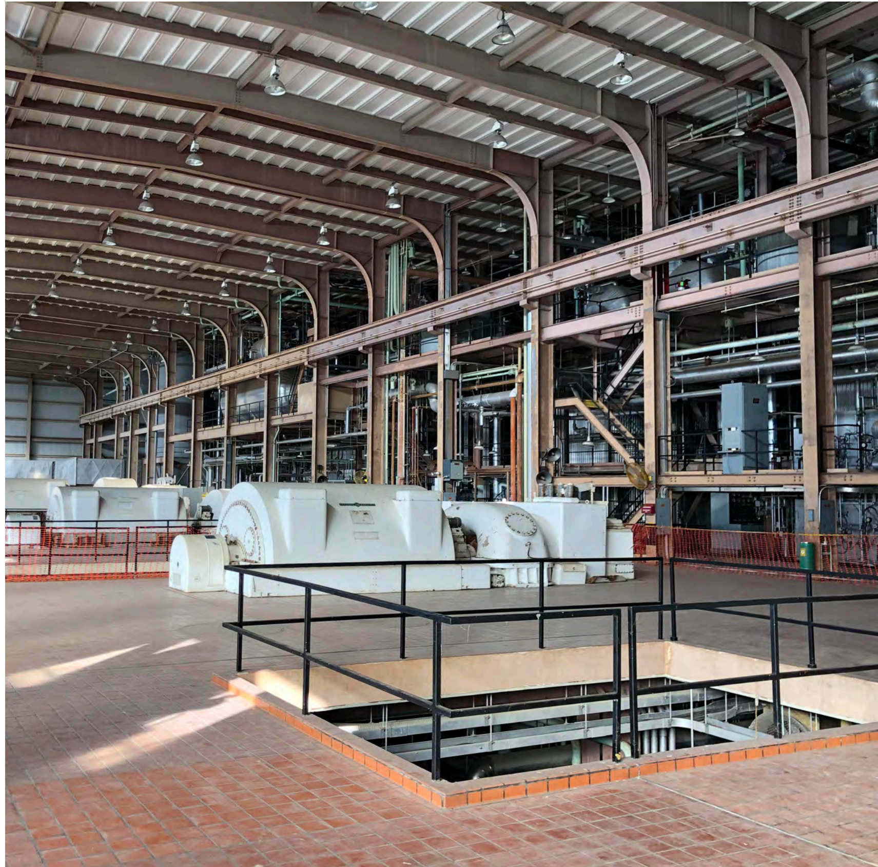
Main Turbine Hall (Facing North)
