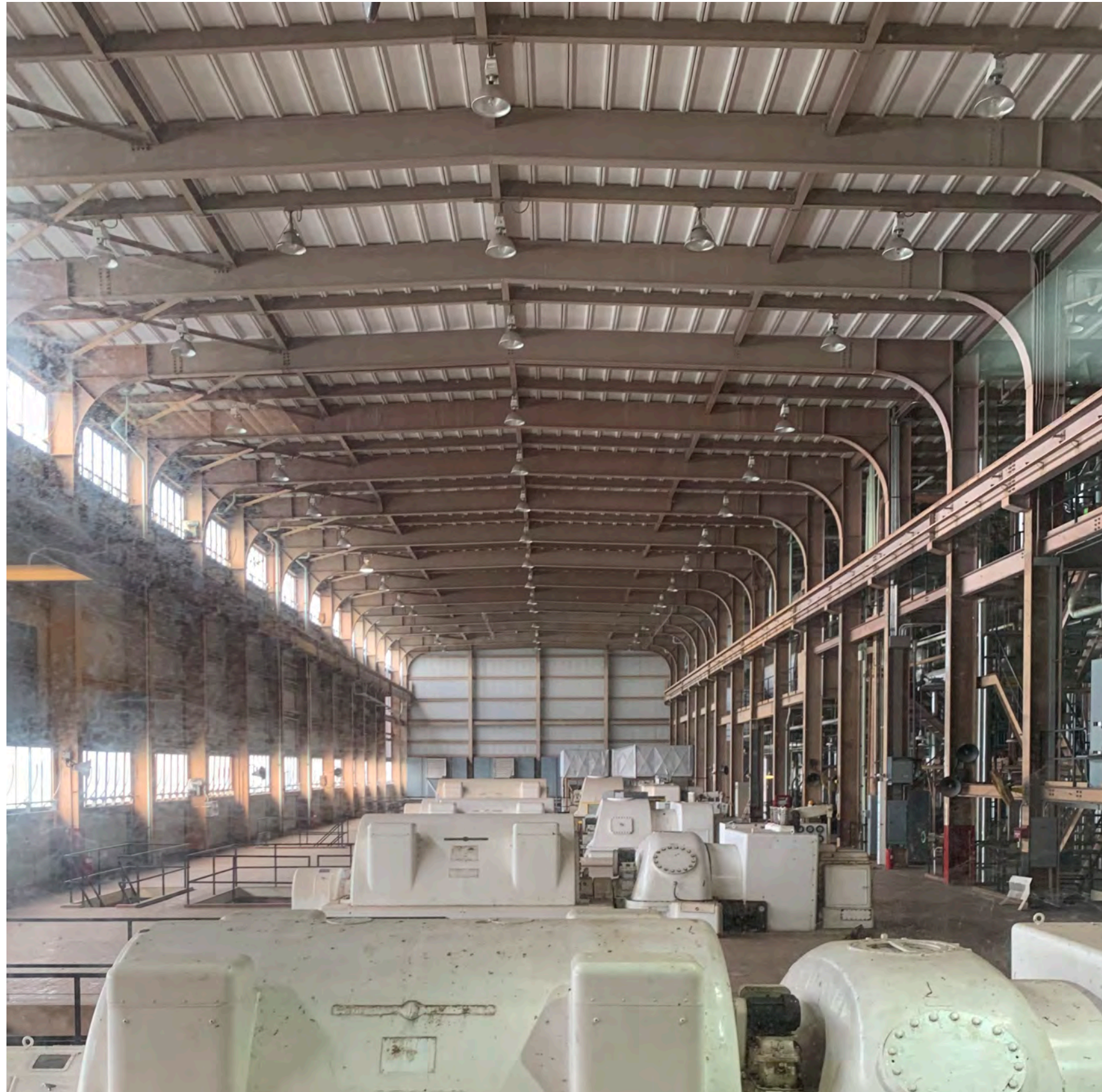
Main Turbine Hall (Facing North)
