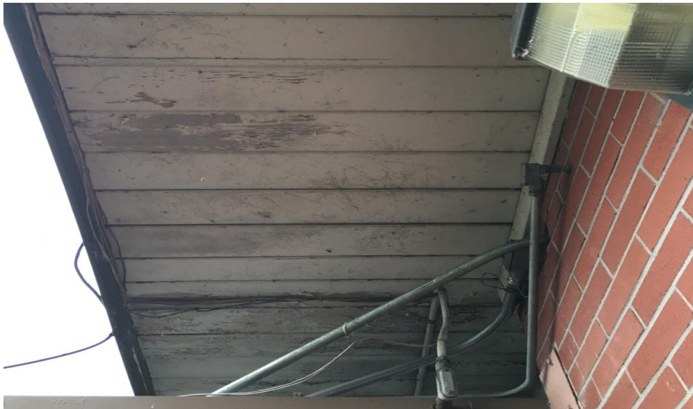
2. Administration Exterior – Peeling lead-containing paint on soffit.
