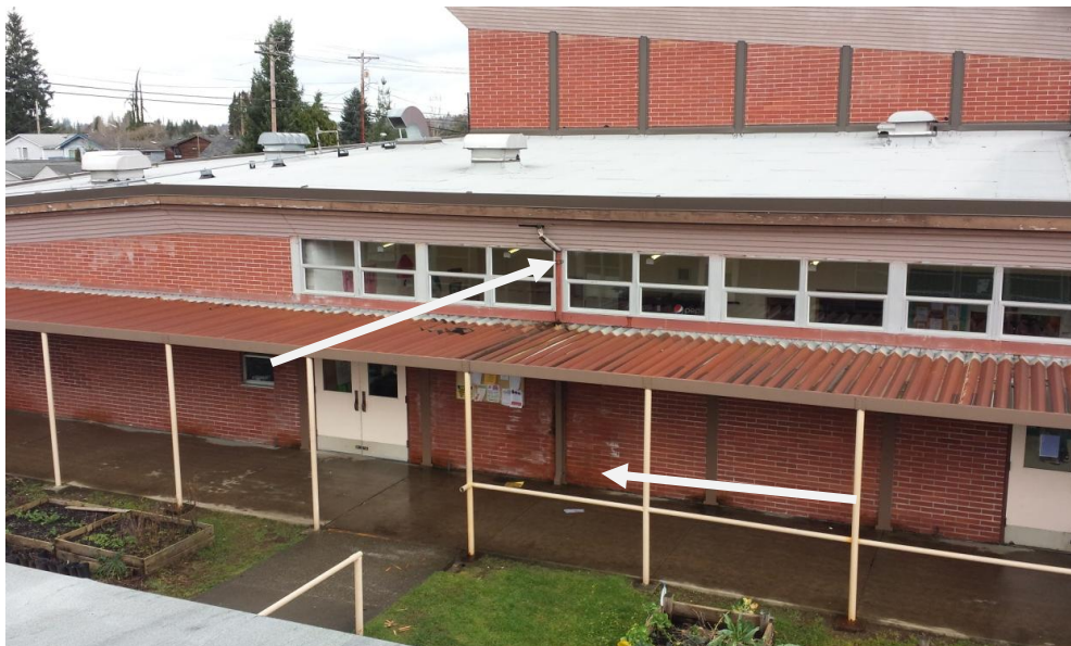
40. Gym Building South Exterior Wall – Damage roof water drainage system causing water to flow down the outside of the building and intrude into the building.
