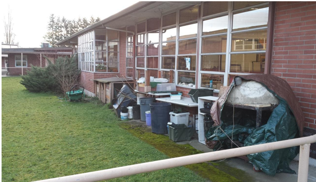
32. Annex Exterior – Garden equipment, compost pile, dirt/debris, and garbage cans placed in front of and surrounding the outside air intake of Room C.
