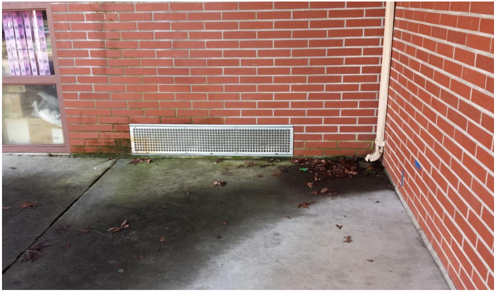
63. Library – The roof stormwater drain leaders direct the flow of water directly in front of the unit ventilator outside air intakes. Biological growth surrounding the intake grill.
