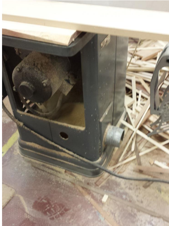
57. Technology Building Woodshop – No sawdust collection system on table saw.
