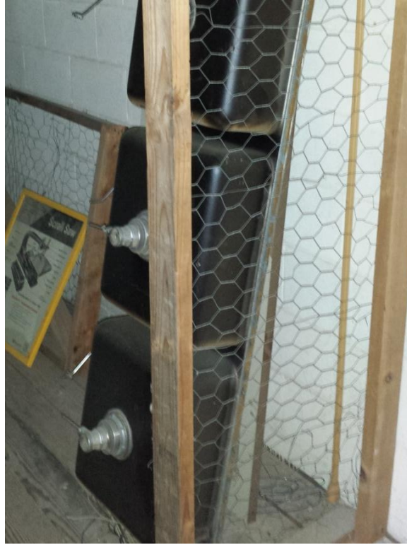
53. Technology Building – Sinks with asbestos-containing coating in mechanical attic.
