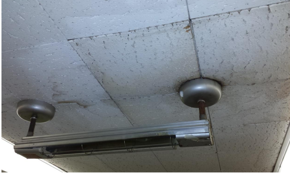
9. Annex Room B Prep – Water damaged ceiling and heating element. Suspect fungal growth present.
