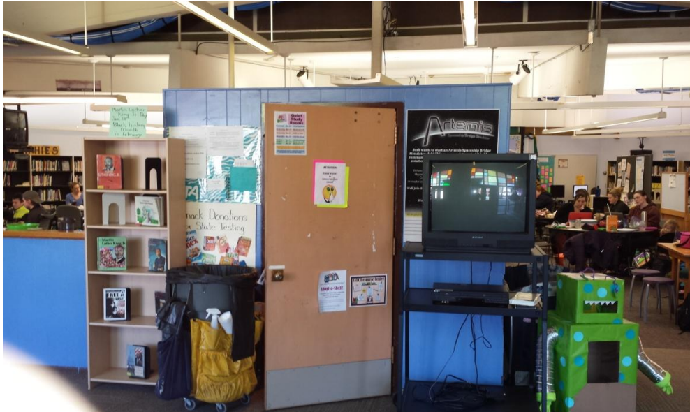
61. Library – Custodial closet with water damage and fungal growth around base of wall.
