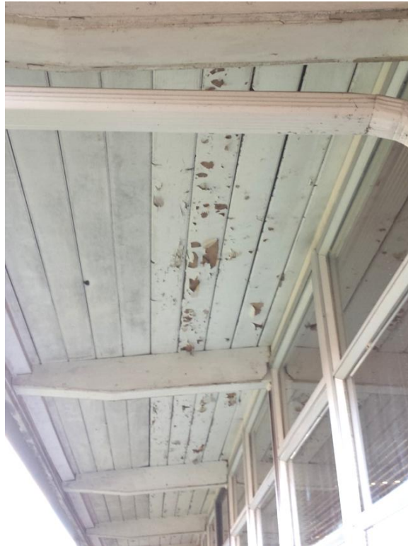
33. Annex Exterior – Peeling lead-containing paint on soffit.
