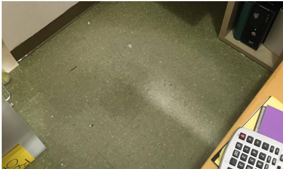
50. Gym Gathering Place West Office – Abrasion of asbestos floor tile from chair rollers.
