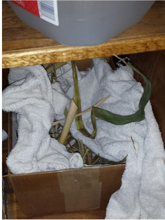
23. Annex Room F – Moldy plant grasses/leaves on shelf.
