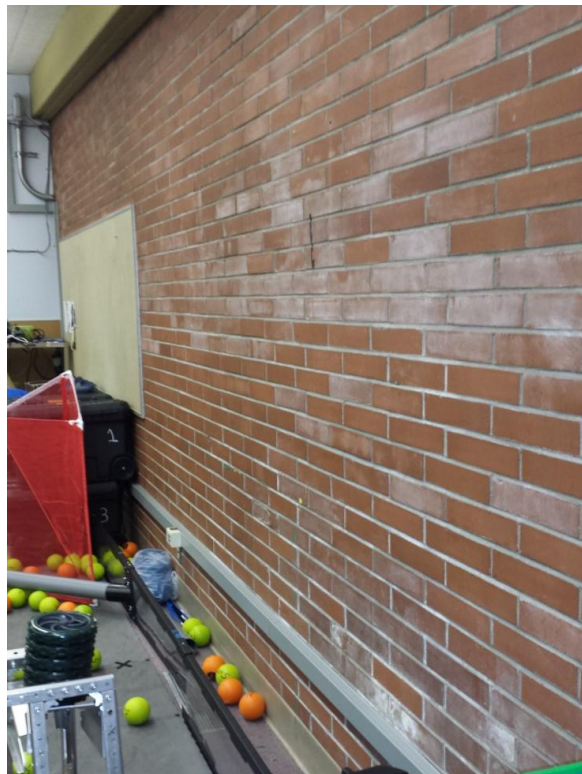
6. Annex Room B – Water intrusion east perimeter wall
