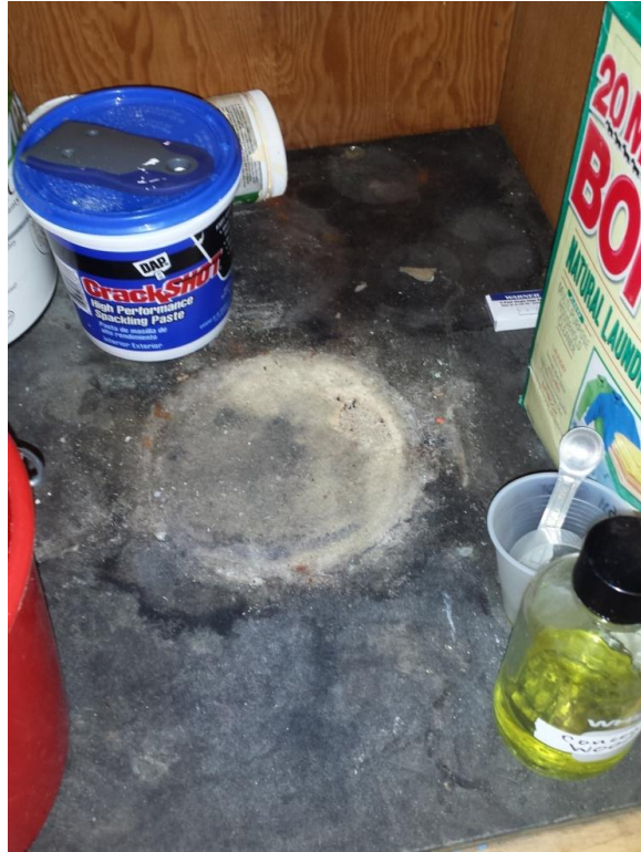
15. Annex Adolescent Montessori Prep Room – Damaged sink cabinet.
