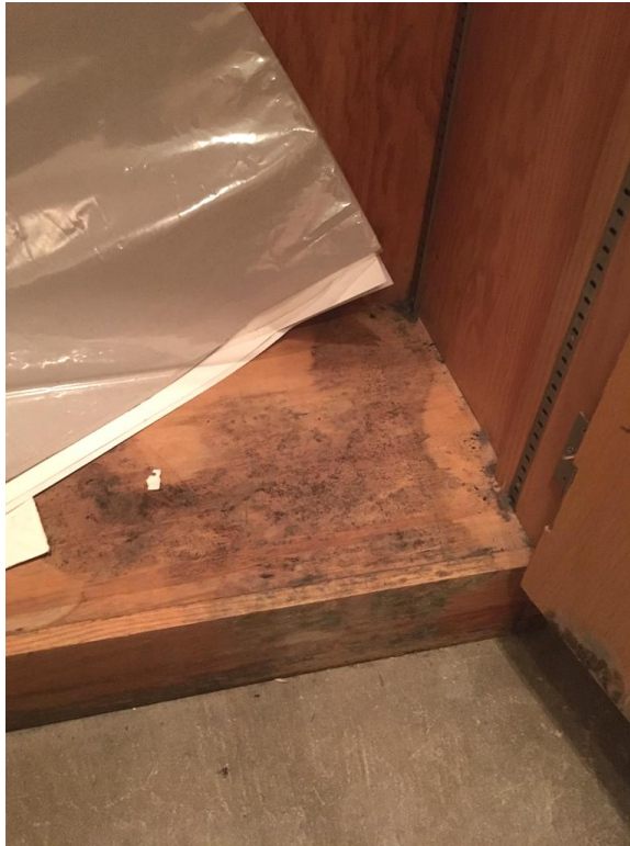
45. Boys Locker Room Wrestling Storage – Fungal growth in wood cabinet.
