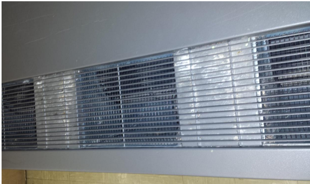
18. Annex Room F – White powder and other debris in unit ventilator supply.
