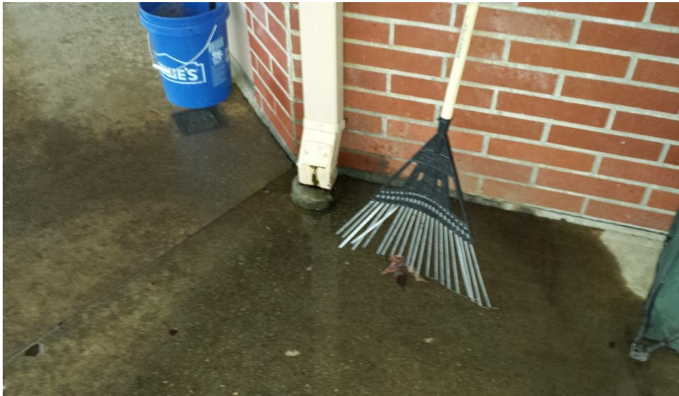
80. Classroom Pod Exterior – Roof rain leaders leak and ground drains are clogged causing water intrusion.
