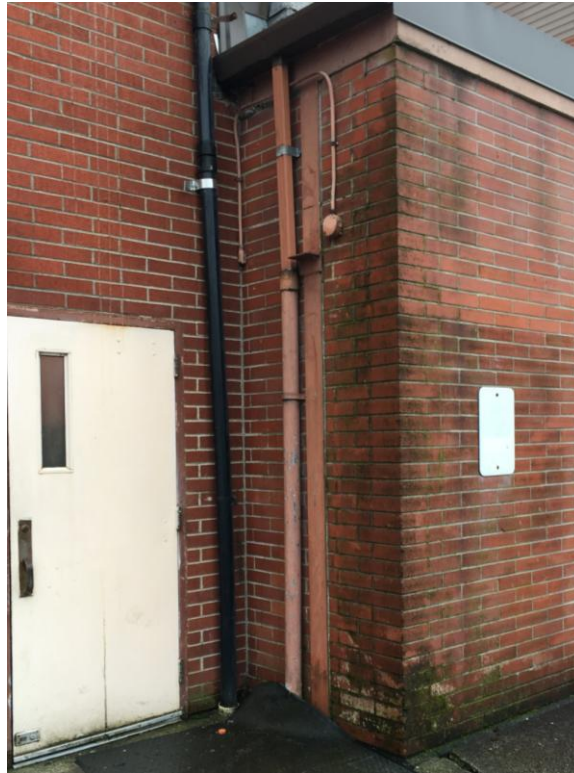
49. Exterior of Girls Locker Room (Archery Storage) – Long term rain water running down side of building causing algal and moss growth, efflorescence and water intrusion into the archery storage room.
