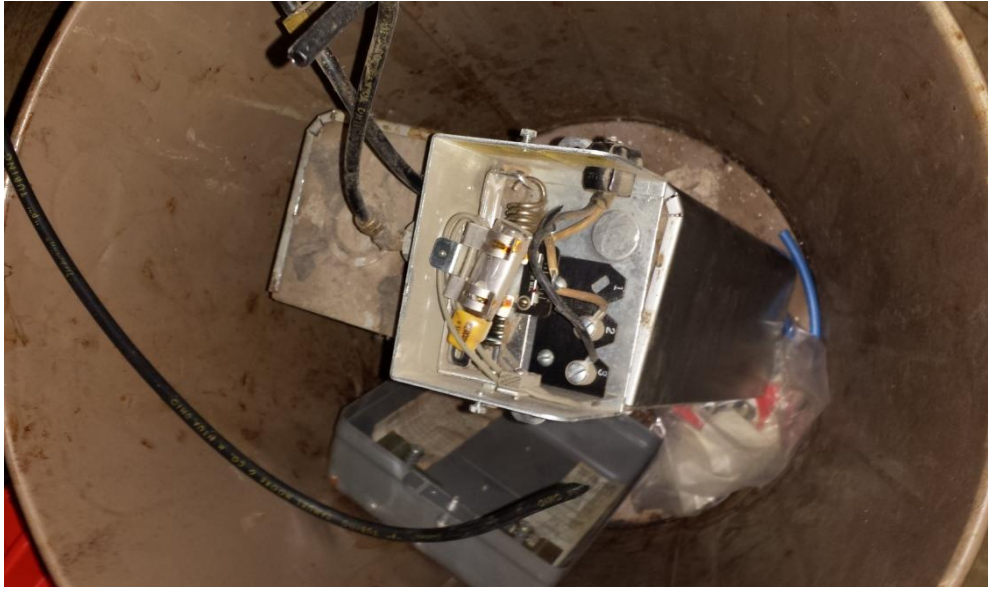
29. Annex Paint Storage Room – Liquid mercury electrical switch.
