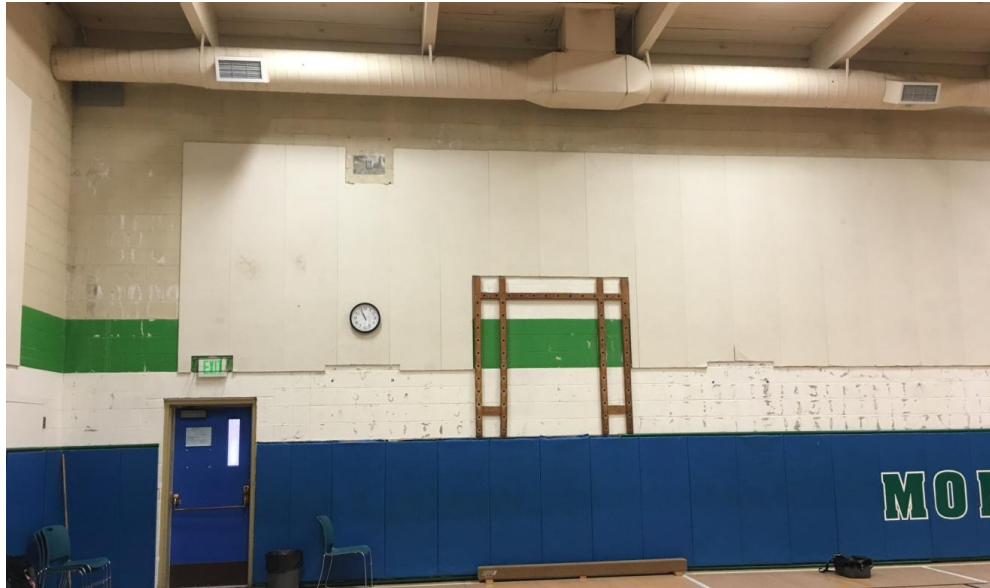
41. Small Gym East Perimeter Wall – Water intrusion through the exterior masonry wall has damaged the paint, caused mineralization. The water intrusion has caused fungal growth behind the sound insulation panels on the upper wall and behind the athletic safety pads on the lower wall.
