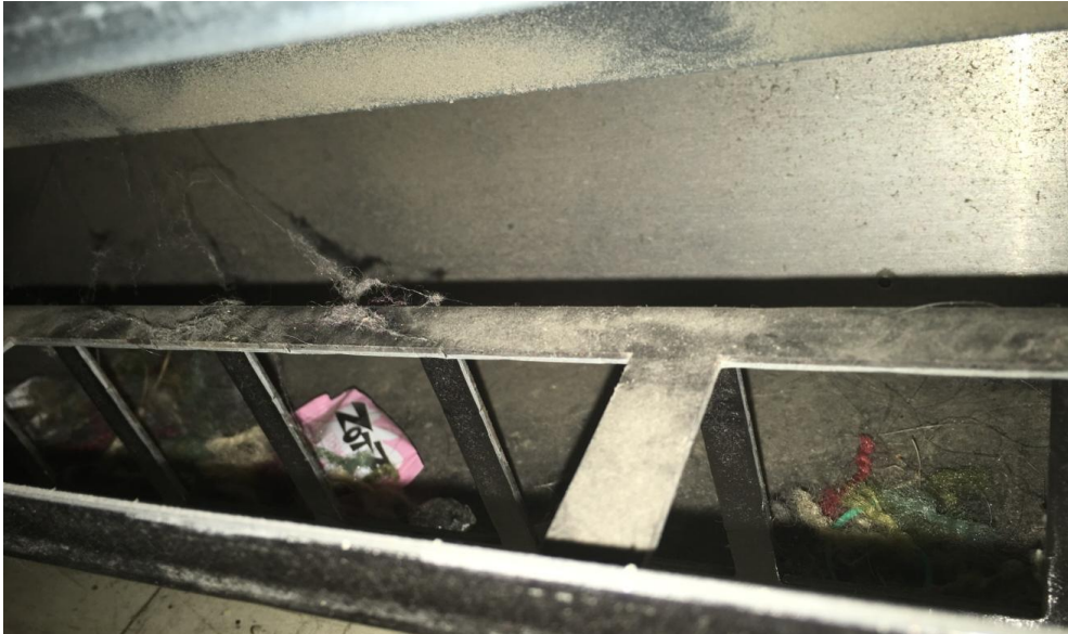
5. Annex Room A - Debris in unit ventilator return.
