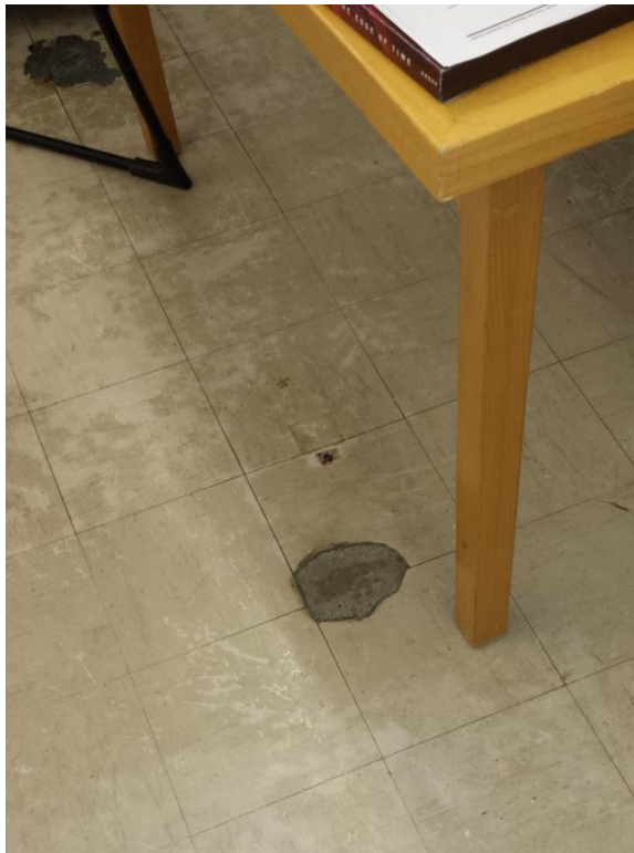
14. Annex Room C – Damaged asbestos-containing floor tile.
