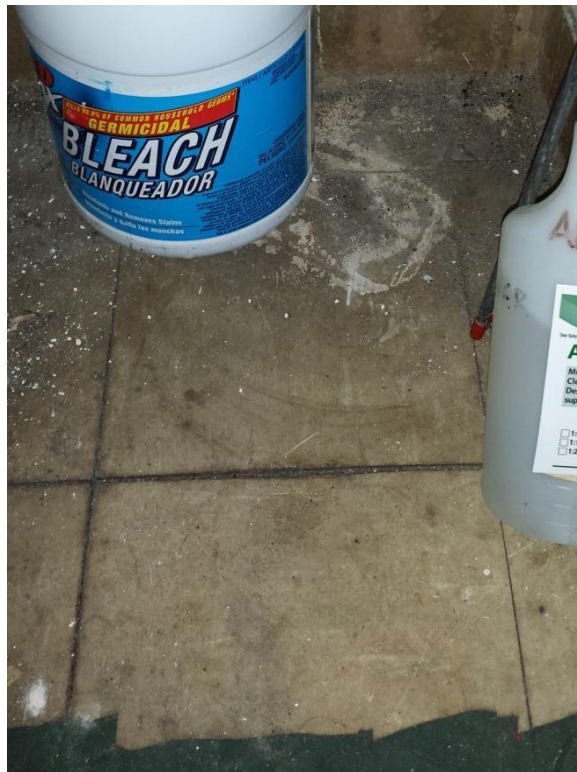
30. Annex Custodial Closet – Damaged delaminating asbestos-containing floor tile.
