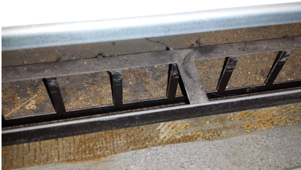
76. Classroom 8 – Concrete and carpet mastic debris in unit ventilator return from floor grinding activities.
