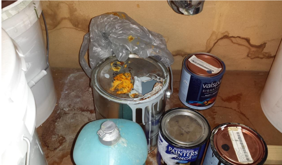
79. East Pod Central Common Area – Damaged can of paint under sink. Water staining on sink cabinet but no suspect fungal growth observed.
