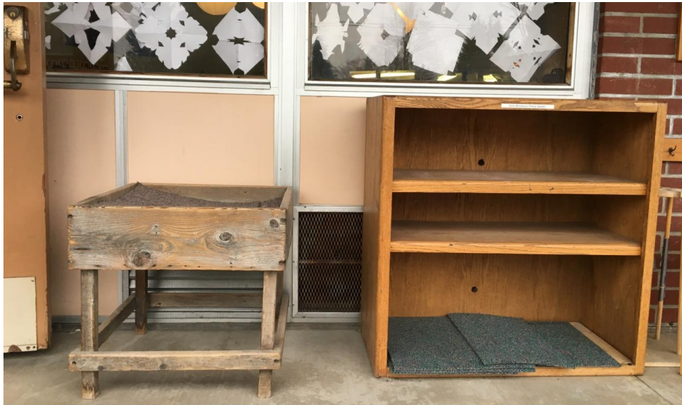
65. Classroom 4 – Outside air intake of unit ventilator blocked impeding air flow. Note the sandbox on the left.
