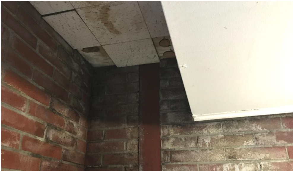
48. Girls Locker Room Archery Storage – Fungal growth and water damage on ceiling and wall.
