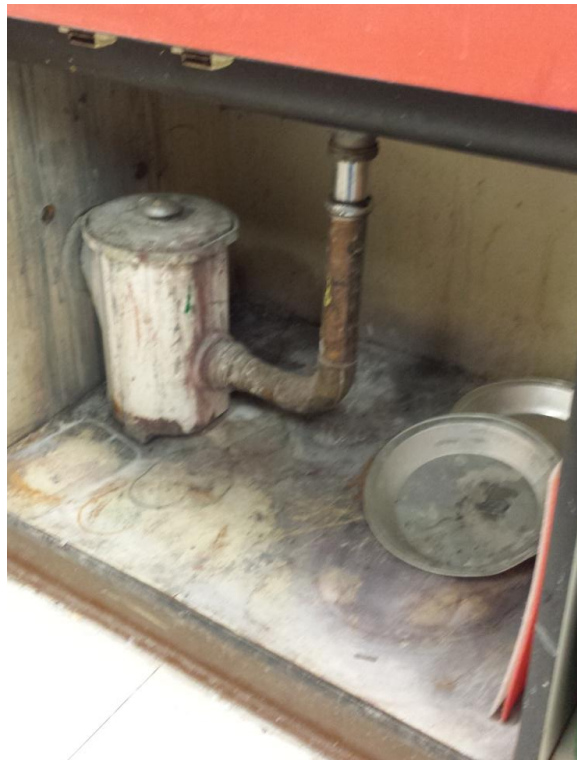
54. Technology Building Art Room – Two water damaged sink cabinets with fungal growth.
