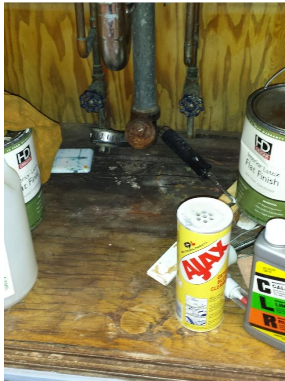
58. Technology Building Room 23 – Water damaged sink cabinet with fungal growth.
