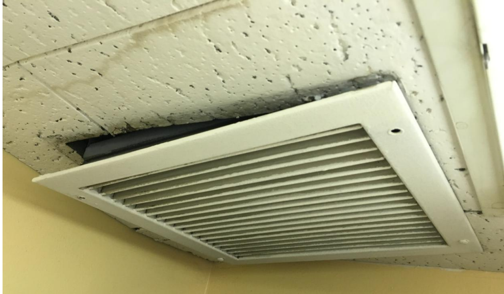
17. Annex Room D – Detached HVAC exhaust grill in entryway.
