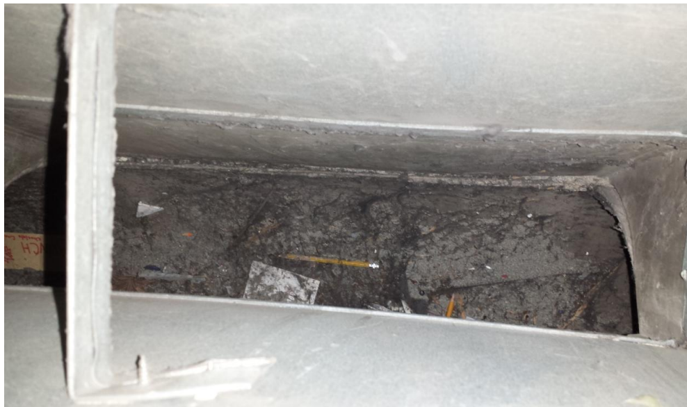
8. Annex Room B – Significant debris in the in-floor air supply duct.
