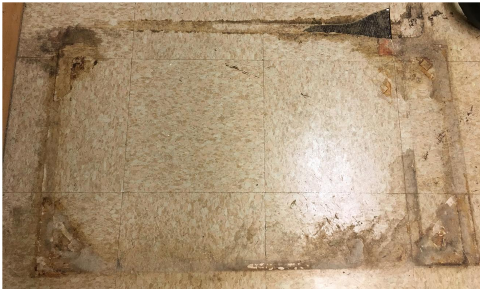
34. Music Room SPA Storage – Damaged asbestos-containing floor tile.
