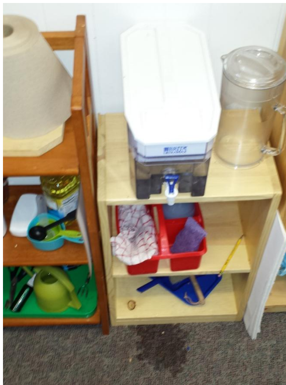
66. Classroom 5 – Water dispenser leaking on carpet.
