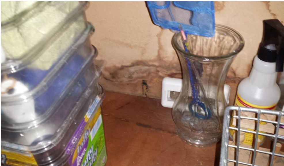
68. South Pod Central Common Area – Suspect fungal growth in sink cabinet.
