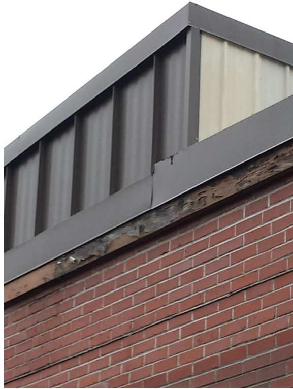
59. Technology Building West Exterior – Peeling lead-containing paint.
