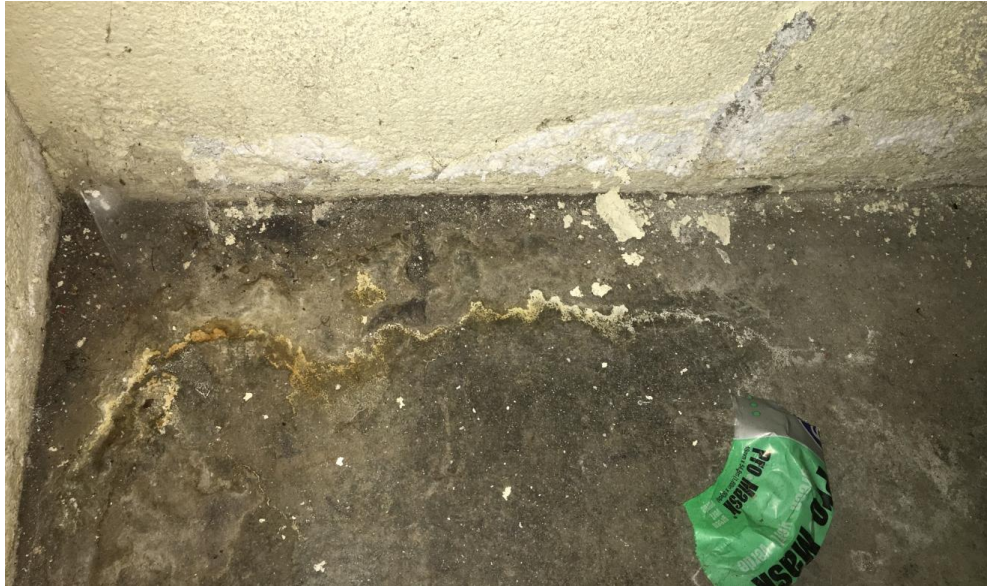
47. Boys Locker Room Wrestling Storage – Fungal growth and water damage on floor from leaking ice machine.
