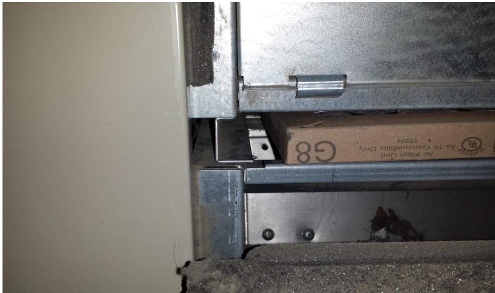
62. Library – Unit ventilator air filter does not fit properly leaving gap for air/particulate bypass.
