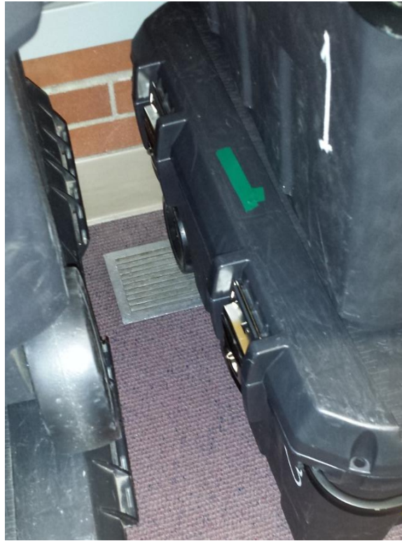
7. Annex Room B – Blocked in-floor air supply grill.
