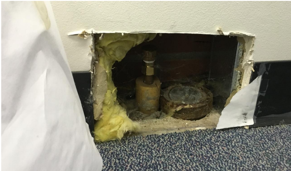
24. Annex 18-21 Transitions – Hole in east wall.
