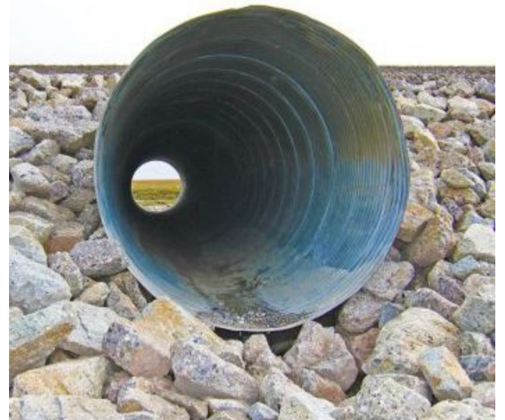
A culvert under the Dalton Highway provides a window to the tundra. Photo taken August 2018 by Alaska DOT&PF staff
