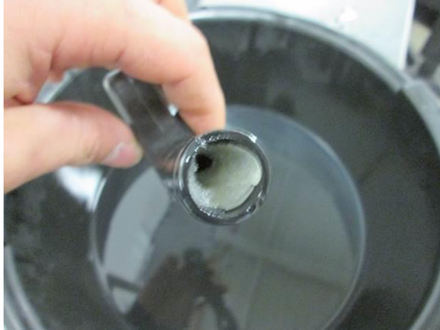
Fig.5: Cold-Weather Operation: Ice Plugging On Oil Breather Tube (Typical)
