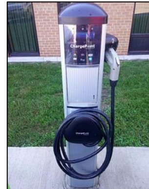
Electric car charging station Source: www.choosecornwall.ca
