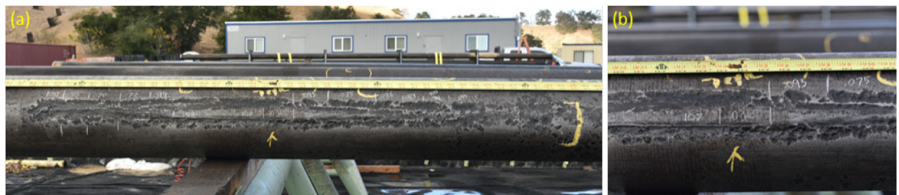
Figure 32: Pipe Body Corrosion on C020
