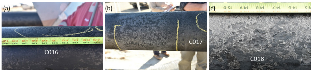
Figure 30: Pipe Body Corrosion on (a) C016, (b) C017, and (c) C018
