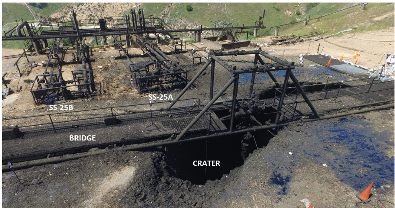
Figure 17: SS-25 Well Site West View Aerial Photograph Post Blowout Taken on April 01, 2016
