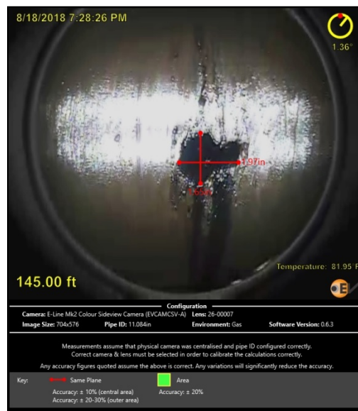
Figure 108: Picture of Hole in 11 3/4 in. Casing with Dimensions from Video Imaging at 145 ft
