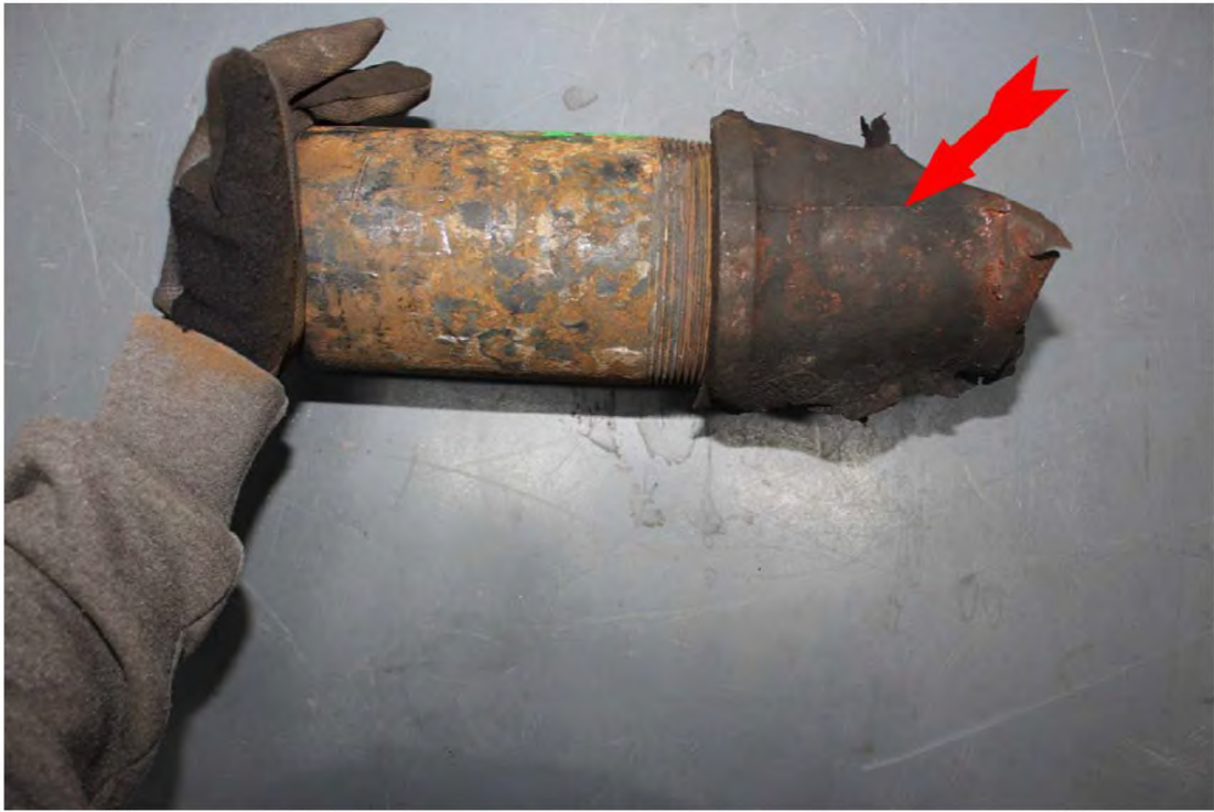
Figure 8 Corroded 4"x2"x4" Reducing Tee attached to 4-inch threaded pipe
