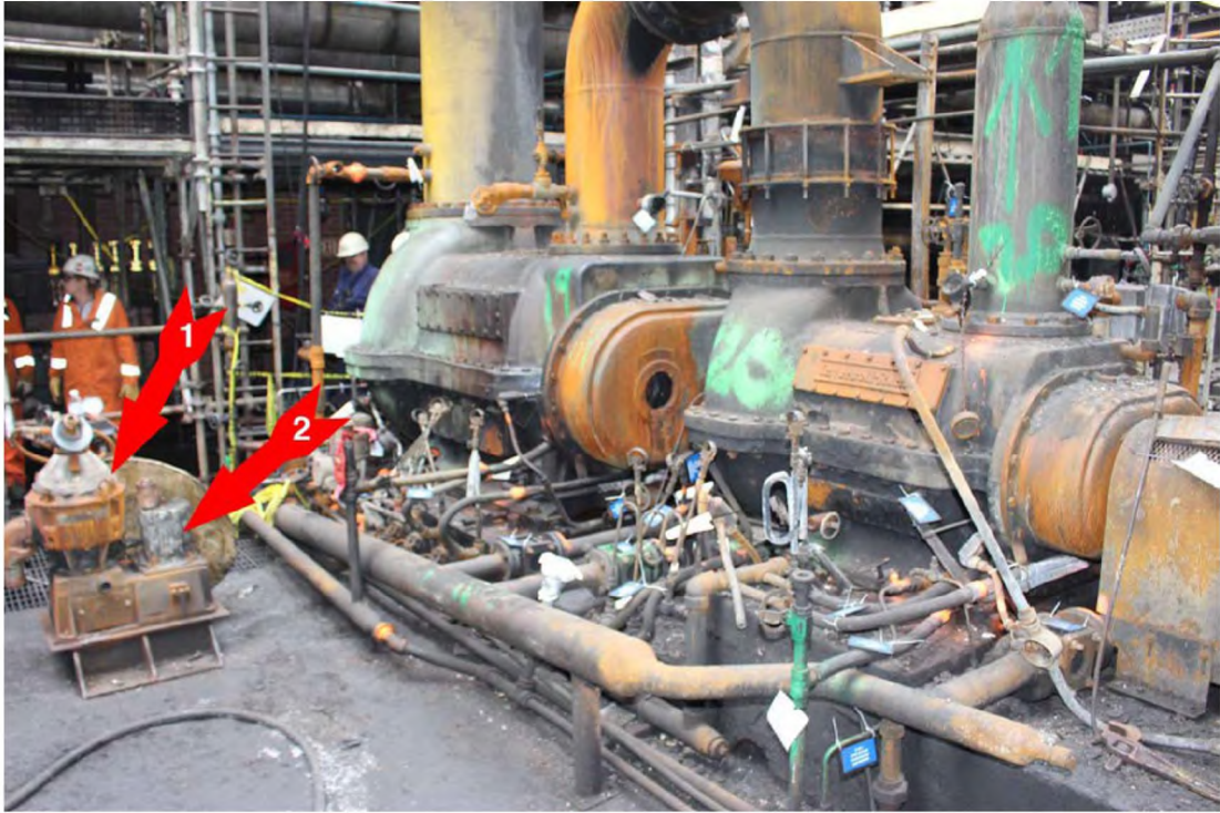
Figure 3 Centrifuge near C-521
