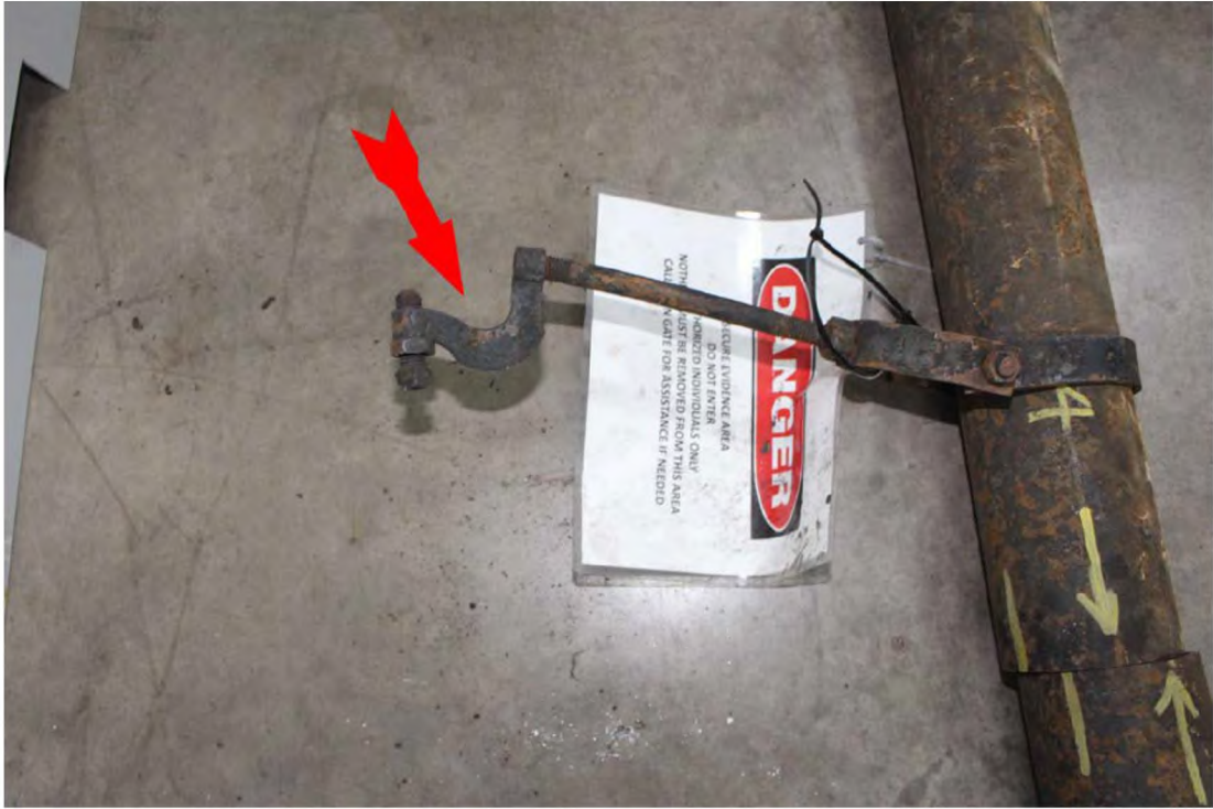
Figure 5 Overload deformation to hanger – Pipe Section “E”
