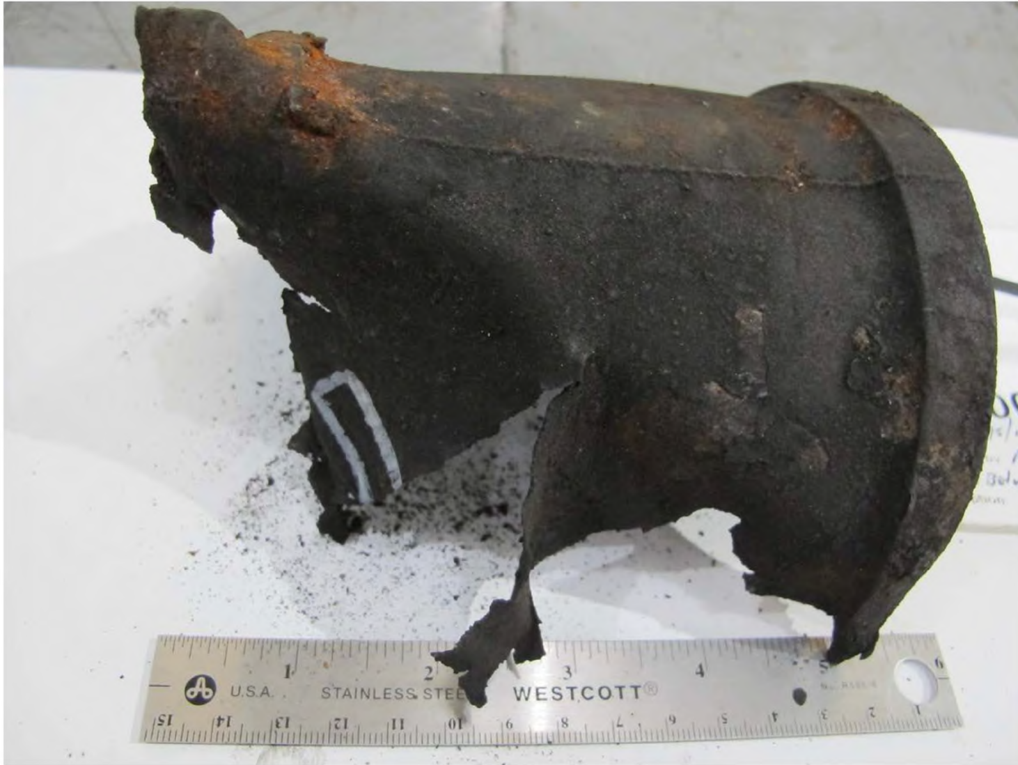
Photograph 16 – 4"x2"x4" Reducing Tee
