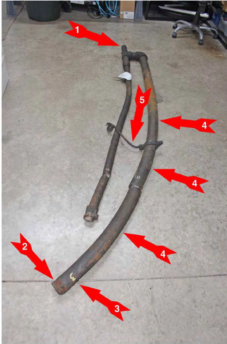
Figure 1 Pipe Section "C" Arrow 1 Pipe Section "B" attachment point Arrow 2 Pipe Section "D" attachment point Arrow 3 Impact location Arrows 4 Deformation due to heat Arrow 5 Deformation of hanger due to heat
