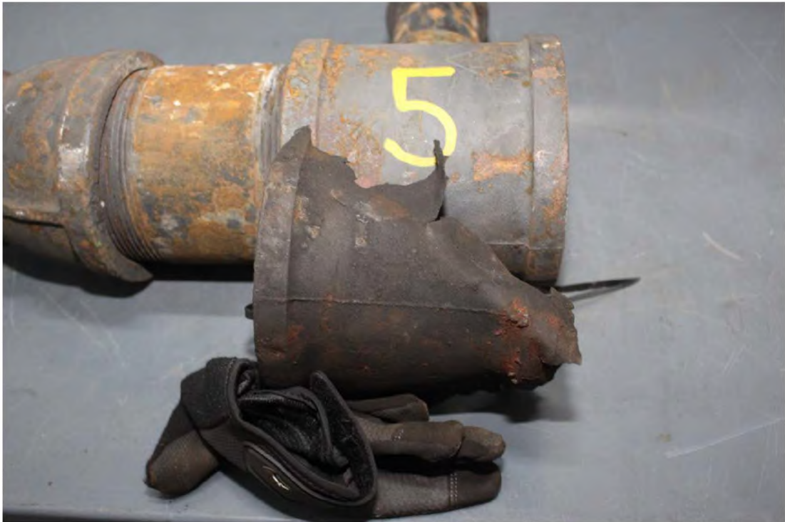
Figure 9 Corroded 4"x2"x4" Reducing Tee placed next to 4"x2"x4" reducing tee comprising Pipe Section "E"
