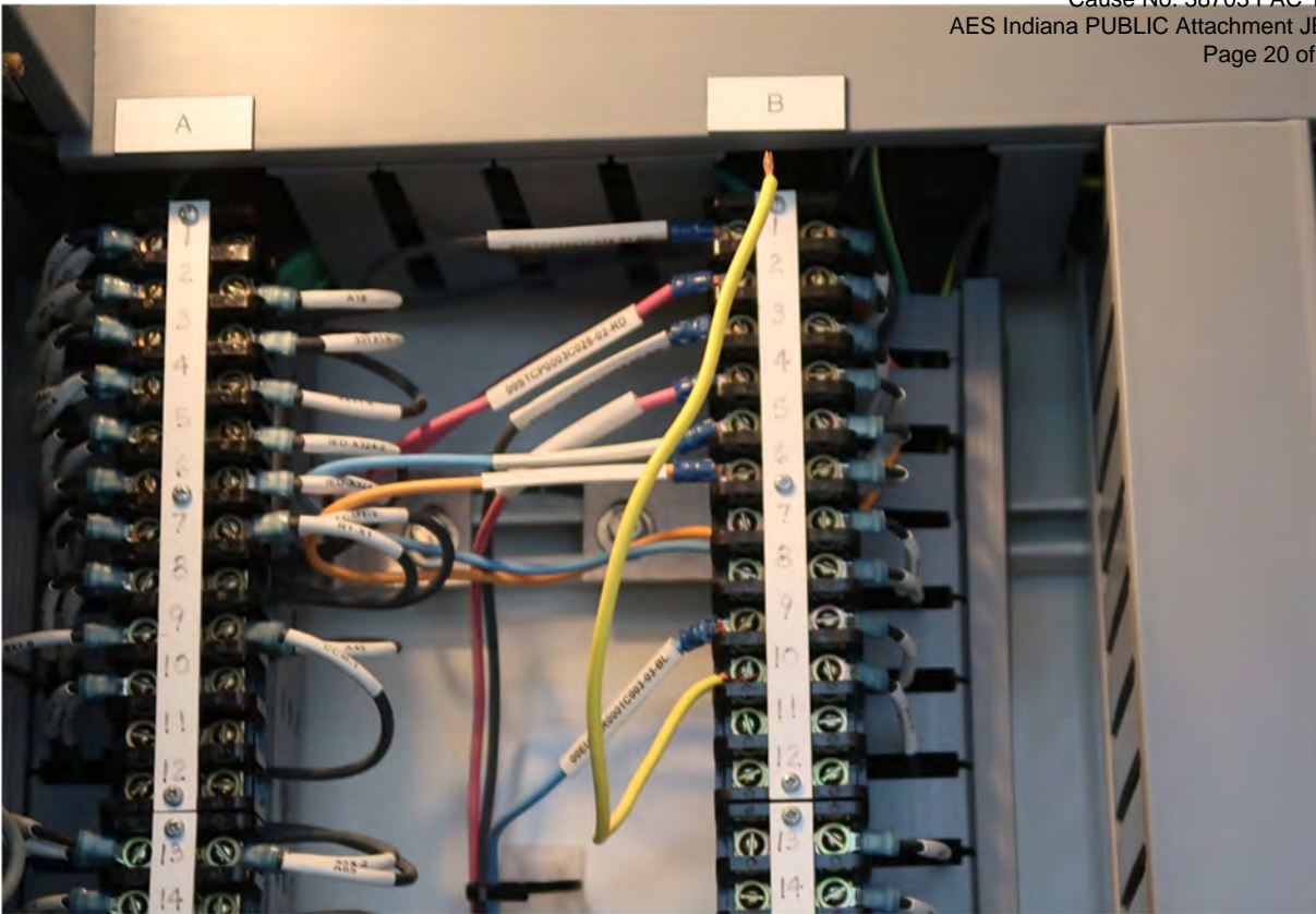
Photograph 3, Loose yellow jumper wire in STG 52G Breaker Cabinet
