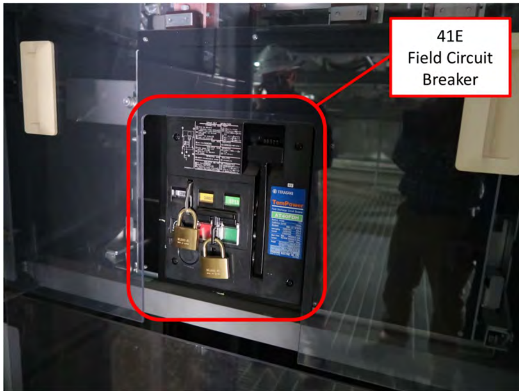
Photograph 2, STG 41E Breaker Location
