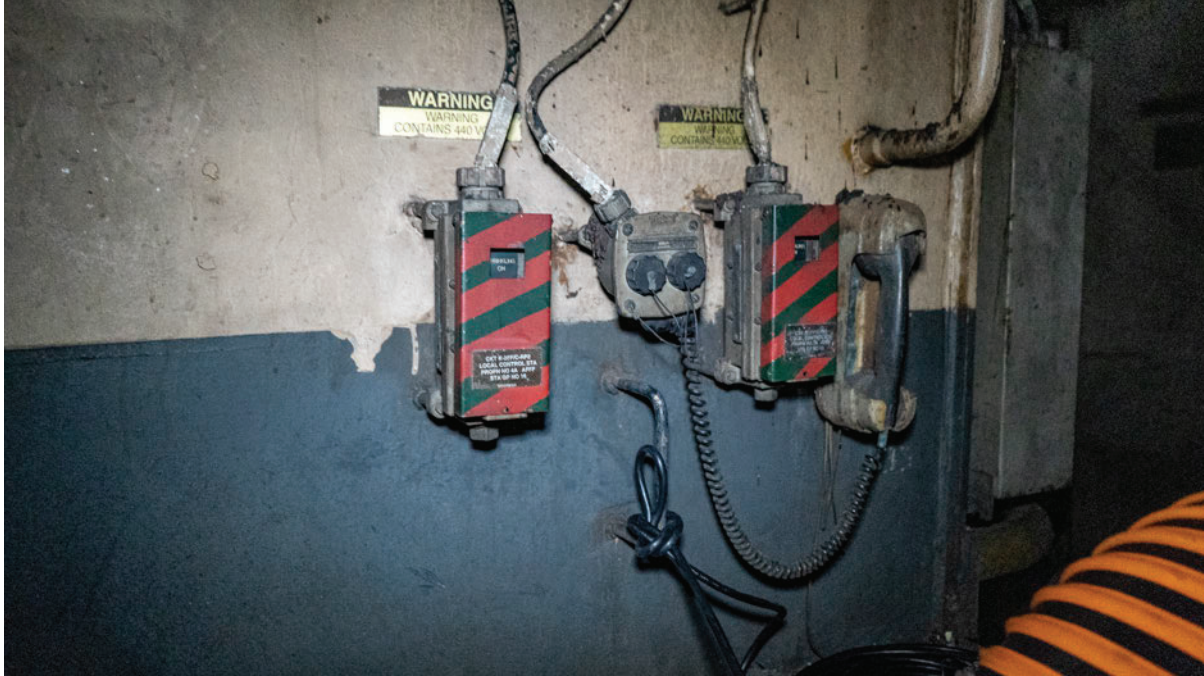
Figure 31, Still photo of AFFF push-buttons for sprinkler groups 15 and 16 serving Lower V with covers closed (16 on left; 15 on right). These push-buttons are in Upper V amidships.
