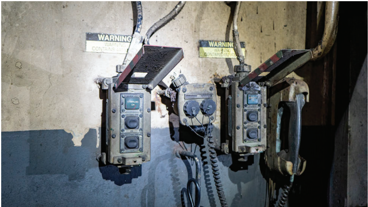
Figure 32, Still photo of AFFF push-buttons for sprinkler groups 15 and 16 serving Lower V with covers open (16 on left; 15 on right). These push-buttons are in Upper V amidships.
