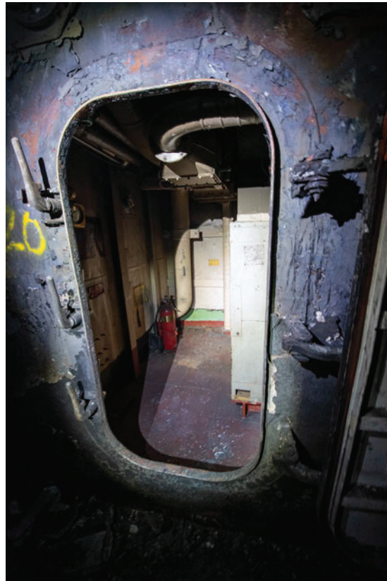
Figure 47 shows two compartments separated by a closed hatch. One compartment was severely damaged, while the adjacent compartment suffered minor damage.
