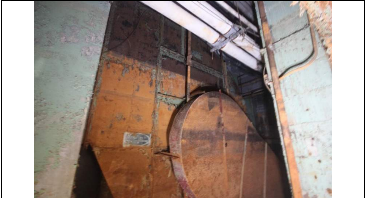
Photo 4: Fan Room in Basement
