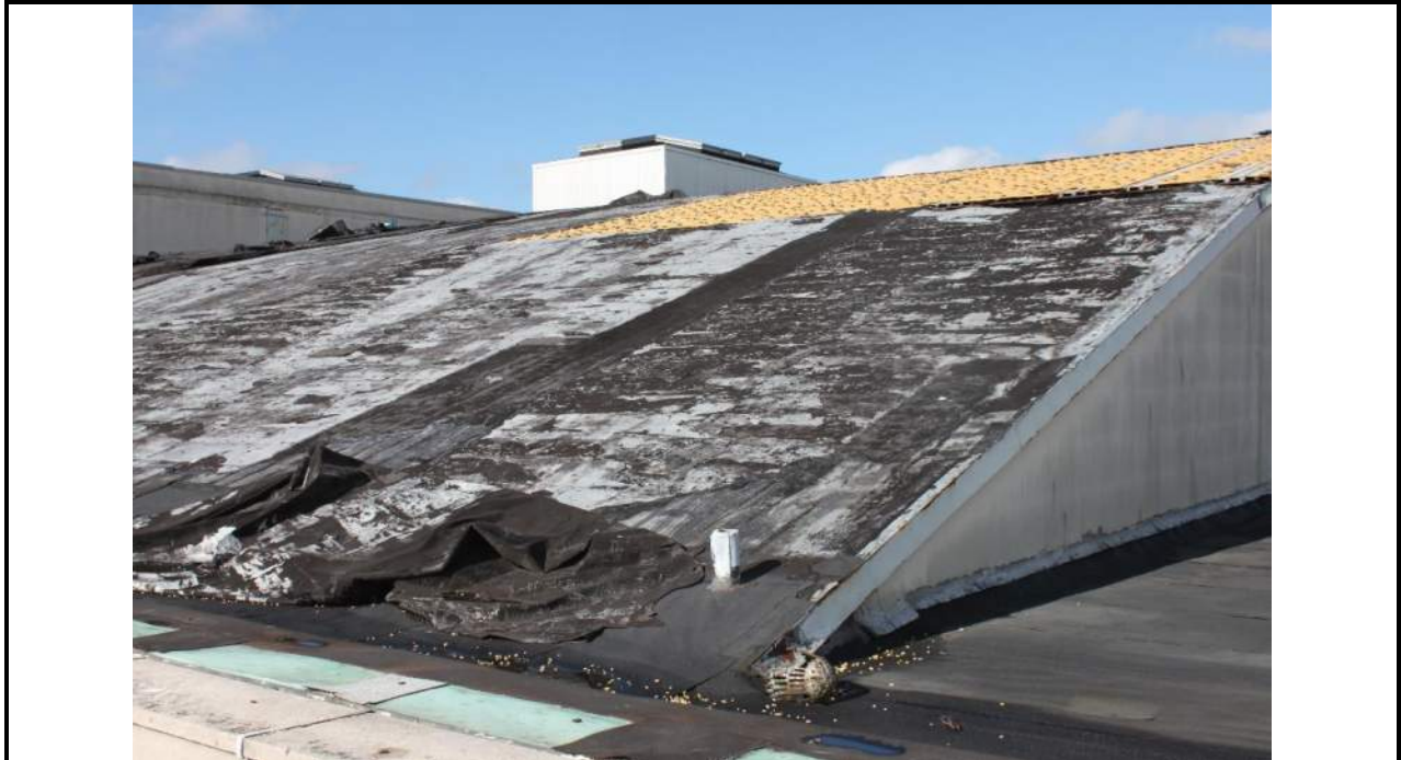
Photo 20: Auditorium Room Damage
