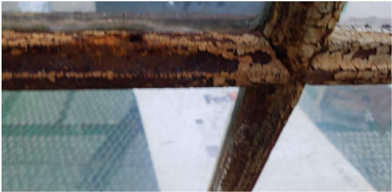
Photo 95: Window Type C that was Previously Removed by Others. Sitting atop Roof E.
