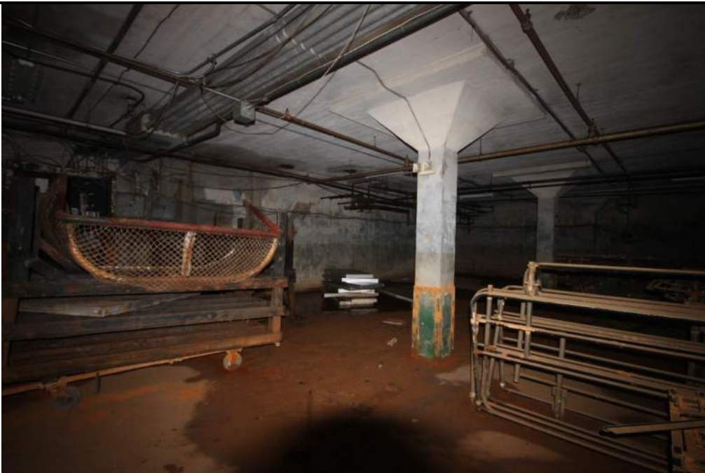
Photo 2: Basement (Area below Roof Leaks)
