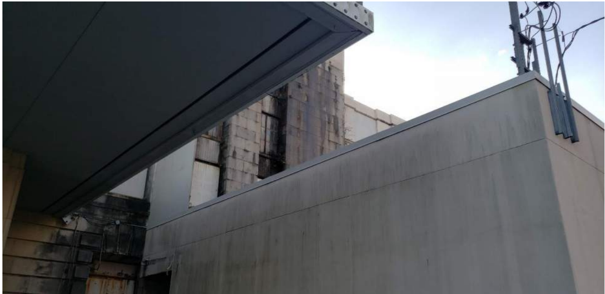
Photo 100: Damaged Limestone Below Hole in Roof.
