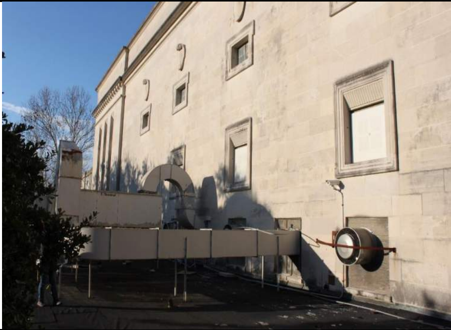
Photo 29: Type H: At both St. Peter and St. Ann Street sides “Masonry Opng. Steel Casement Opng. Out”
