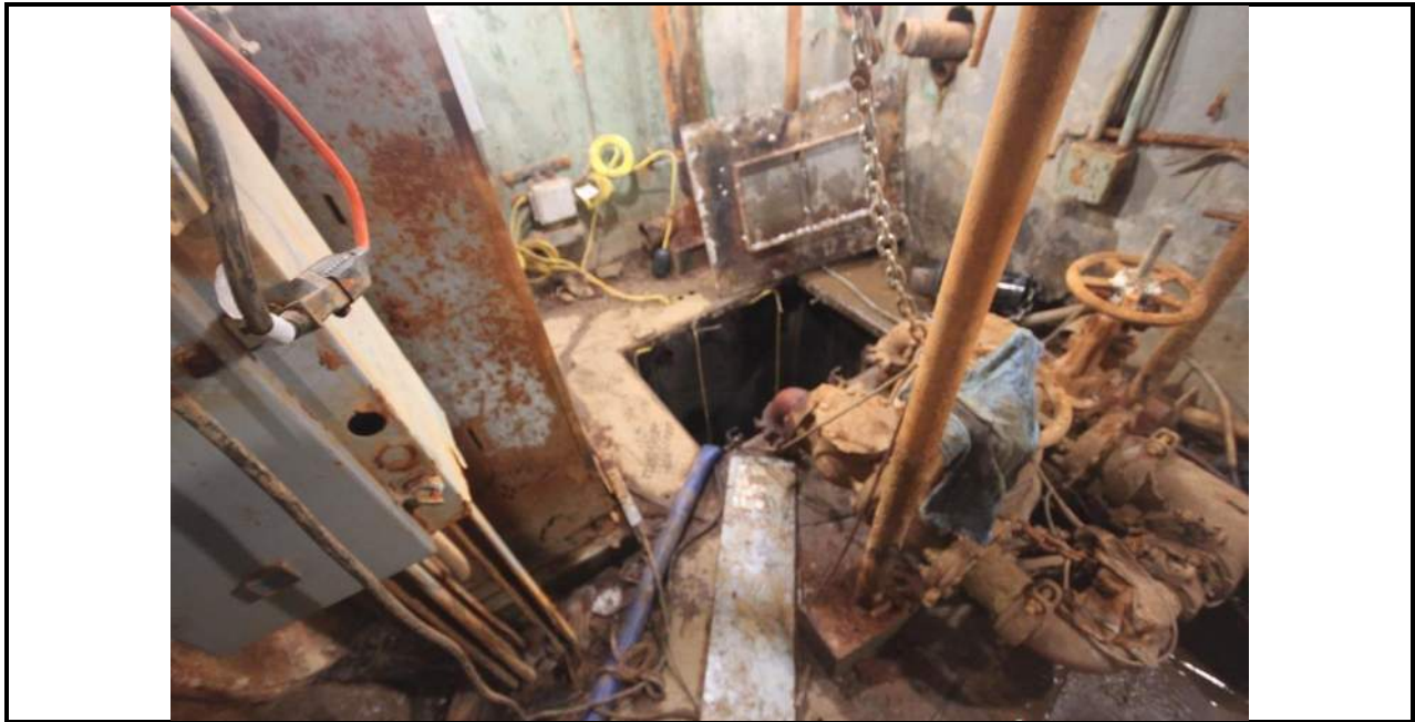
Photo 3: Sump Pump in Basement
