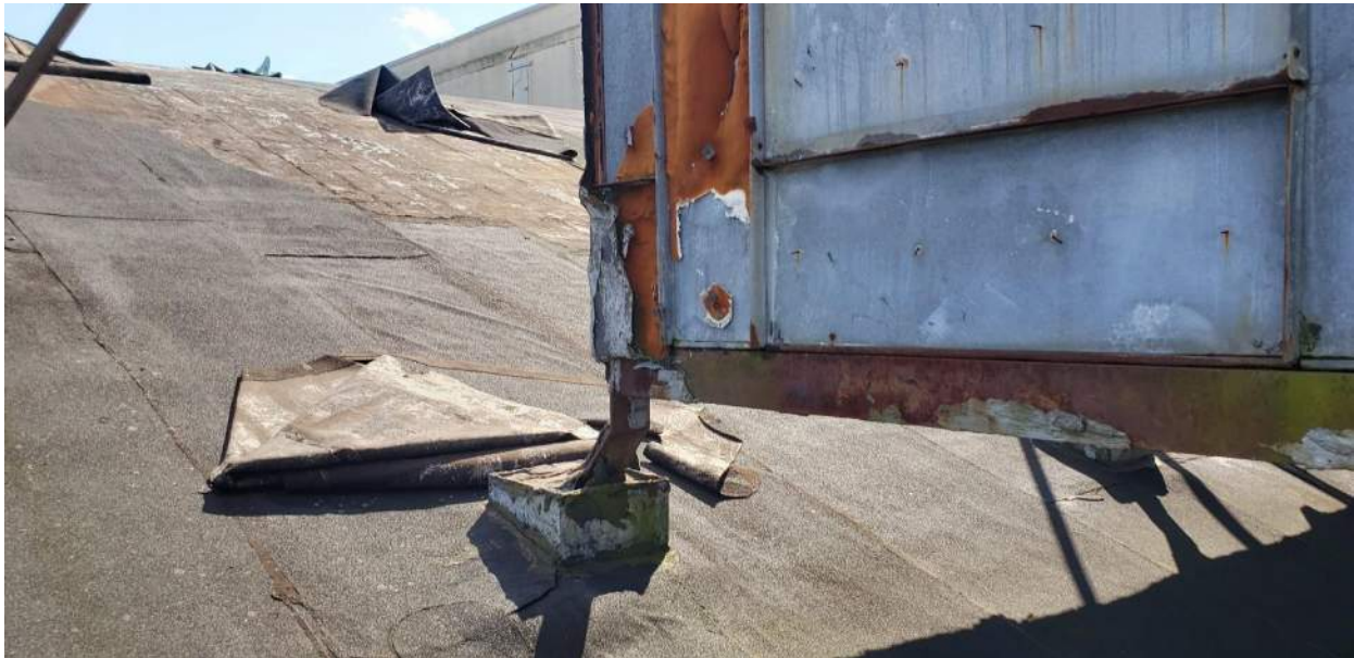
Photo 94: Pitch Pan Attachment for HVAC System.
