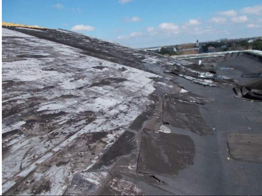
Photo 65: Damaged Barrel Vault Roof
