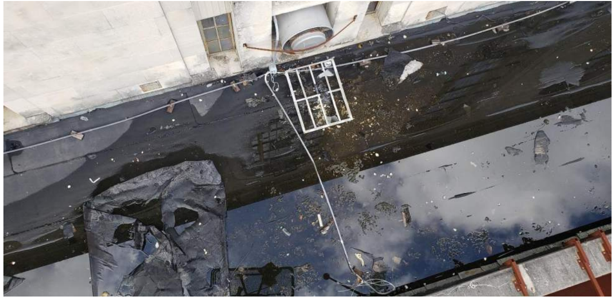
Photo 35: Roof Section C. The drains are clogged, and the roof is ponding.
