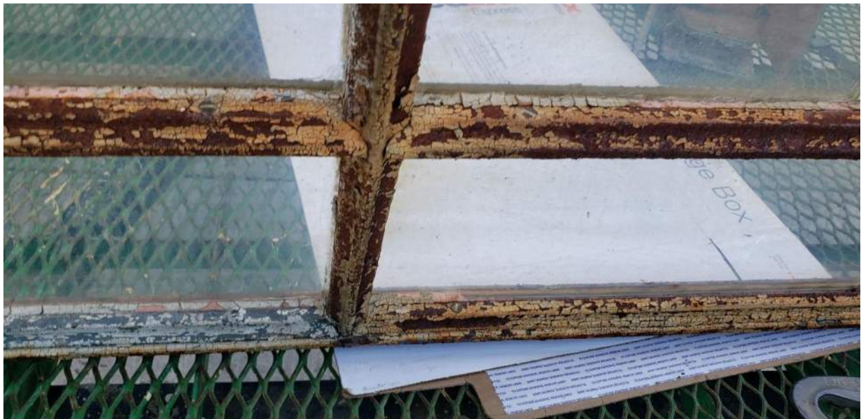
Photo 96: Window Type C that was Previously Removed by Others. Sitting atop Roof E.
