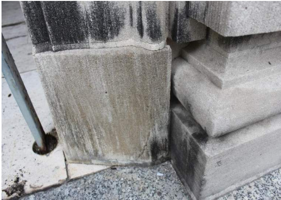
Photo 13: Cracked Mortar Joint and Limestone at Covered Porch
