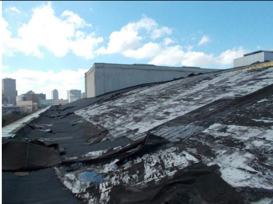
Photo 58: Damaged Roof of Barrel Vault along St. Ann
