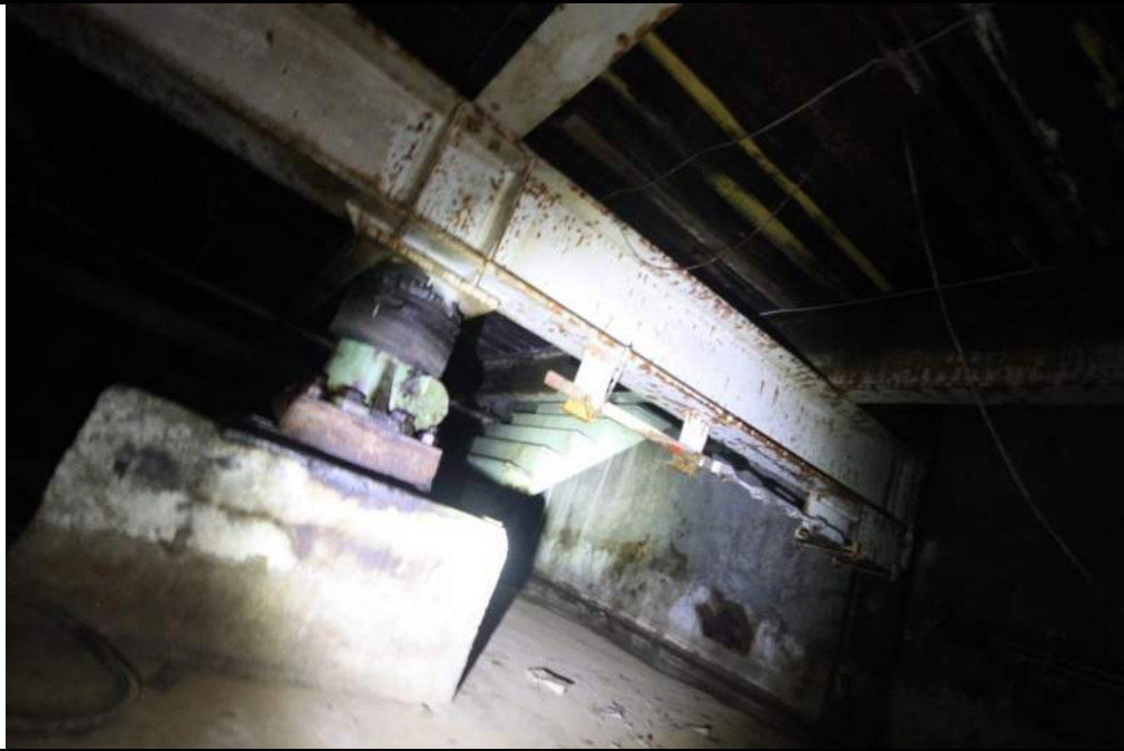
Photo 5: Gear-Driven Jack and Beam Supporting Operable Stage
