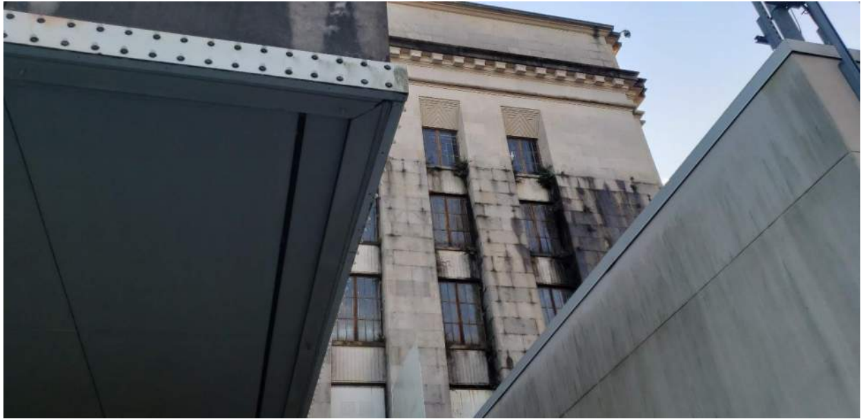
Photo 99: Damaged Limestone Below Hole in Roof.
