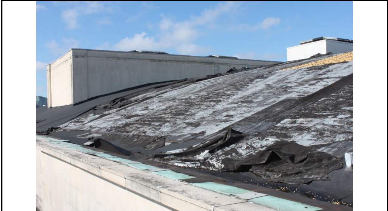
Photo 8: Valley in Between the Coping and the End of the Barrel Vault Roof
