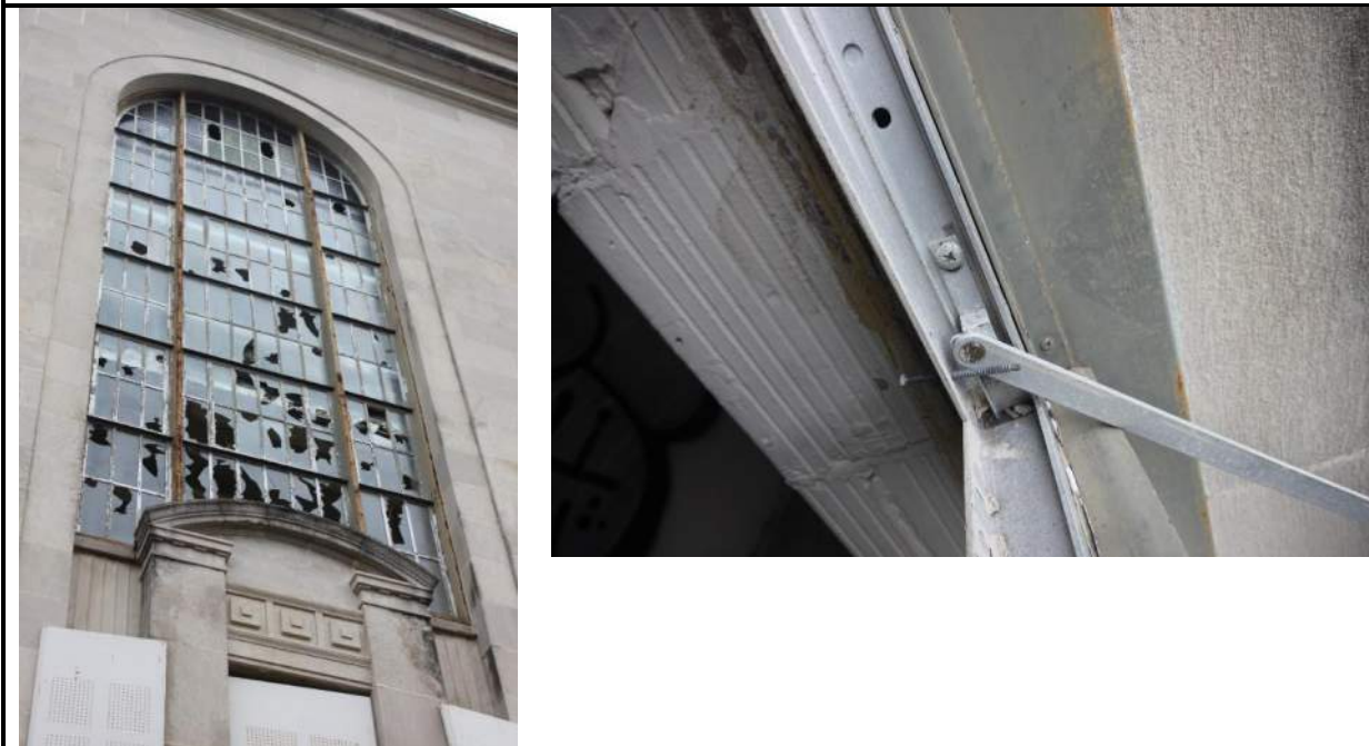
Photo 22: Type A “Circular Headed Masonry Openings – Steel (replaced with Aluminum) Sash and Frame”
