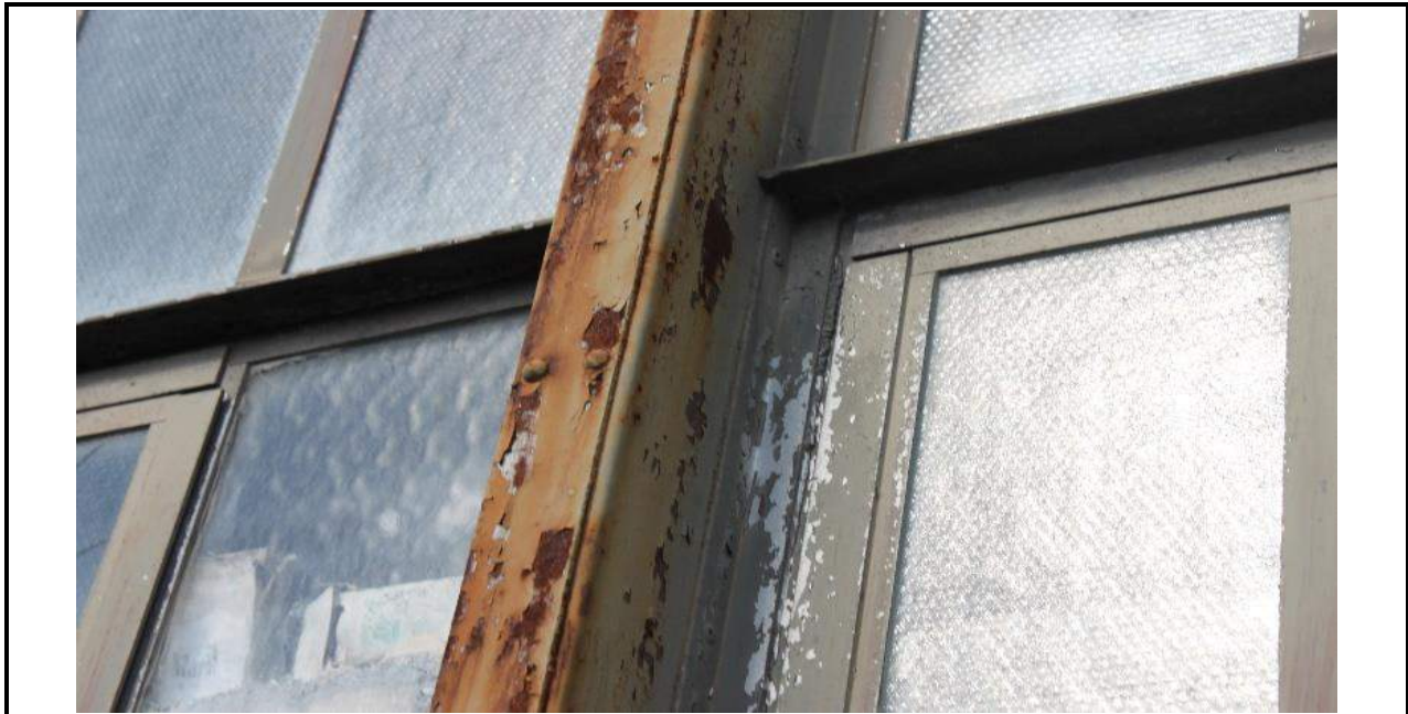
Photo 23: Type A “Circular Headed Masonry Openings – Steel (replaced with Aluminum) Sash and Frame”
