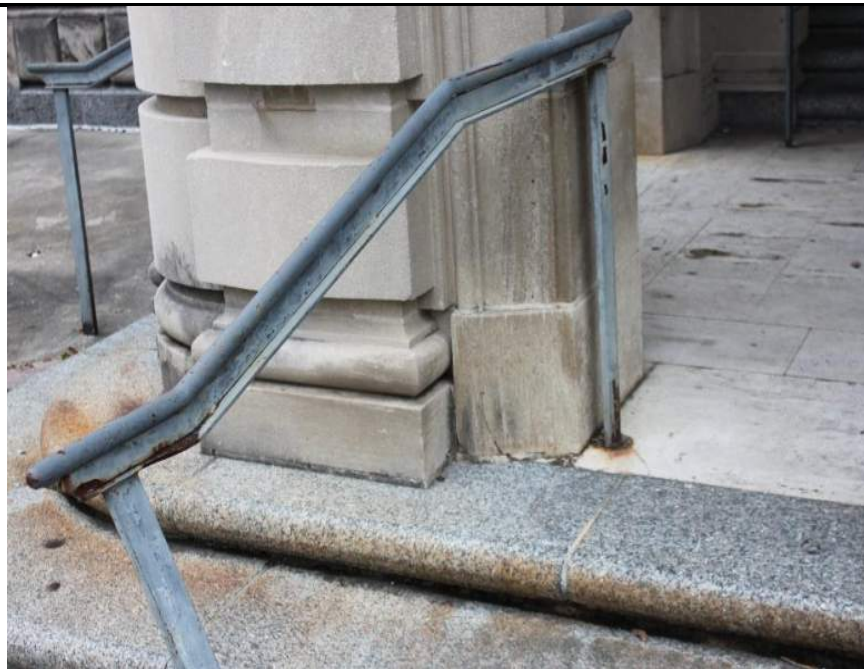
Photo 14: Cracked Mortar Joint and Limestone at Covered Porch
