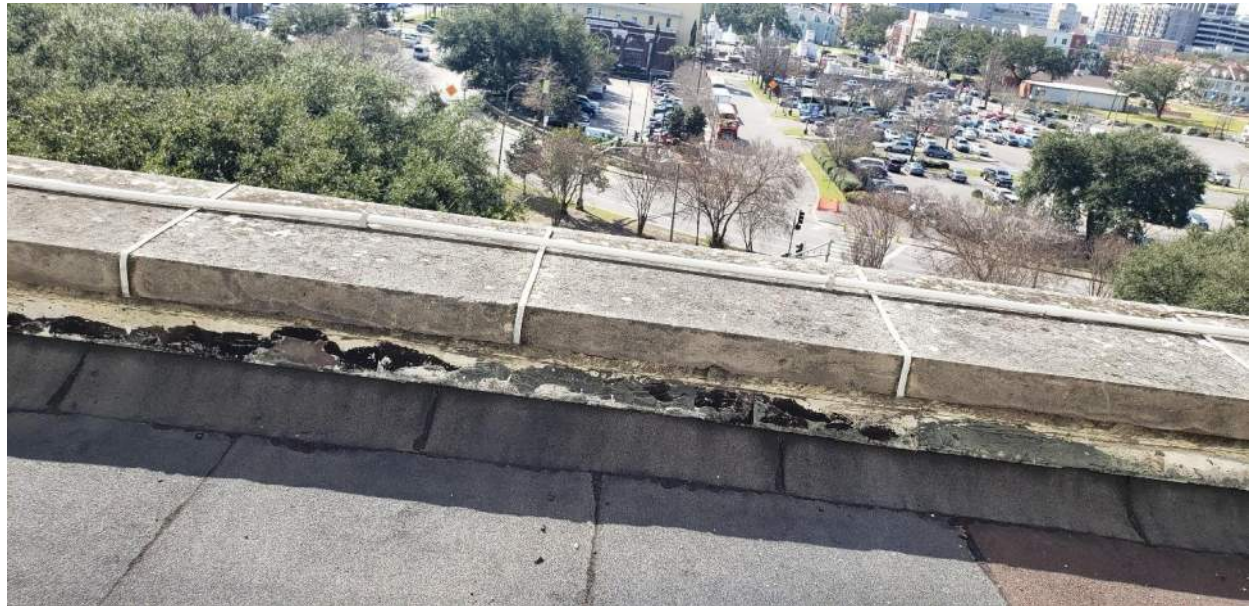
Photo 50: Missing Copper Flashing Along St. Peter
