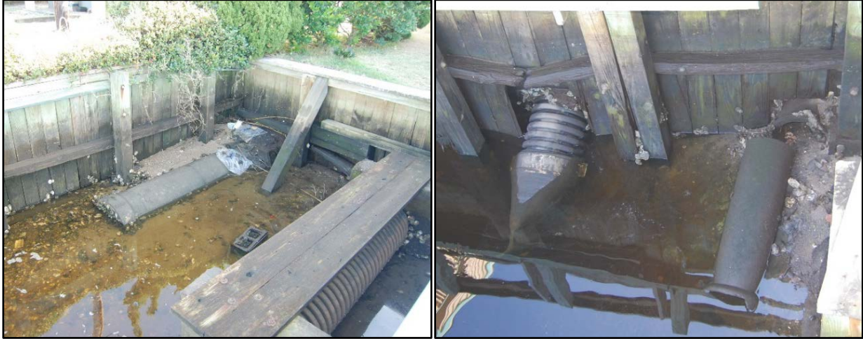
Figure 23. Abandoned Stormwater Outfall Pipes. (left: 909 Canal Drive, right: Street End at Seagull Lane and Canal Drive)
