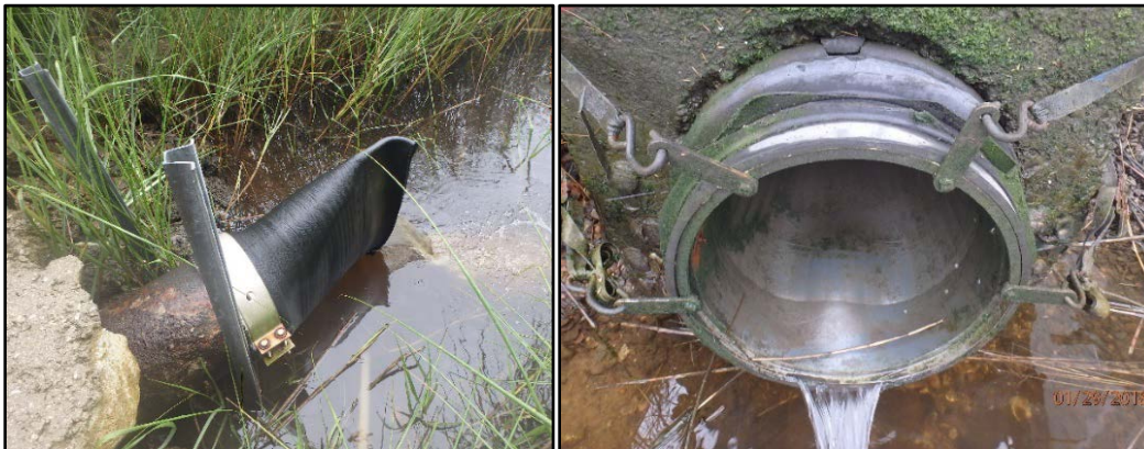
Figure 22. Examples of Functioning Backflow Prevention Devices Currently Installed. (left: recurved duckbill valve, right: WaStop® Inline Check Valve)
