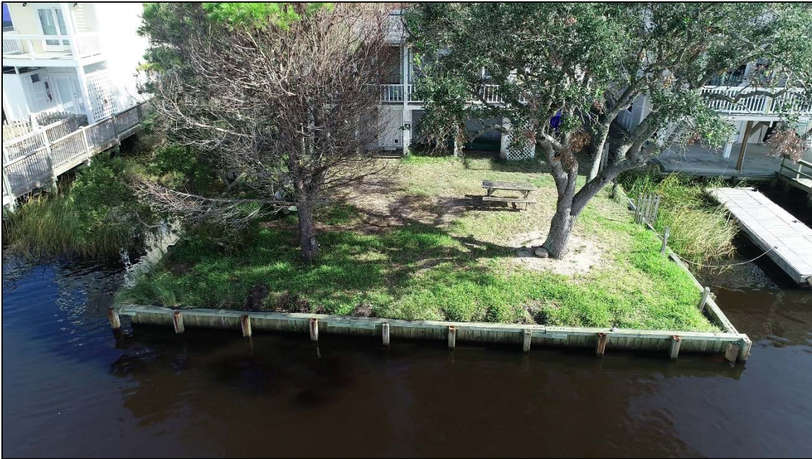
Figure 15. Screenshots from the Drone Video showing a portion of the marina bulkhead along Canal Drive and the bulkhead at 1313 Canal Drive.
