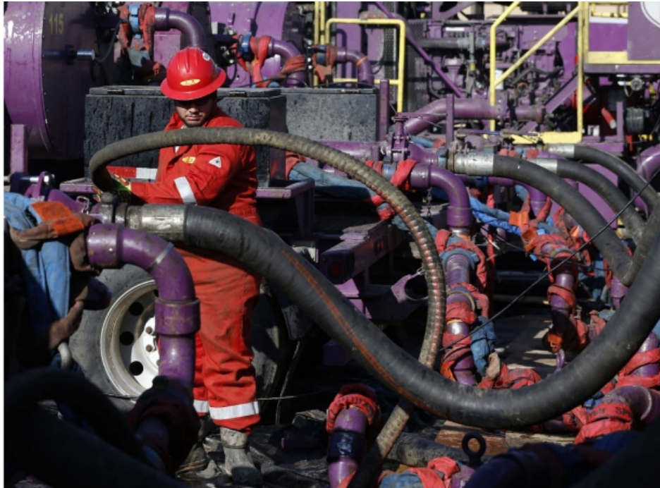
Figure 5-8. A worker adjusts hoses at a hydraulic fracturing site near Mead, Colorado.
