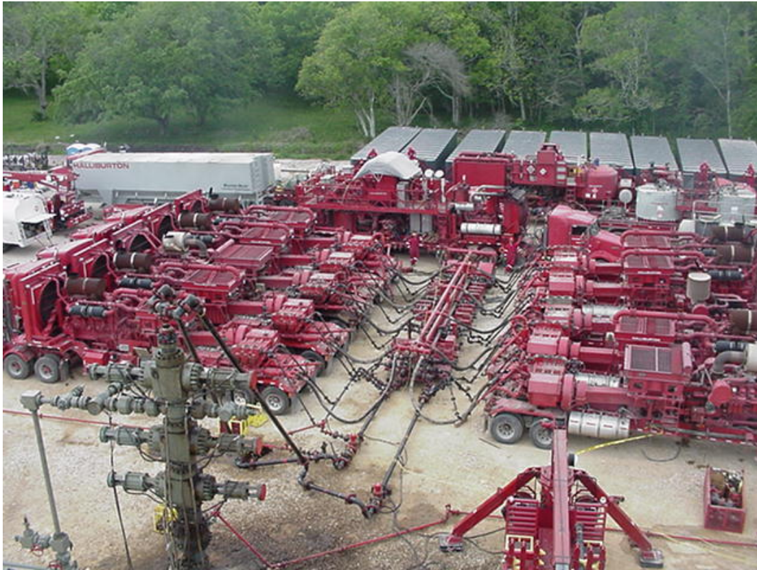
Figure 5-10. High-pressure pumps on either side of the manifold.
