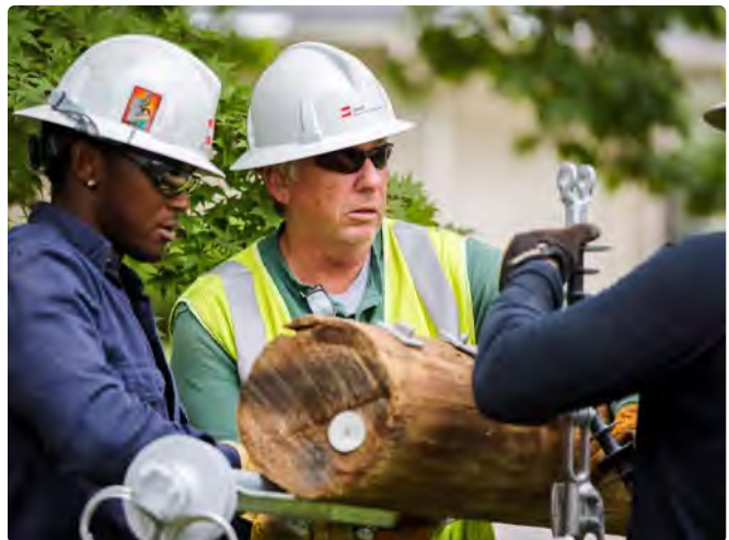
Making investments to upgrade and replace our aging transmission and distribution grid is essential to maintaining the highest levels of reliability and resiliency.
