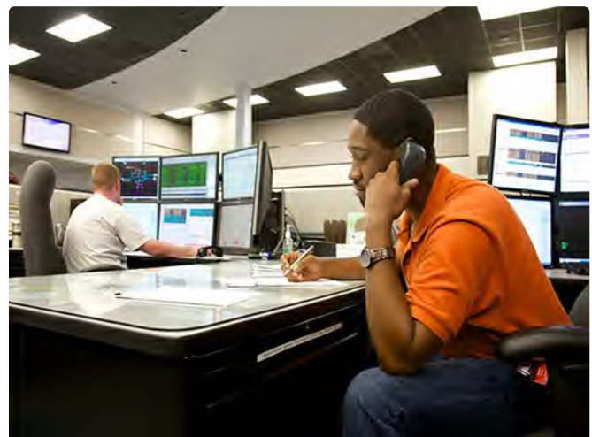
Our Smart Grid Command Center offers 24/7 service monitoring for our entire network communications between AMI, DACR, VVO/CVR and underground network vaults.
