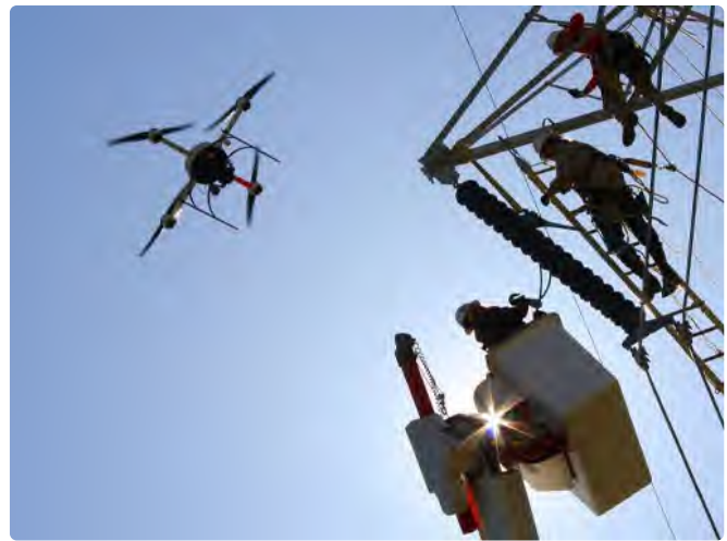
Drones are an effective means of inspecting power lines for regular maintenance and to survey damage after storms.
