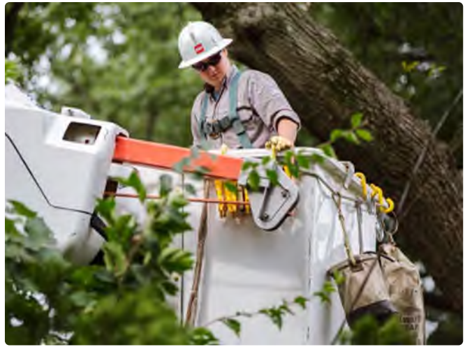
Outages and equipment failures related to overgrown and/or fallen vegetation – trees and other vegetation – are among the biggest challenges to AEP's service reliability.
