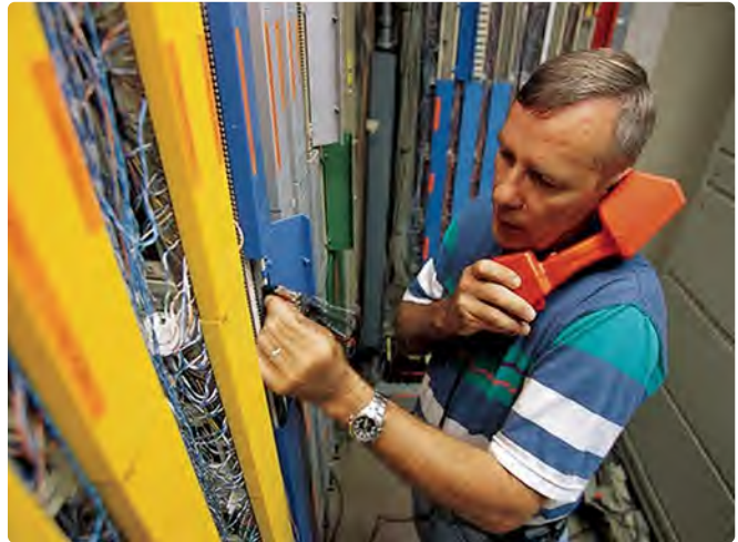
Having the proper infrastructure in place to support our evolving telecommunication needs to meet both current and future operational demands is imperative.
