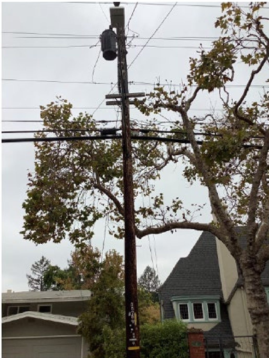
Figure 8. Oakland K-1101 defect #2
