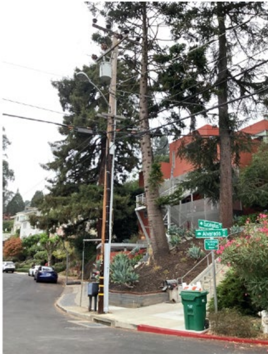
Figure 7. Oakland K-1101 defect #1
