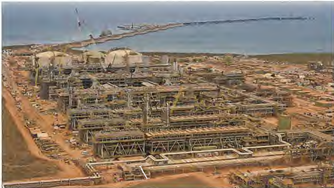
March 2016: Aerial view of the gas processing plant site looking southeast. The three carbon dioxide compressor modules can be seen in the lower left of the photo.
