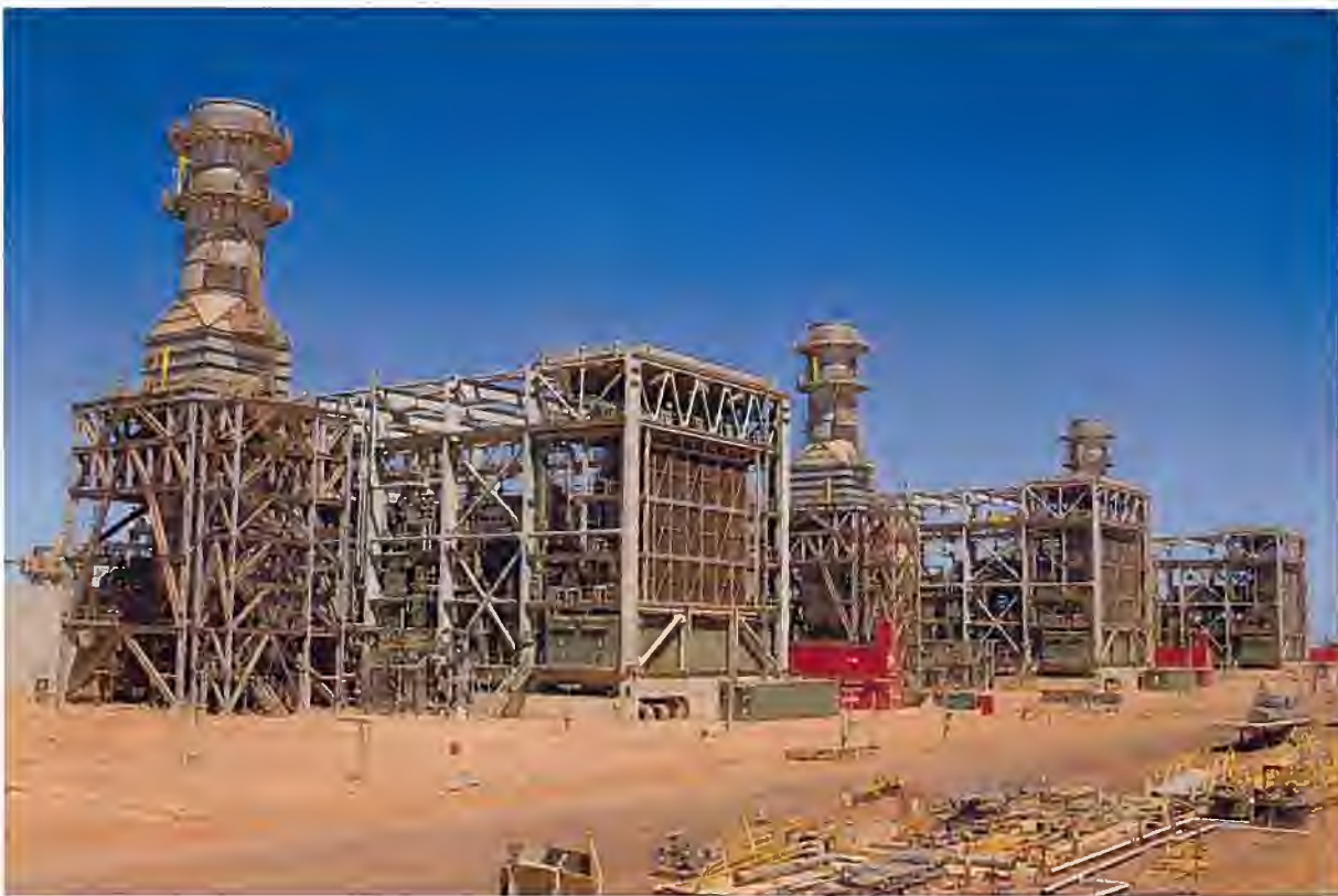
March 2016: Three of the five gas turbine generators used to provide electrical power for the gas processing facility.
