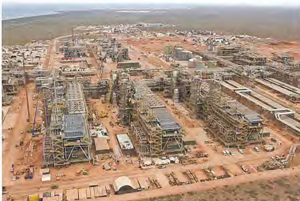
March 2016; Aerial view looking south showing the three carbon dioxide compressor modules in the foreground, the three carbon dioxide removal units (acid gas removal units) in the middle ground and the five gas turbine generators in the background. The gas inlet receiving facilities are shown in the right of this photo.
