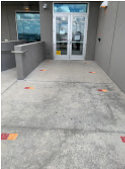
Marked Floors.JPG 4247K
