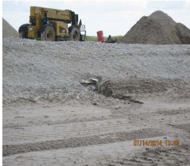
Figure 2: Apparent Berm Fluid Discharge Pipe with Erosional Gully
