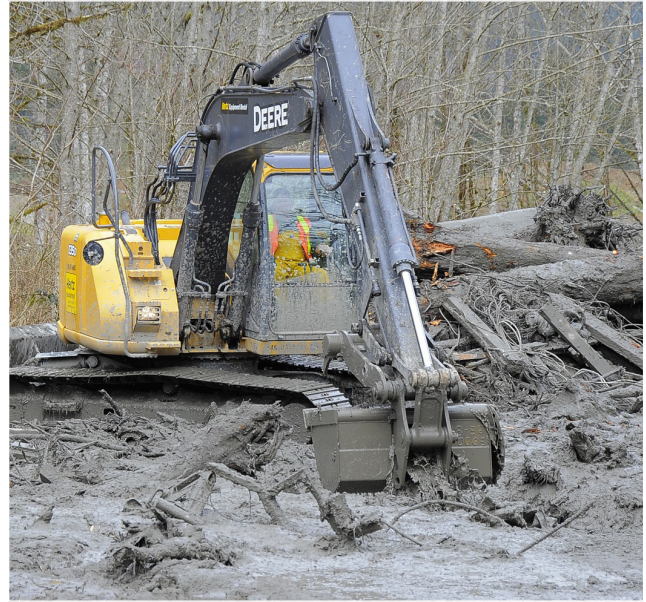
An Excavator Working in the Debris Field near Oso. Photo courtesy of WSP. Flickr/Snohomish County - CC: BY-NC-ND 2.0
