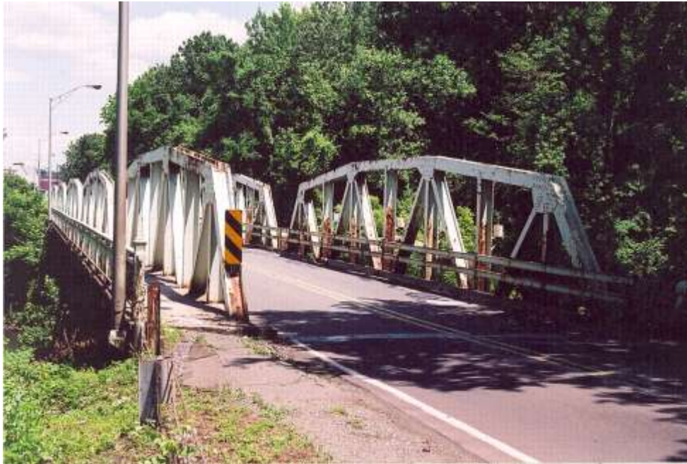
Keim Street Bridge, a significant entry point to the borough, is in need of repair. (Photo Credit: Raymond Klein at www.bridgehunter.com )
