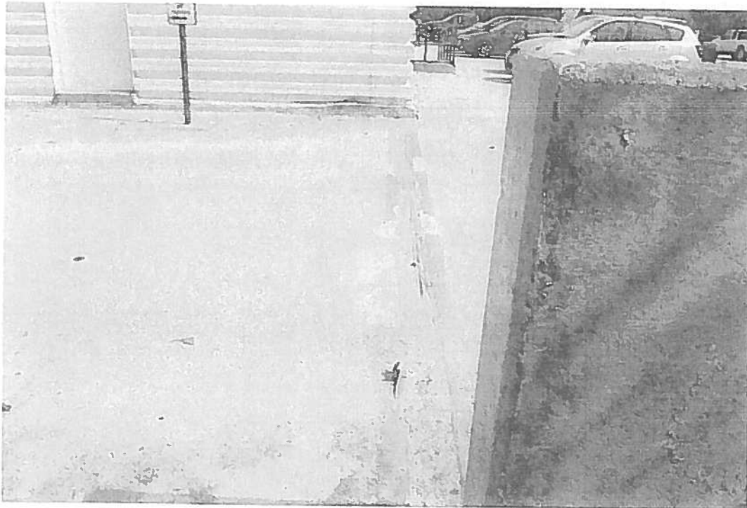
Picture 4: Major expansion joint at SW corner of Algo Inn. Leakage in Library below.
