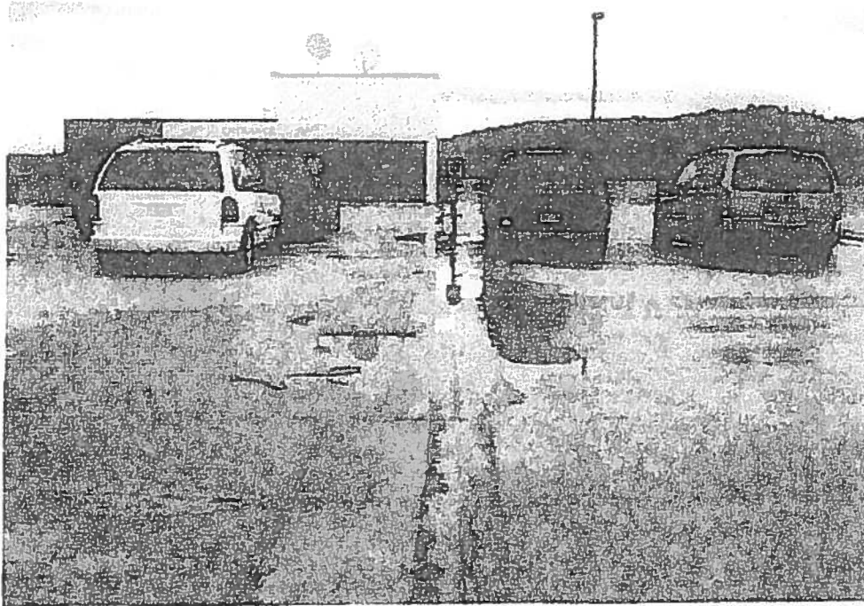
Picture 1: Grid Line 5 water ponding on parking deck despite the design in structure slope to drains on Grid Line 4 ponding appears to be due to positive camber of precast slabs.
