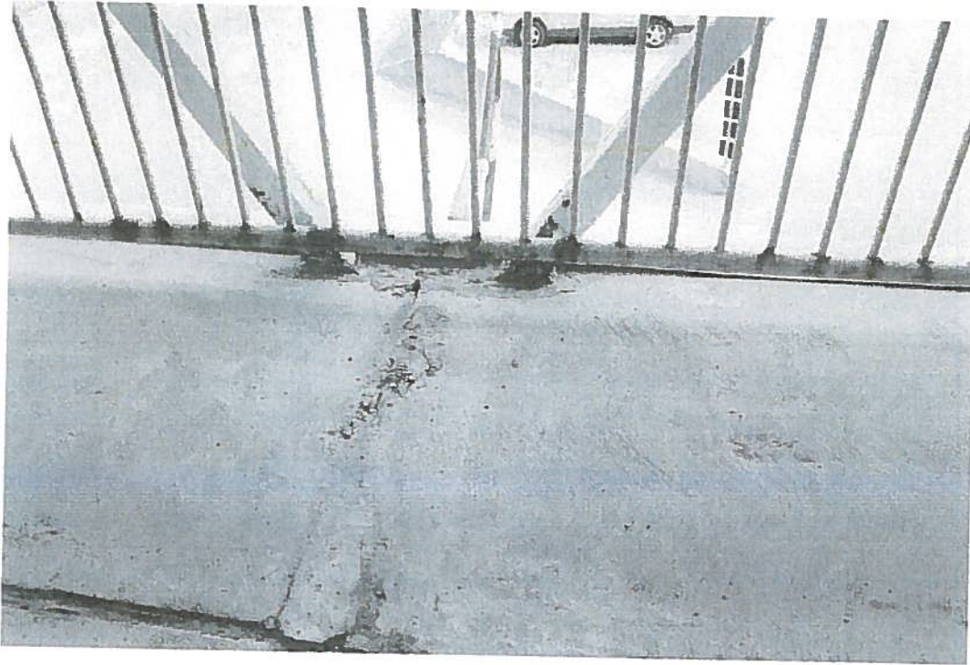
Picture 11: Rusting steel at base of diagonal HSS members of open walkway.
