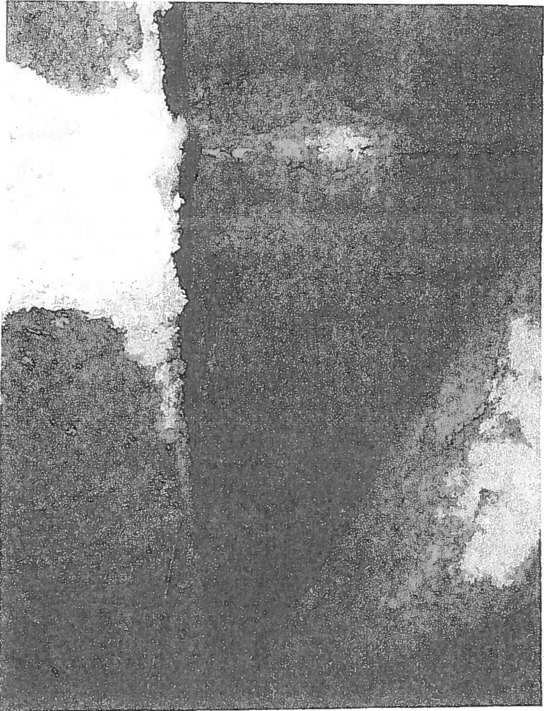
Picture 6: Exposed underside of right parking area. Precast slabs right of beam leakage location at ticket kiosk in Mall, Grid Line 16 efforescence stain at precast slab joints and fire proofing has fallen off bottom flange of steel support beam.
