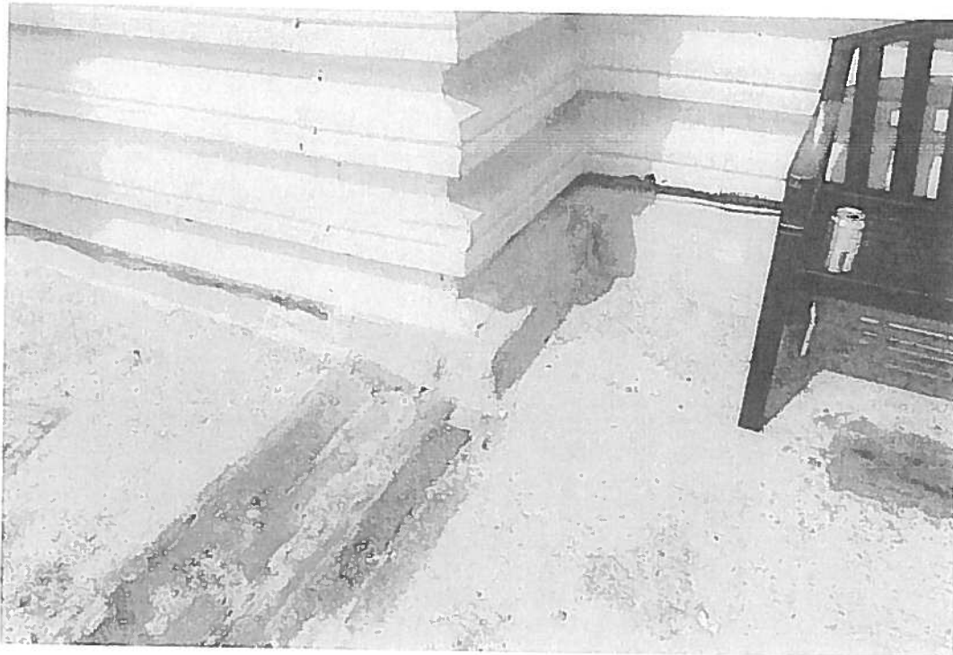
Picture 6: Expansion joint at SE corner of Algo Inn leaks in lottery ticket booth mall below.
