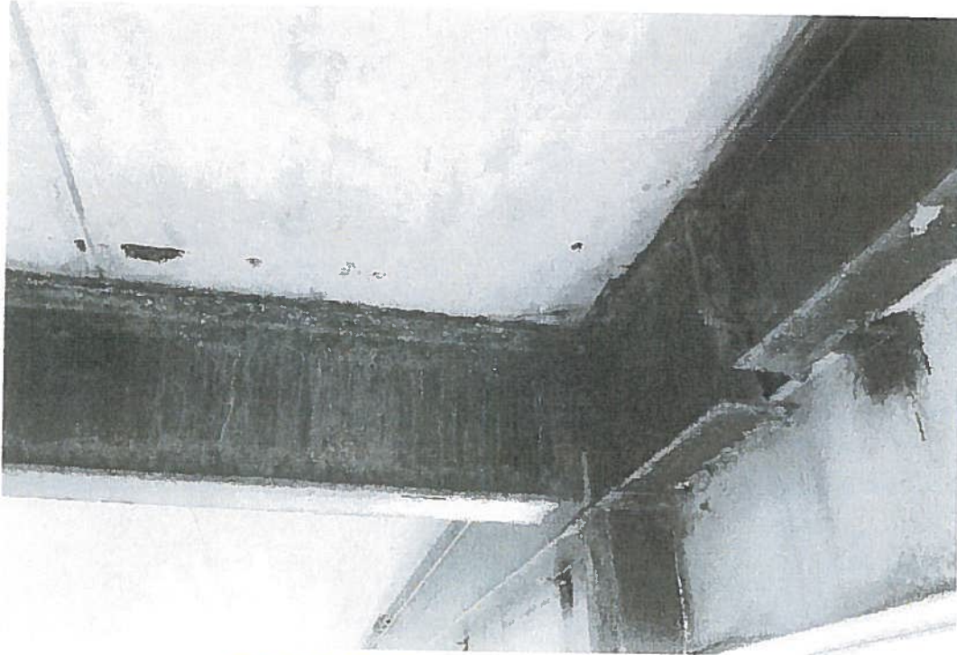
Picture 12: Rusting steel U/S of deck of open walkway.
