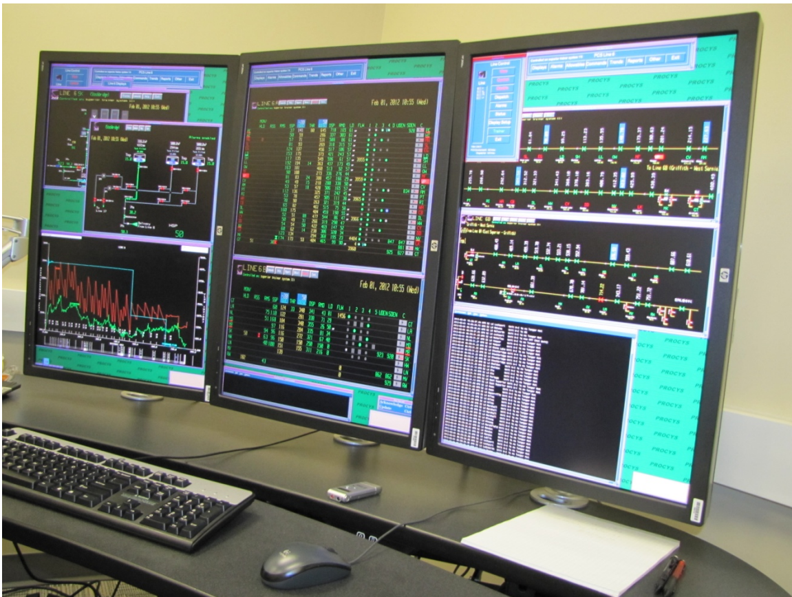
Figure 2: Simulated Training Console; operations SCADA screens displaying simulated Line 6A & 6B on February 1, 2012, Source: NTSB. See Appendix 2
