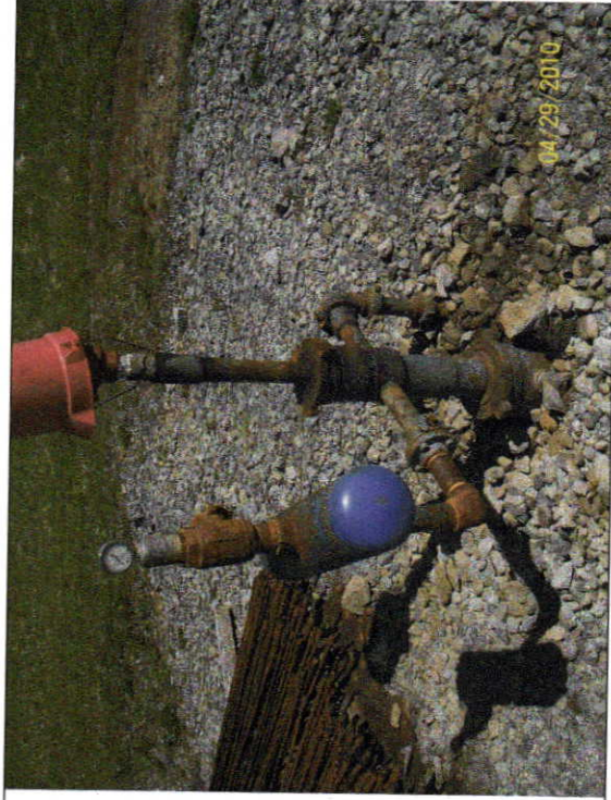
Caption: Well Head, note the lack of a tag on the well head.
