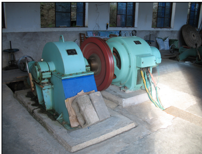
Fig. 6: SHP generator operating in Yunnan Province Source: Yunnan Digital Government
