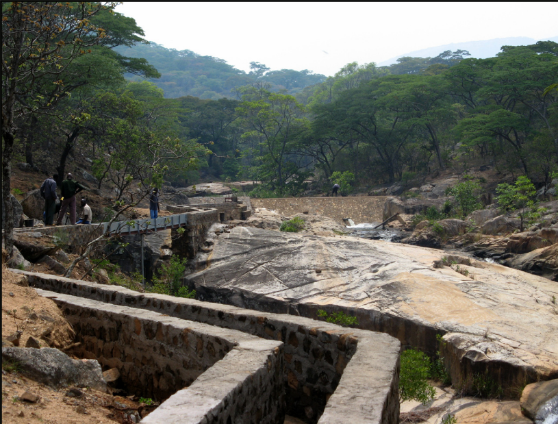
Fig. 15: Construction of the river diversion Dazi, near Nyanga Nation Park, Zimbabwe. The project was developed with the support of Practical Action. Source: Practical Action
