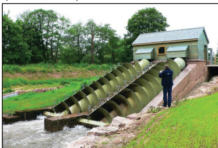
Fig. 8: An innovative Archimedean screw installed at an old mill site in the UK. While efficiency is slightly lower than regular turbines, the design allows fish of all sizes to pass unharmed through the slow moving screws Source: Engineering and Technology Magazine
