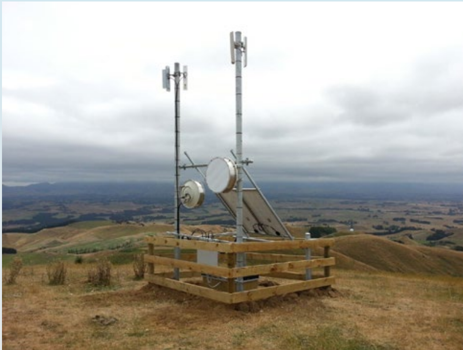
The new equipment installed for Sherwood School uses solar power
