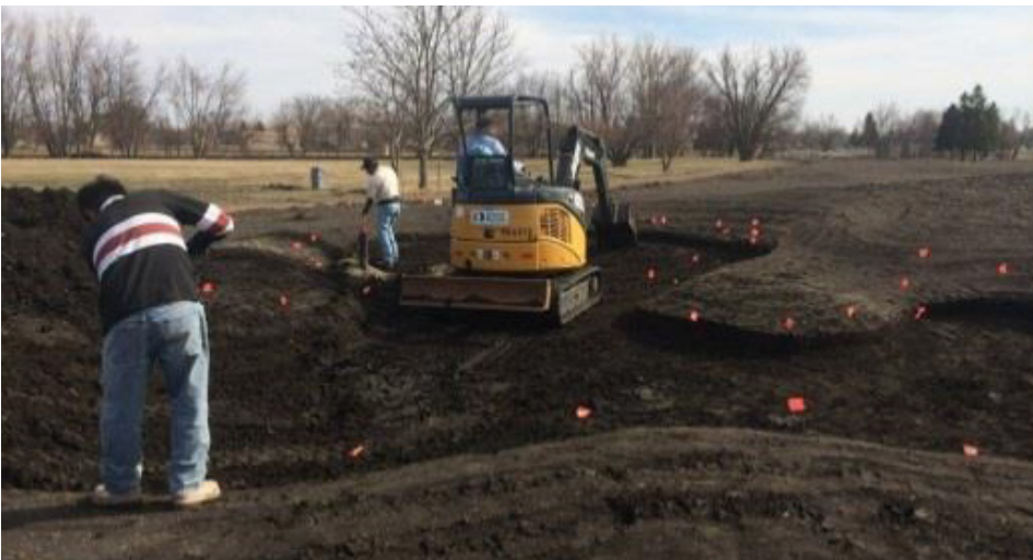
Workers build a new sand bunker to ensure safety of air space 734
