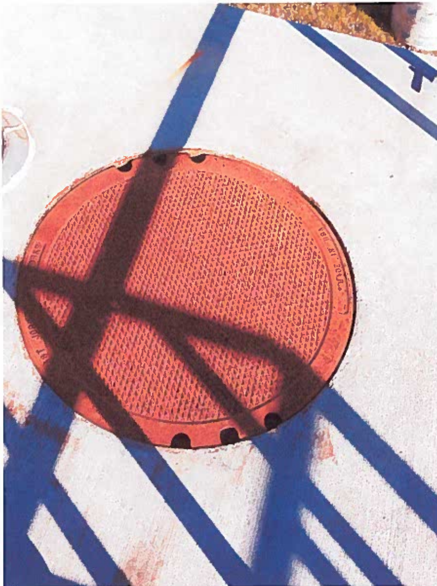
3 - Photo of junction box manhole cover unsealed
