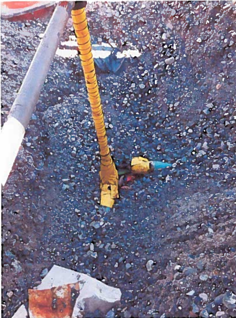
1 - Photo of disconnected sump pump effluent line
