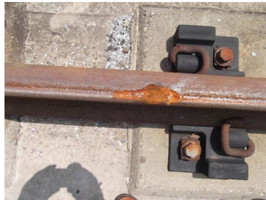
Figure 18 – Rail burn marks on the Danny Thomas Blvd. Bridge on the Madison Avenue Line
