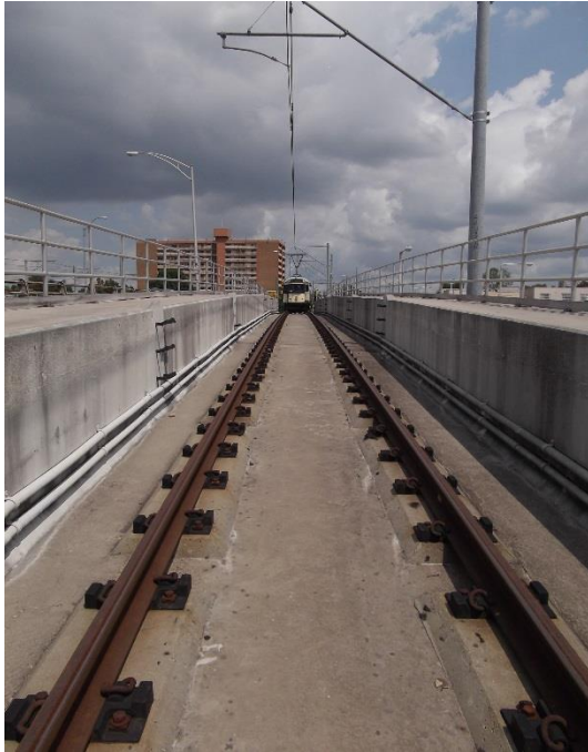
Figure 16 – Showing the limited clearance and the 6% grade over the Danny Thomas Blvd. Bridge on the Madison Avenue Line
