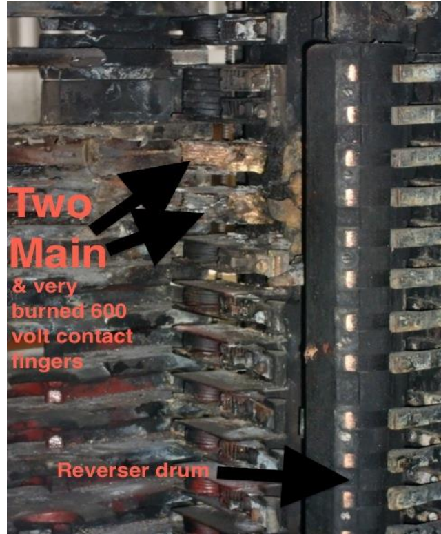
Figure 10 – Reverser drum on trolley #452 after the fire,
