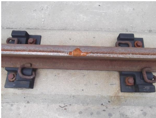
Figure 17 – Rail burn marks on the Danny Thomas Blvd. Bridge on the Madison Avenue
