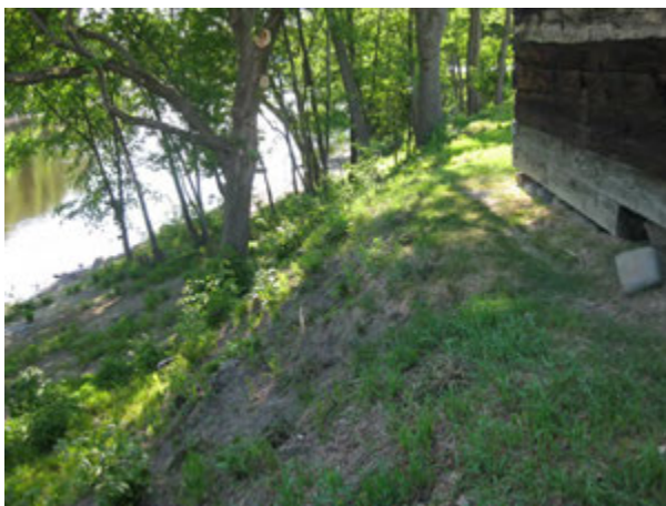
View of the eroding slope behind the Block House. The slope should be stabilized to stop erosion, improve riparian habitat, and protect the historic resources.
